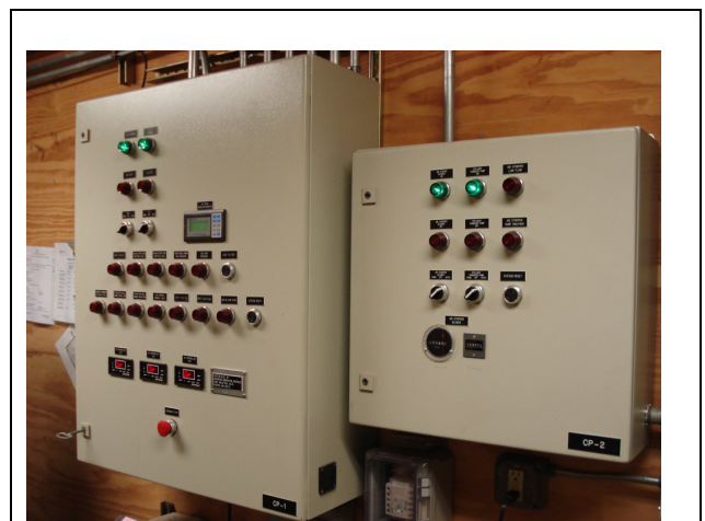
Photo 6. Control panels in GWTS unit.
