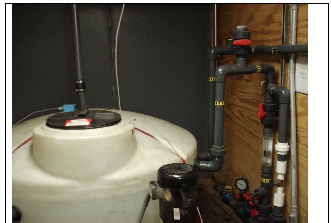
Photo 4. Equalization tank inside GWTS unit.
