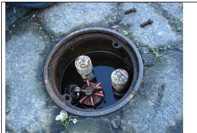
Photo 11. MW-8, inside flush mount cover.
