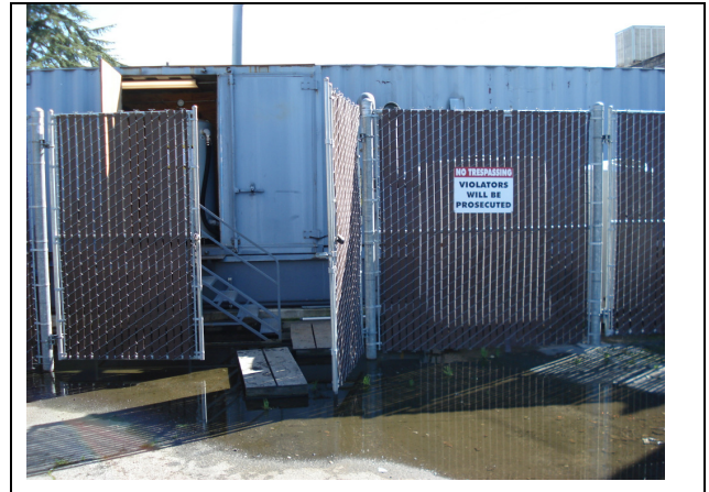
Photo 2. Security fence surrounding treatment systems.
