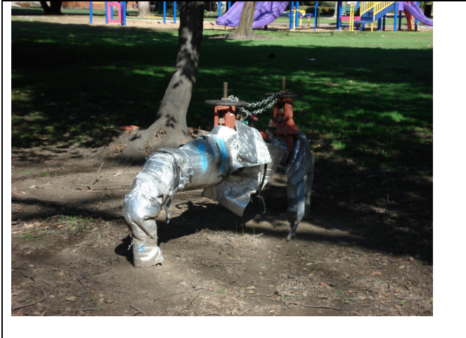
Photo 13. Municipal Well 12 (not in operation).
