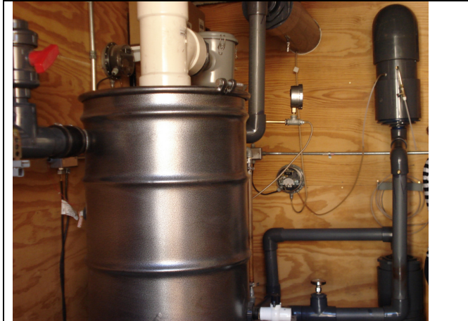
Photo 7. GAC treatment inside SVE unit.
