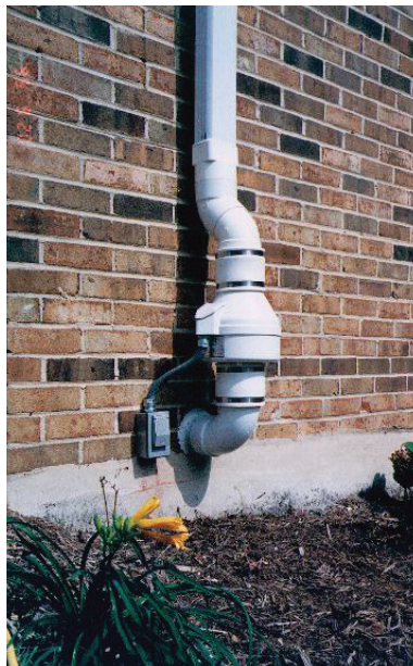
Typical fan and vent pipe.
