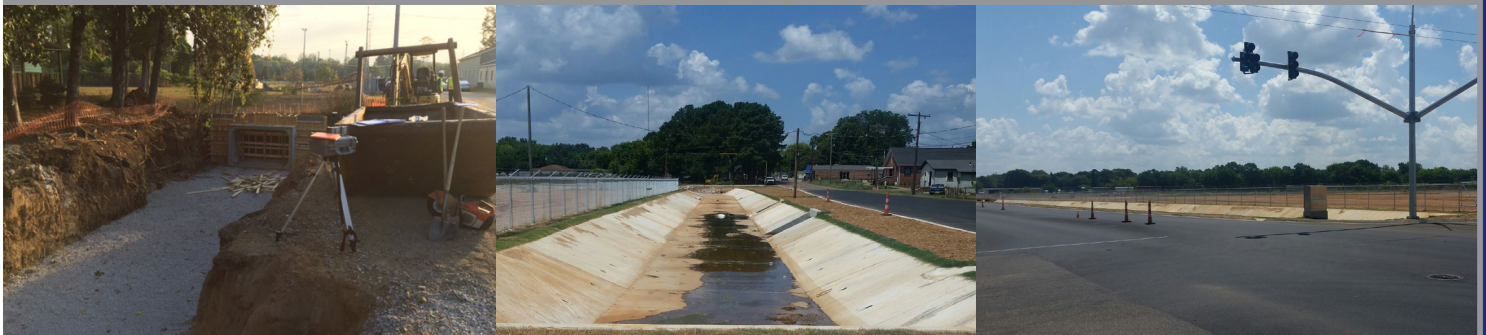
Images from left to right: October 2016 cleanup of 7th Avenue ditch, installation of new 14th Avenue ditch and completed, paved intersection.
