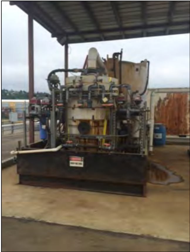
Photo 6. Groundwater treatment plant.
