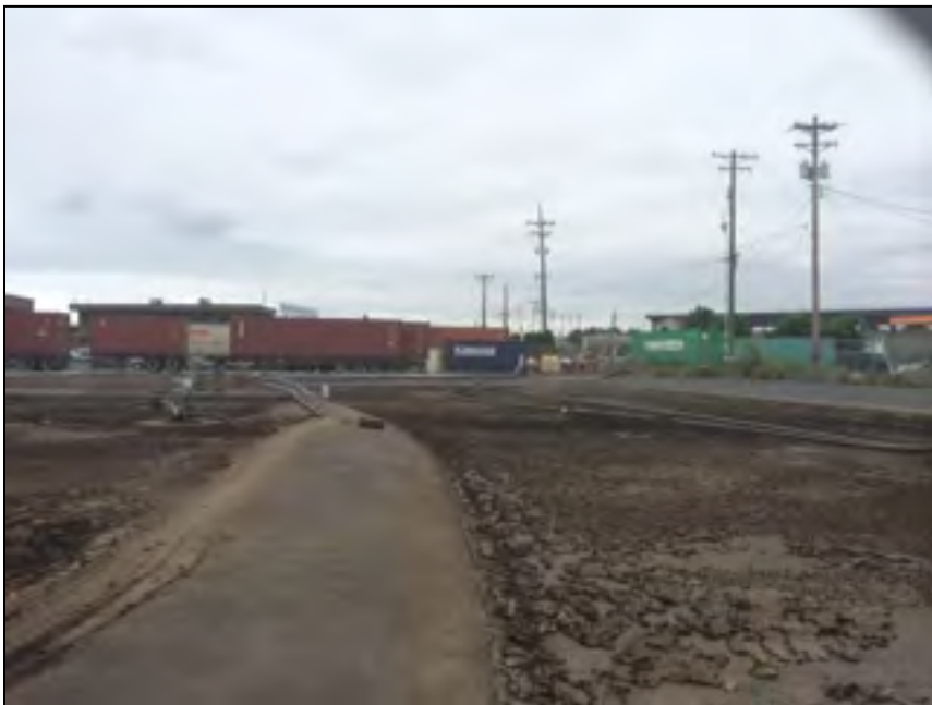
Photo 2. Sedimentation in Detention Basin 2.
