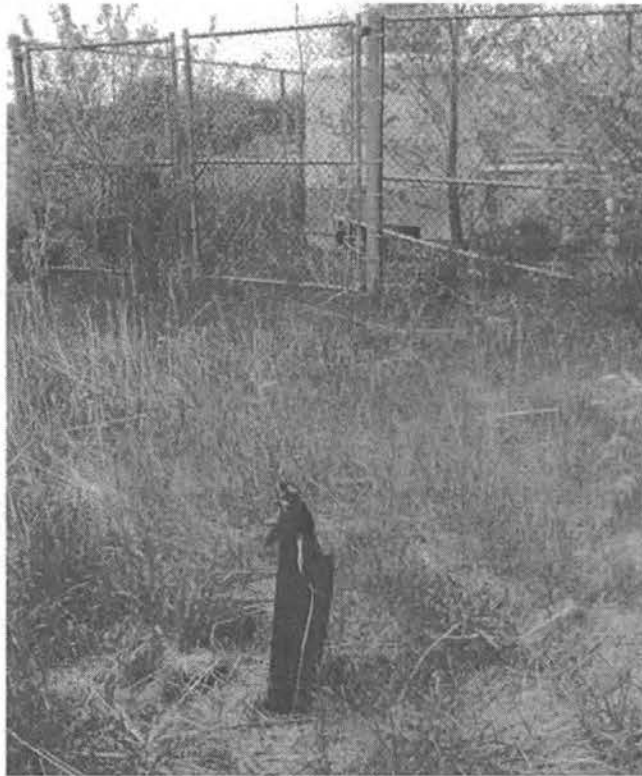
Picture 4 – Damaged Monitoring Well G120
