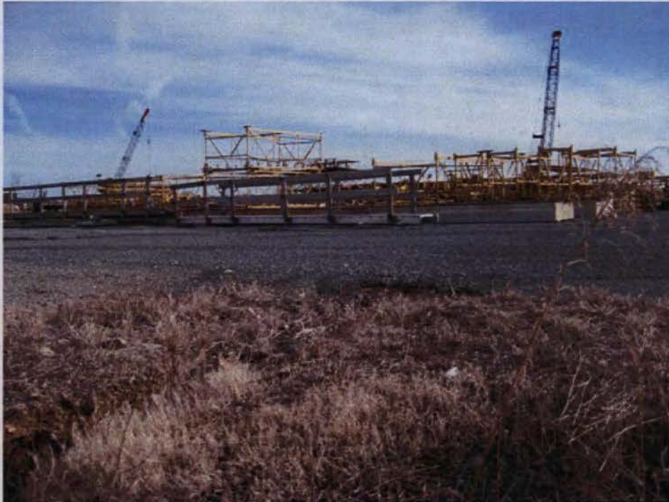
Graveled storage area extended beyond cap with equipment storage.
