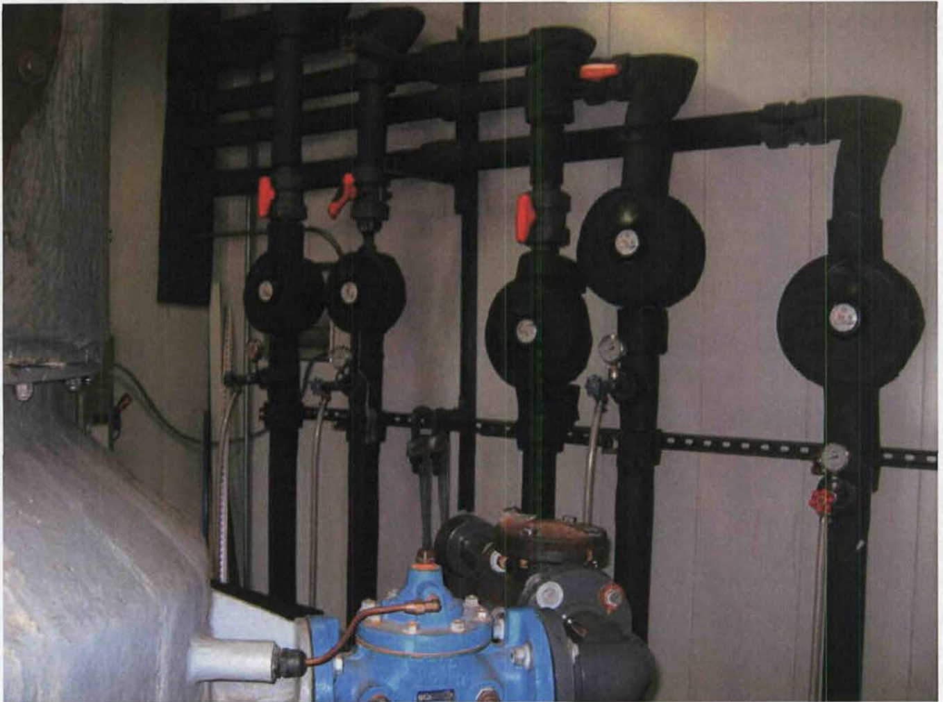
Extraction Pump Lines 1-4
