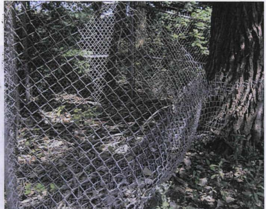
Photo 12: View of more vandalism to a large area of the RSQ Site perimeter fence.
