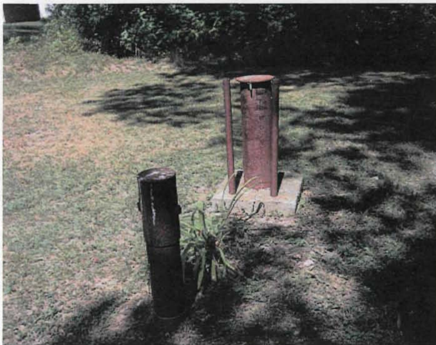
Photo 17: A view looking eastward toward MW B-2 located in the backyard of a resident of the New Riverbend Homes subdivision along West River Road. The residential lot is immediately adjacent to the RSQ Site northern property line. MW B-2 is representative of the condition of the other MWs.
