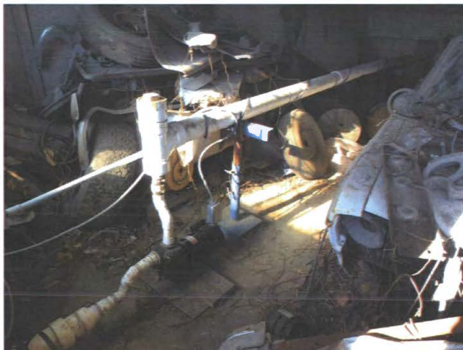
Recovery pump, located in a garage at McKinney's Towing.
