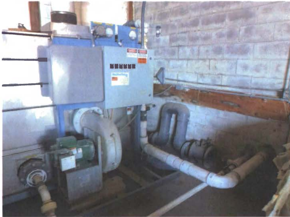
Air stripper, located in a garage at Harris Towing.
