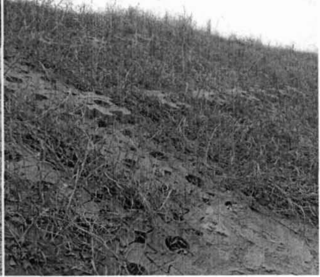
Photo 28. Looking west at ACB from the eastern edge. Note the raised concrete blocks.
