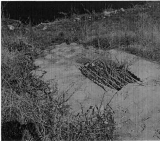
Photo 31. Clogged CMP outfall in stabilized Leon River bank.
