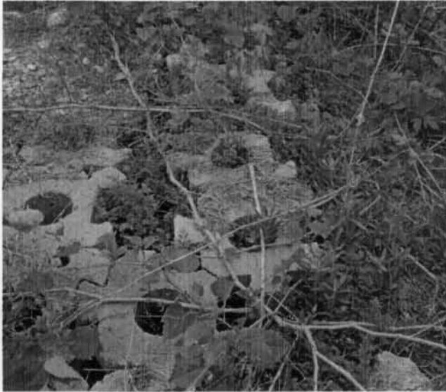
Photo 39. Instability and loss of continuity in the ACB at the toe of the LRB.
