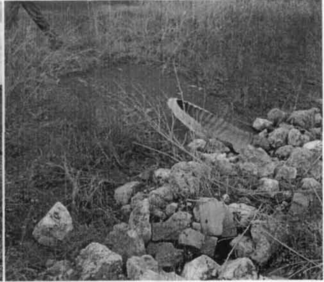
Photo 71. Detention basin outlet pipe.
