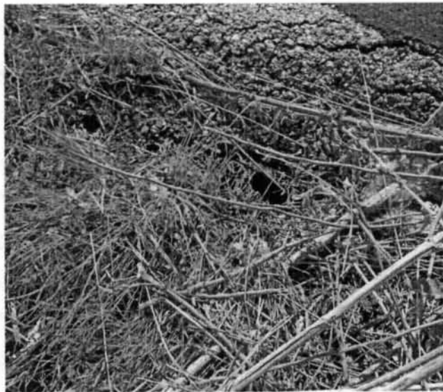
Photo 68. Possible minor erosion at the southern edge of the CC cap.
