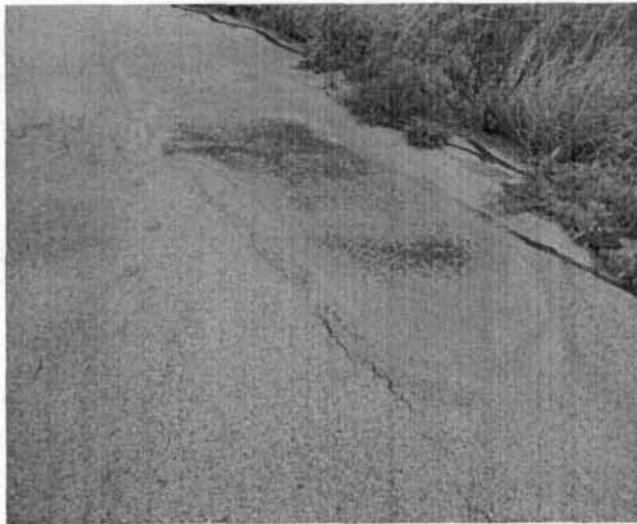
Photo 60. Area where water stands near the edge.
