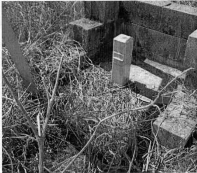
Photo 15. MW-25-90, identification marker has fallen off
