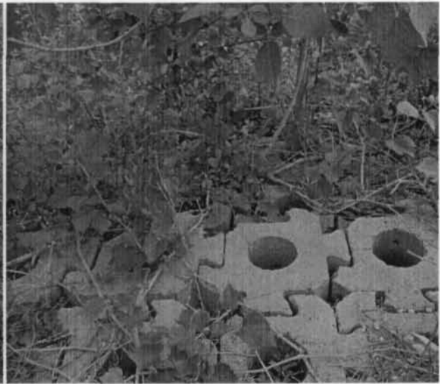
Photo 42. Instability and loss of continuity in the ACB at the toe of the LRB.
