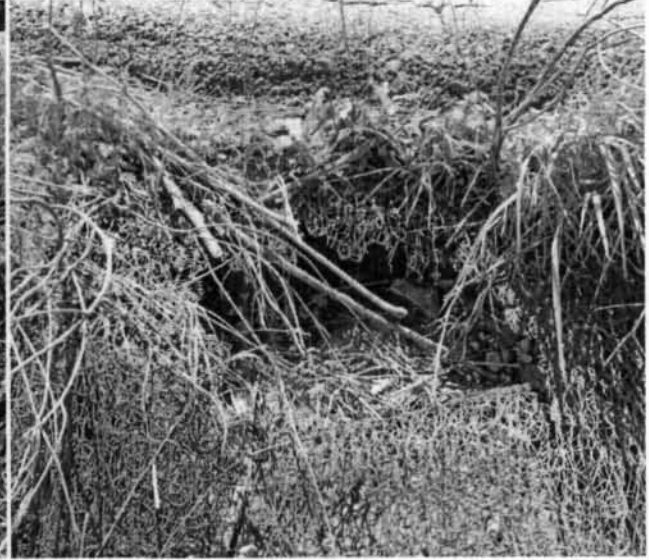
Photo 67. Possible minor erosion at the northern edge of the CC cap.
