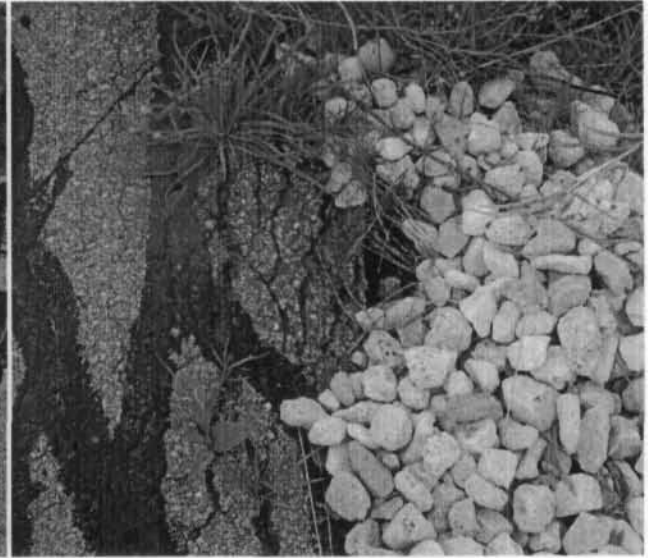
Photo 63. Rip rap along the southern edge of the CC. The hole in the rip rap indicates that erosion may still be occurring.
