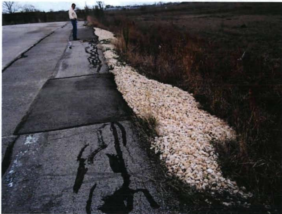
Repaired erosion damage to the Matcon cap, March 17, 2011 photograph.
