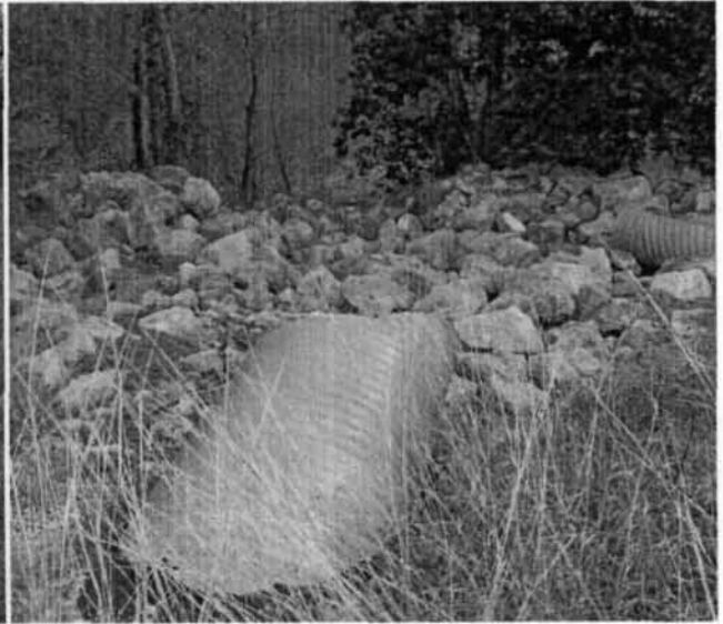
Photo 54. CMP outfalls at the northern edge of the CSP.
