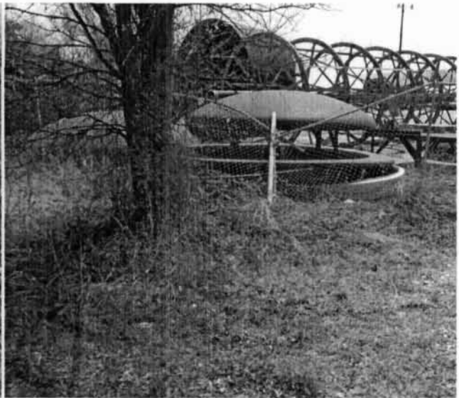
Photo 46. Damaged fence at the northwest corner of the paved parking area.
