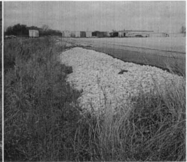
Photo 65. Rip rap and repaired cap along the southern edge of the CC.
