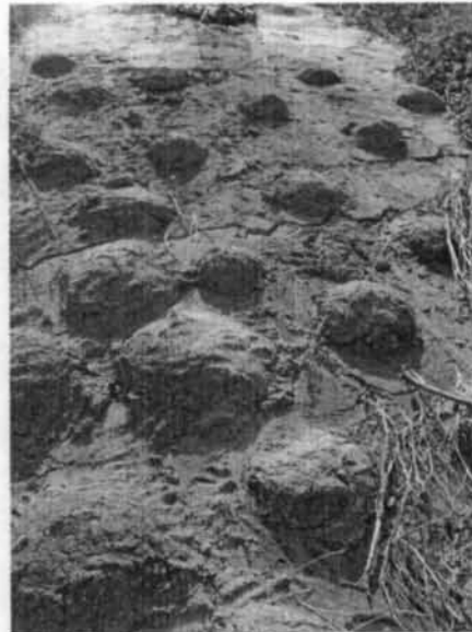
Photo 34. Crack in concrete CMP outfall.
