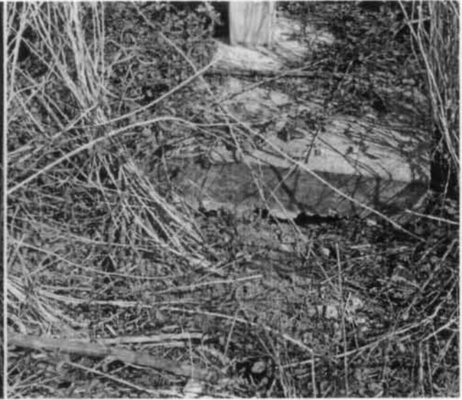
Photo 18. MW-28-90, soil has eroded out beneath the well pad.
