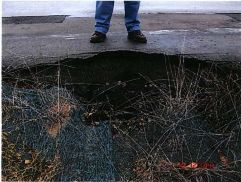
Undated photograph of erosion damage to the Matcon cap.
