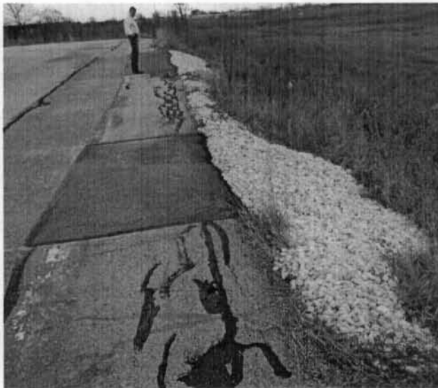
Photo 64. Rip rap and repaired cap along the southern edge of the CC.
