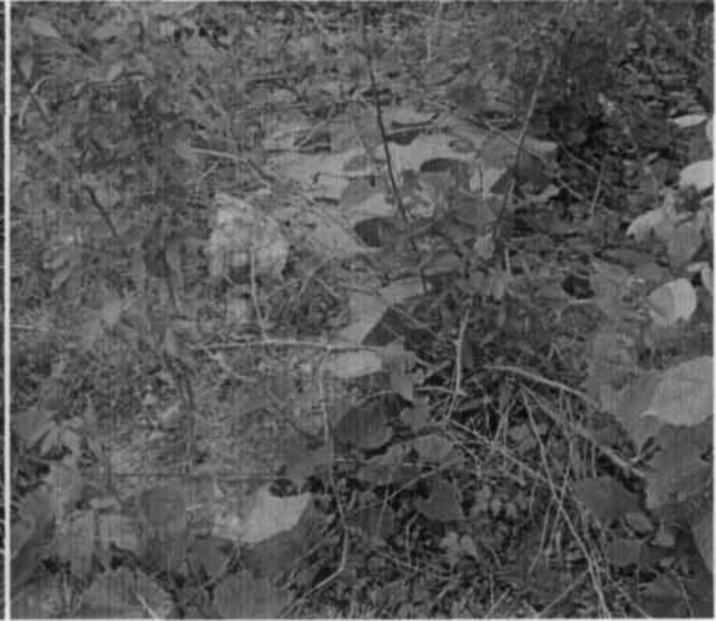
Photo 40. Instability and loss of continuity in the ACB at the toe of the LRB.
