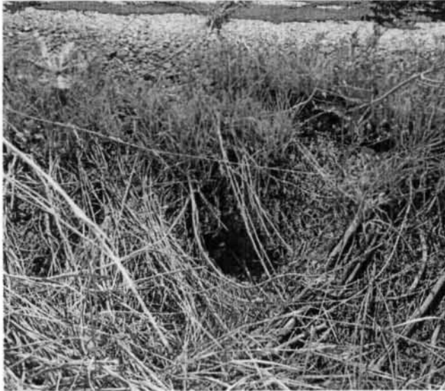
Photo 66. Possible minor erosion at the northern edge of the CC cap.
