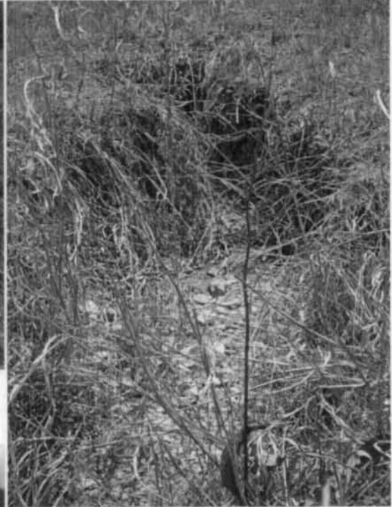
Photo 48. Erosion in EVL area about 25 feet west of well MW-35-90.
