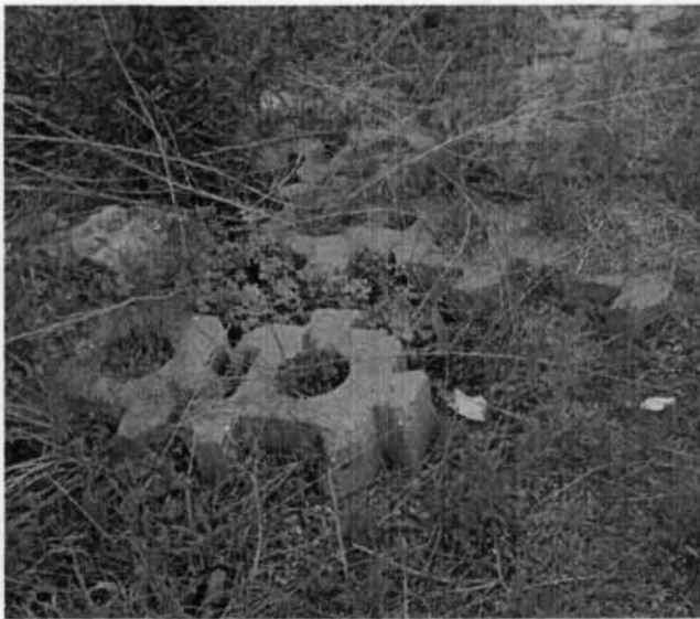
Photo 41. Instability and loss of continuity in the ACB at the toe of the LRB.
