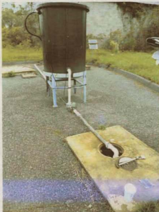
Flushing system for F&G ground water remedy at OUI.
