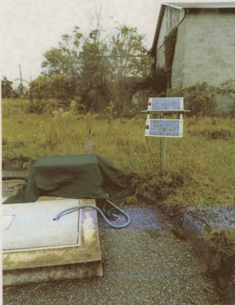
Solar panels used as part of the F&G system.
