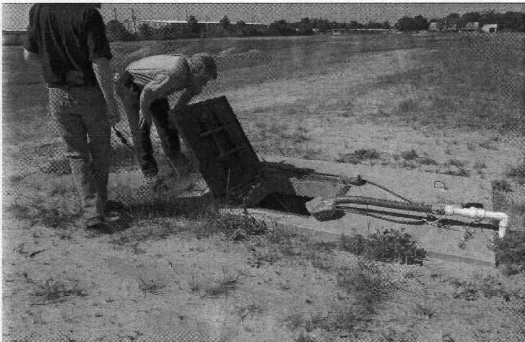
Leachate collection system located on the southeast corner of the soil containment cell
