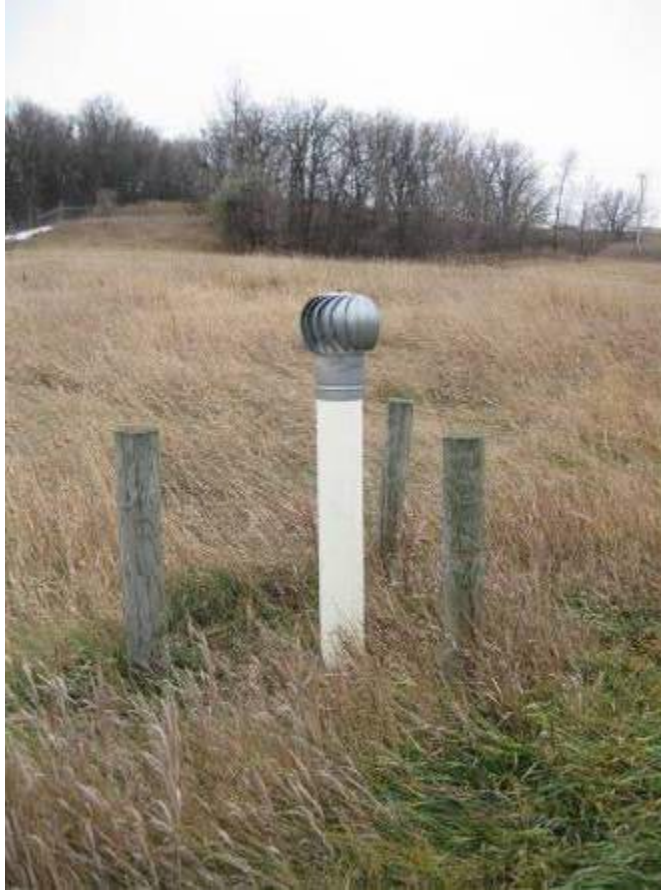
Passive landfill gas vent
