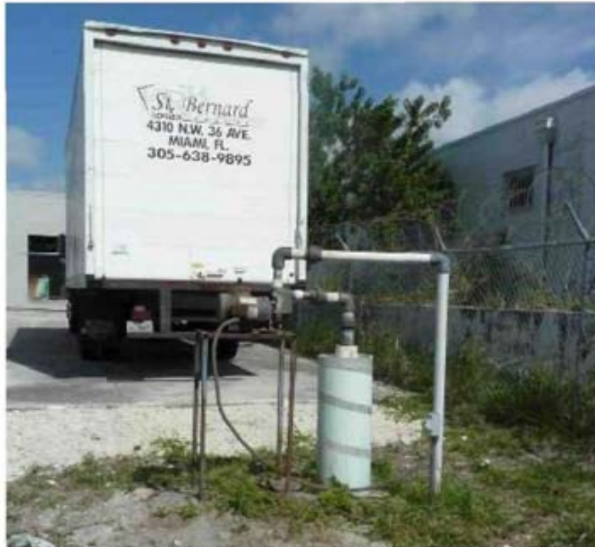
Recovery well (RW-1) and company truck parked on cap.
