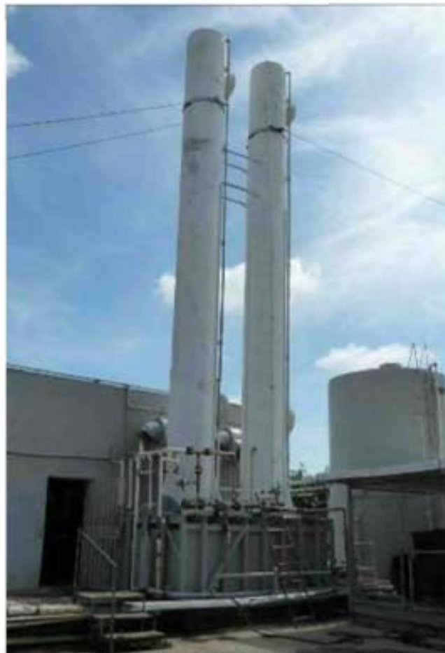
Air strippers at the Airco Plating Co. facility.
