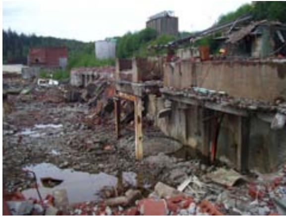
Photo 9. View northwest of demolished buildings where scrap metal has been removed for sale
