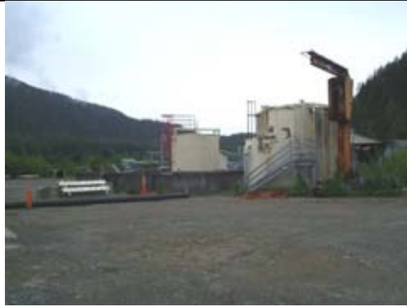
Photo 38. Aboveground storage tanks
