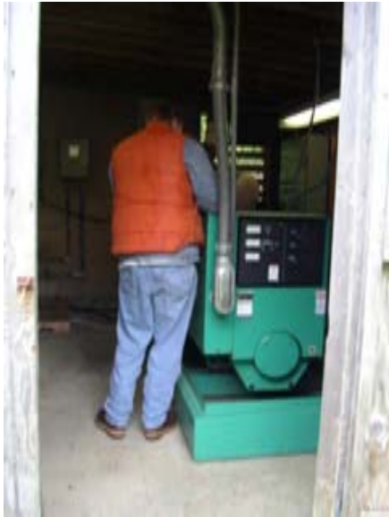
Photo 51. Generator for landfill
