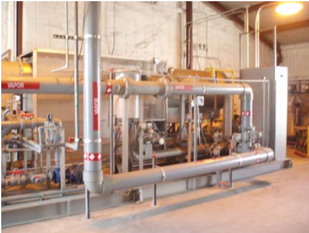
Photo 8: Flame Thermal Oxidizer view 2. May, 27 2010
