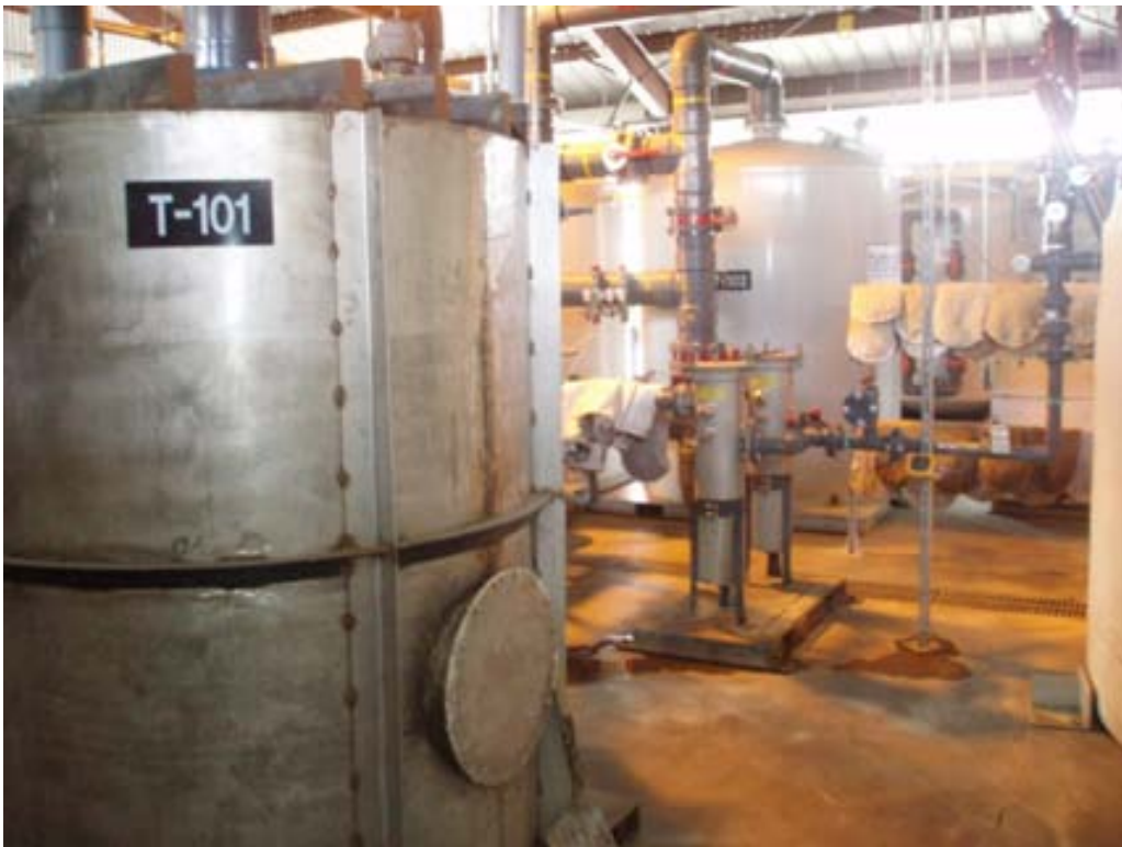
Photo 2: Knockout tank T-101 in foreground with Carbon tanks T-302 in background. May 27, 2010.
