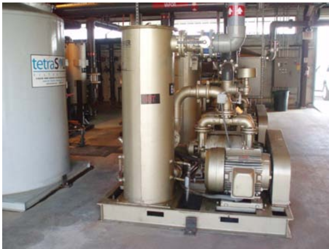
Photo 6: Vacuum blowers. May 27, 2010
