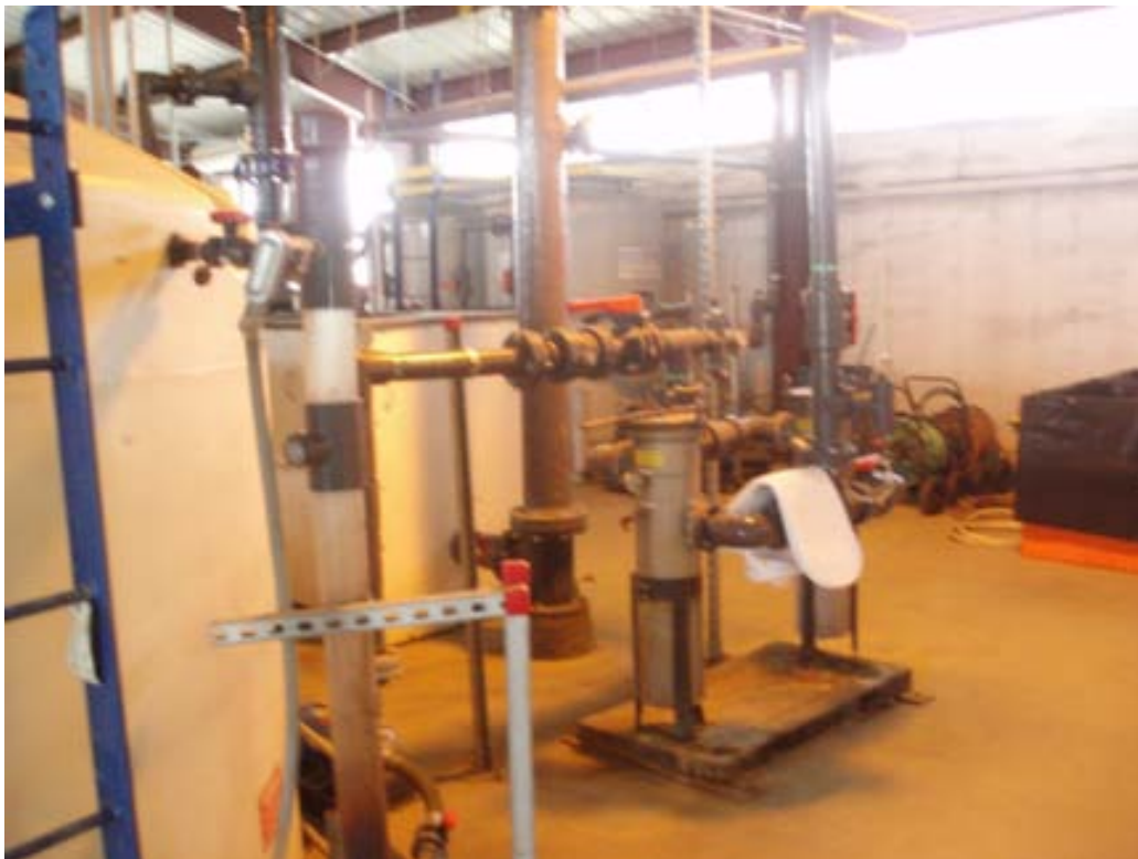
Photo 4: SP-204 and clean filter bag ready to be inserted into filter bag housing. May 27, 2010.
