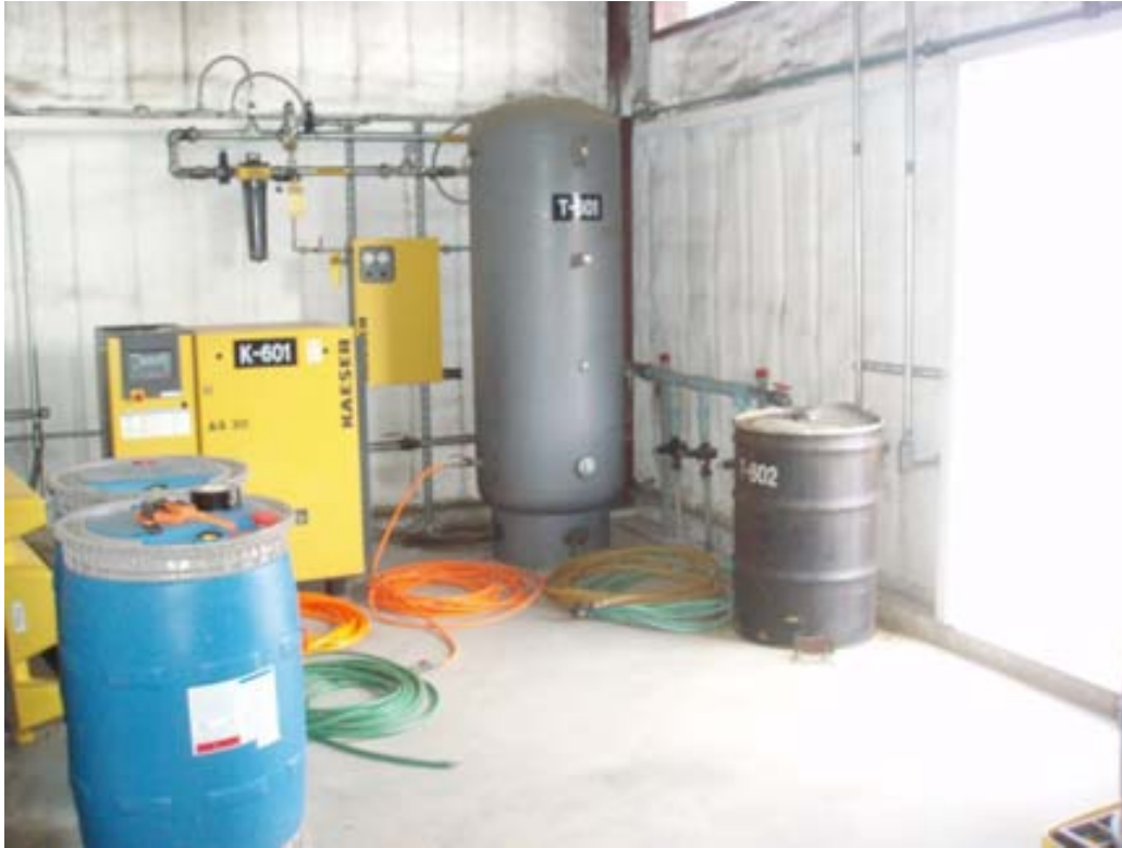
Photo 3: Compressed air tank. T-601. May 27, 2010
