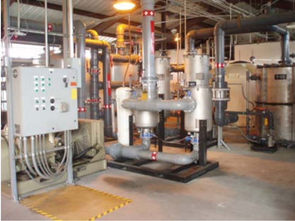
Photo 9: SP-104 and blower control panel. May 27, 2010
