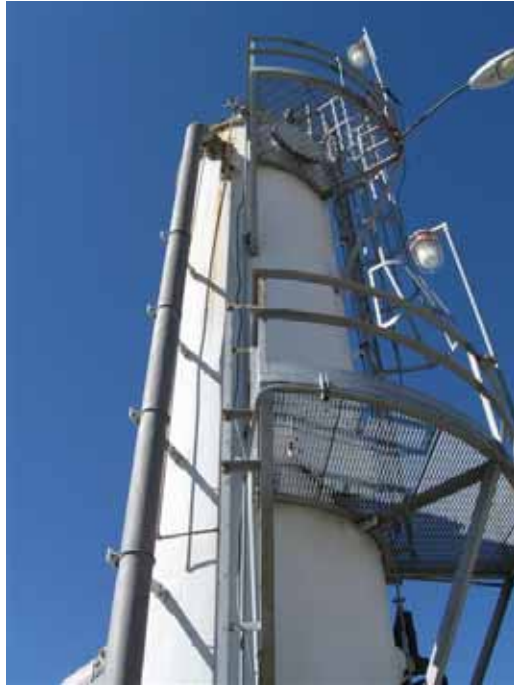
Photo 16. PGAS Site Visit. Subunit A airstripper tower.
