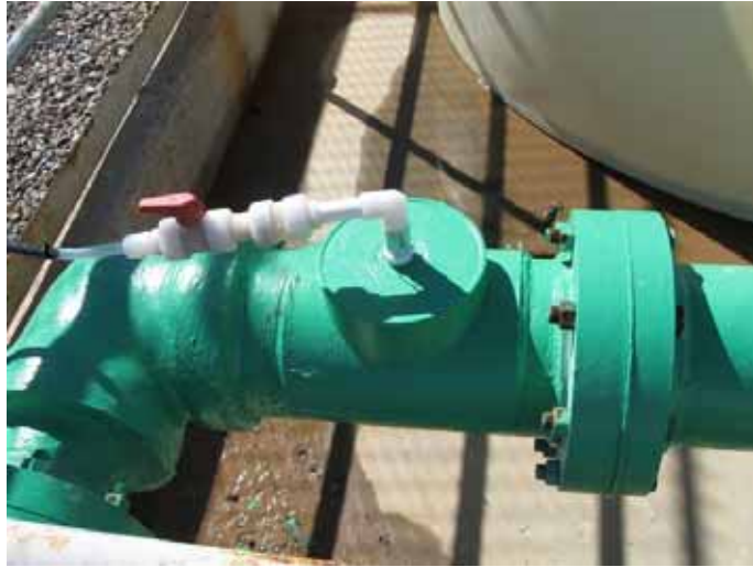
Photo 14. PGAS Site Visit. Influent anti-scaling injection location.
