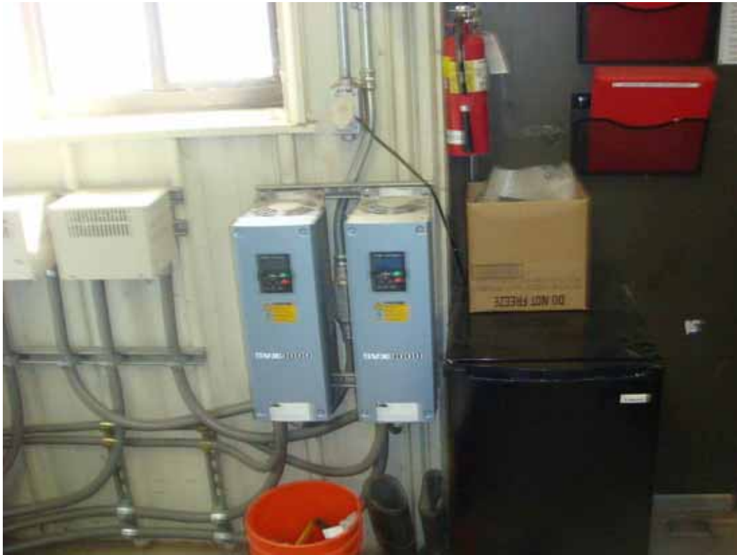
Photo 5. PGAS Site Visit. Variable Frequency Drives operating process water (injection) pumps, Southern Subunit A.
