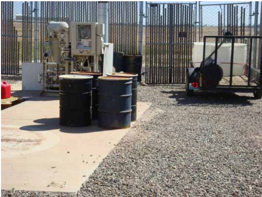
Photo 27. PGAS Site Visit. Subunit A treatment compound showing unmarked drums and decommissioned SVE system.
