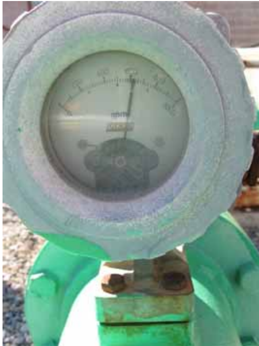
Photo 4. PGAS Site Visit. Subunit A influent flow meter.
