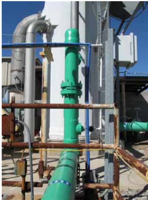
Photo 15. PGAS Site Visit. Subunit A extraction piping and airstripper.
