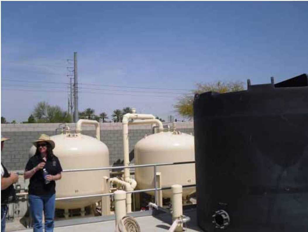
Photo 6. PGAN Site Visit. Liquid phase carbon vessels at EA-06.
