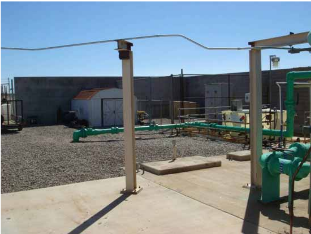
Photo 13. PGAS Site Visit. Subunit A treatment compound showing inlet piping and anti-scalant storage.
