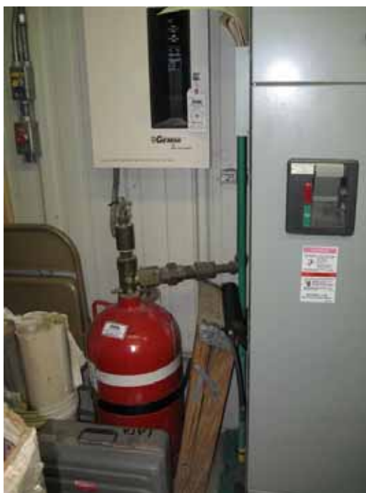
Photo 22. PGAS Site Visit. Subunit A control room.
