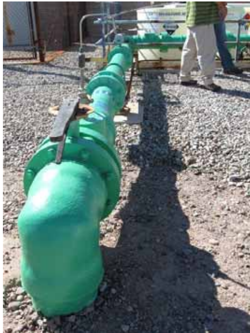
Photo 2. PGAS Site Visit. Subunit A influent piping showing manual shutoff valve and sample port.
