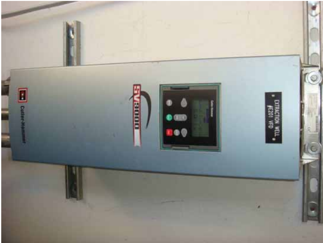
Photo 36. PGAS Site Visit. Variable Frequency Drive for Subunit C extraction well (E-201).
