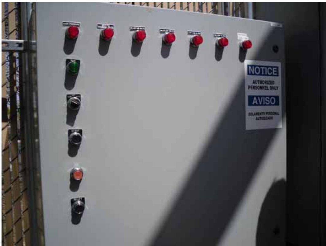
Photo 4. PGAN Site Visit. EA-05 control panel.
