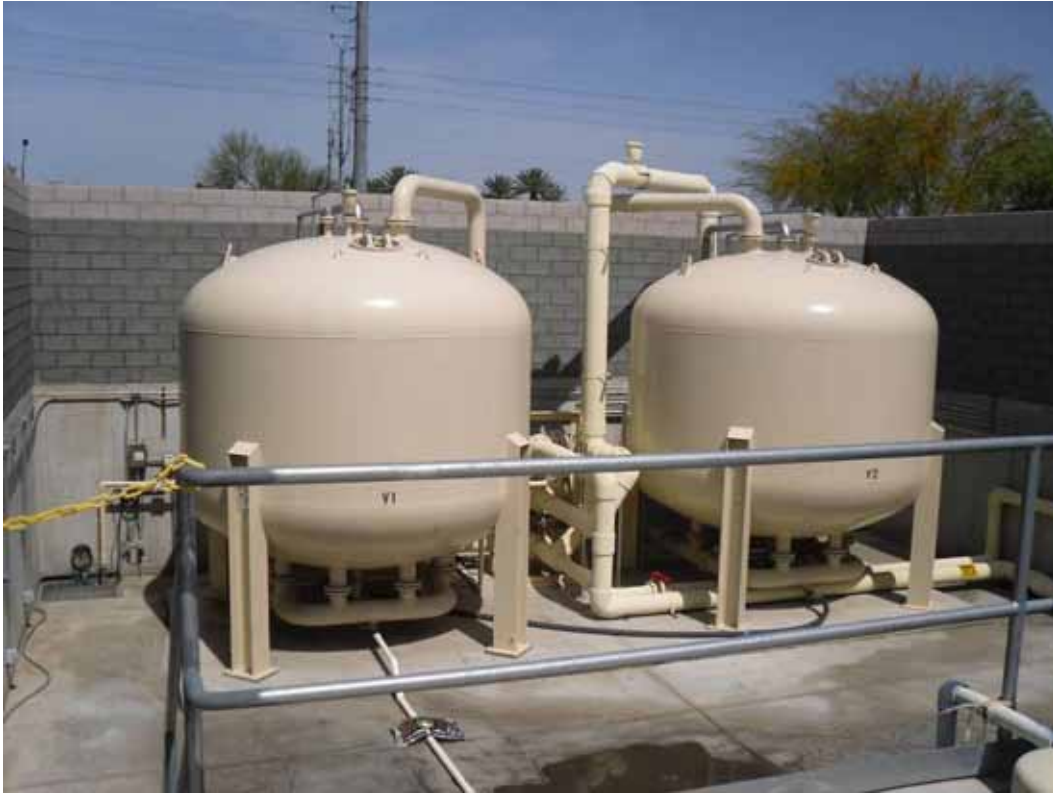
Photo 7. PGAN Site Visit. Liquid phase carbon vessels at EA-06.
