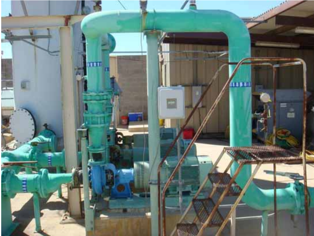
Photo 26. PGAS Site Visit. Piping from Subunit A airstripper to injection wells showing process pumps and motors.
