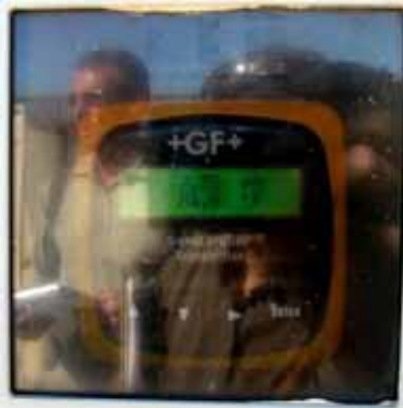
Photo 17. PGAS Site Visit. Subunit A differential pressure switch.
