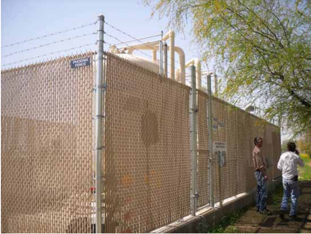
Photo 5. PGAN Site Visit. EA-05 treatment system compound.
