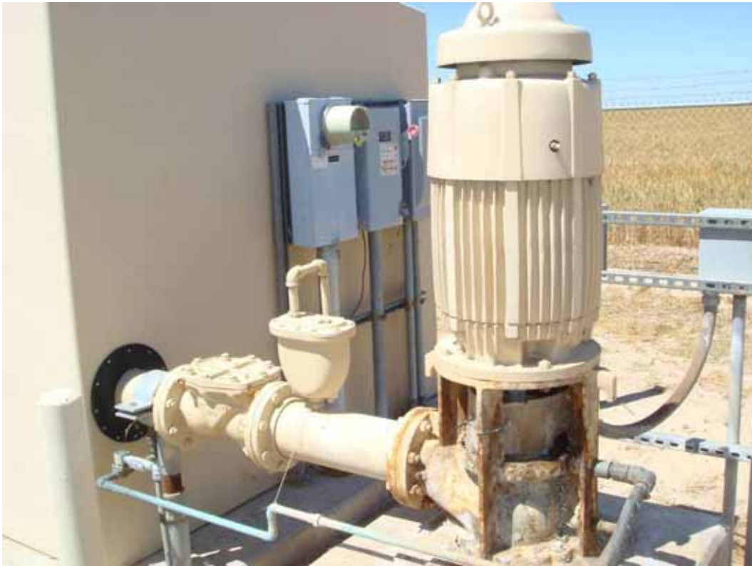
Photo 45. PGAS Site Visit. Extraction pump for well E-102.
