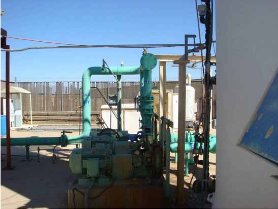
Photo 7. PGAS Site Visit. Piping from Subunit A airstripper to injection wells.
