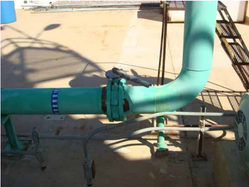
Photo 8. PGAS Site Visit. Piping from Subunit A airstripper to injection wells showing manual shutoff valve.
