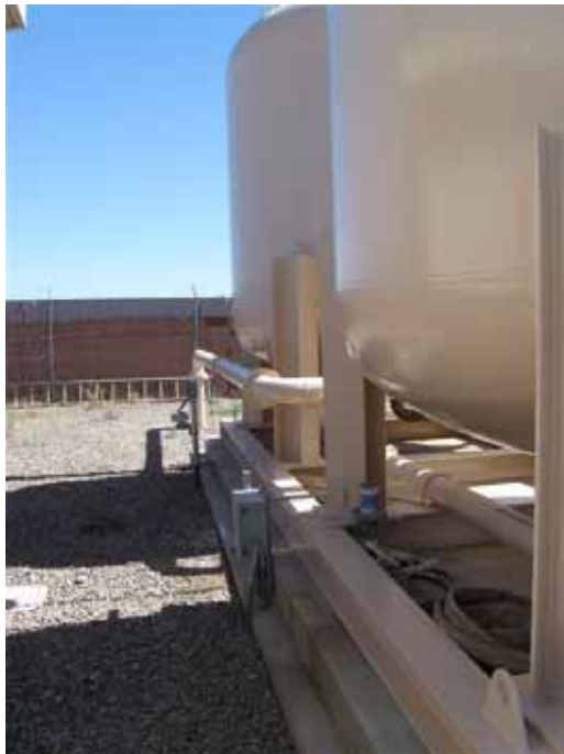
Photo 35. PGAS Site Visit. Subunit C treatment system effluent piping.
