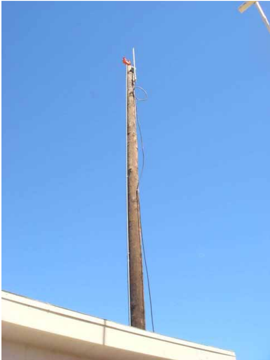
Photo 38. PGAS Site Visit. Radio telemetry device at Subunit C treatment compound.
