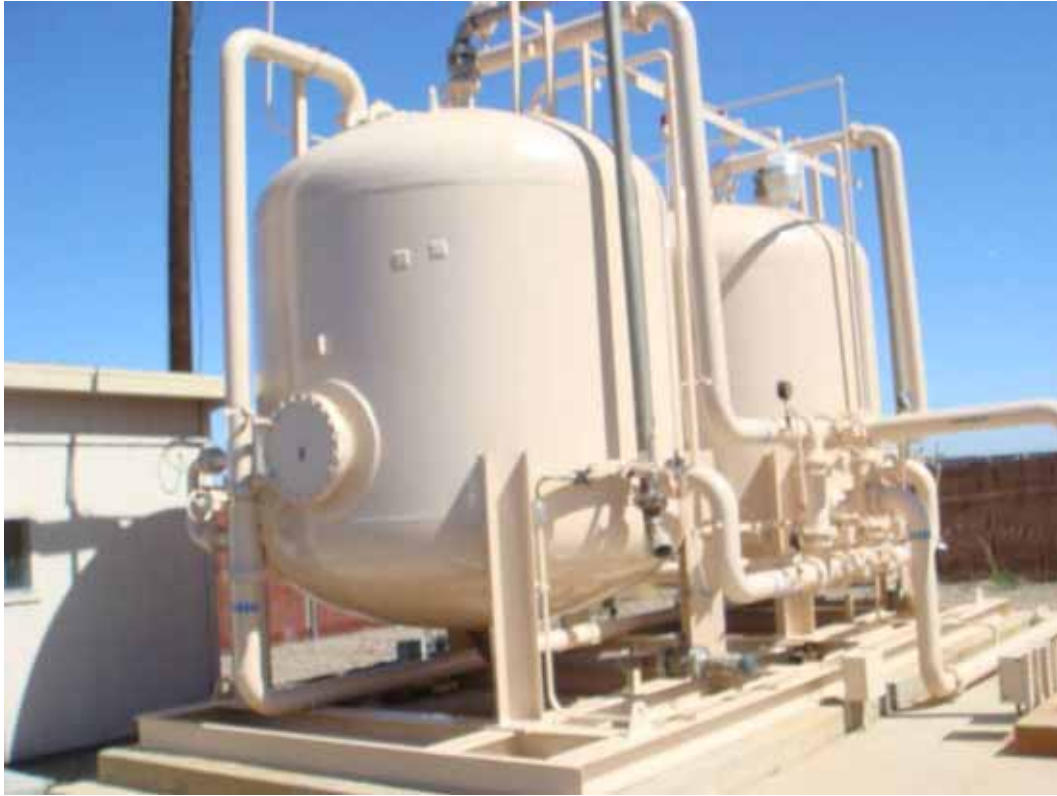
Photo 32. PGAS Site Visit. Subunit C liquid phase carbon vessels.
