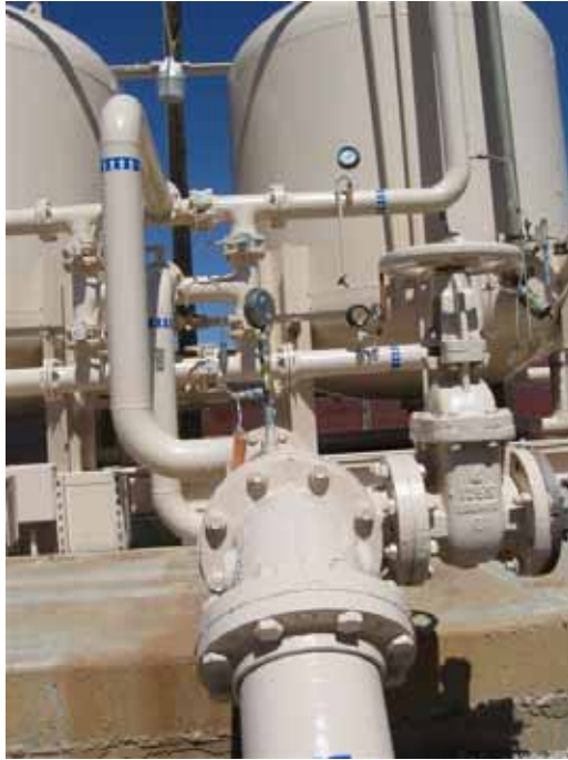
Photo 34. PGAS Site Visit. Subunit C influent piping into liquid phase carbon vessels.
