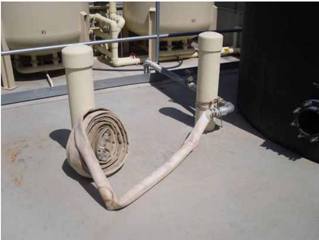
Photo 8. PGAN Site Visit. Tie-in for Maricopa County Flood Control District access to treated effluent at EA-06.
