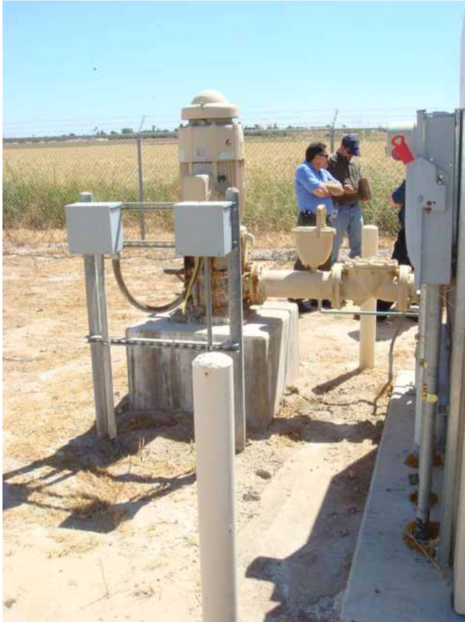
Photo 42. PGAS Site Visit. Extraction pump for well E-102.
