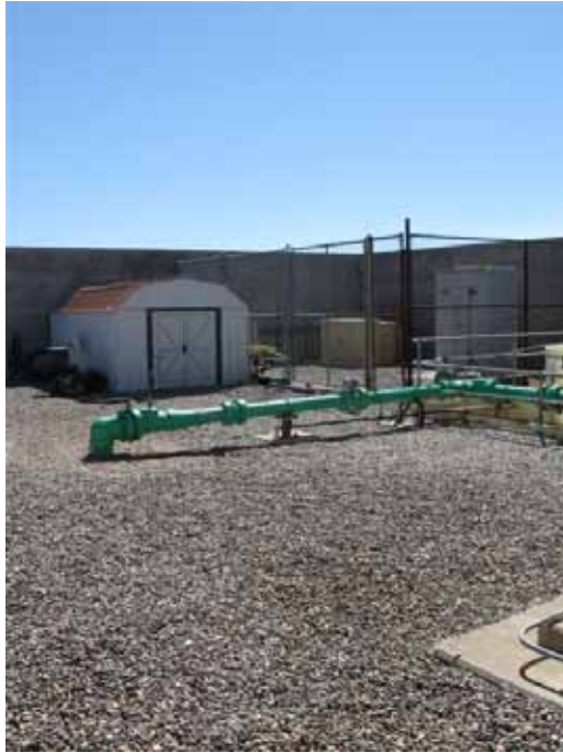
Photo 3. PGAS Site Visit. Subunit A influent piping showing manual shutoff valve and sample port.
