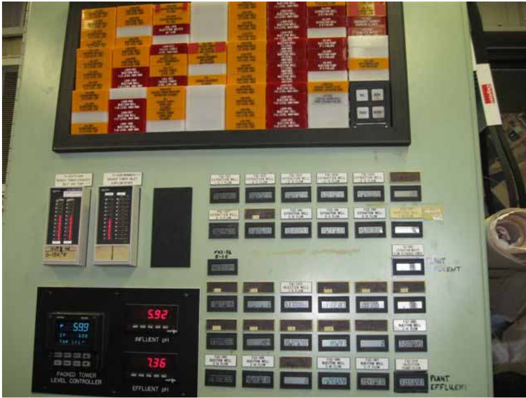
Photo 20. PGAS Site Visit. Control Panel for Subunit A extraction and treatment system.
