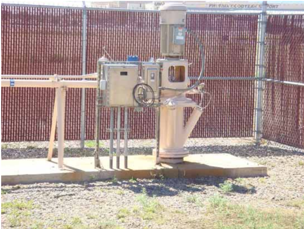
Photo 33. PGAS Site Visit. Subunit C extraction wellhead.
