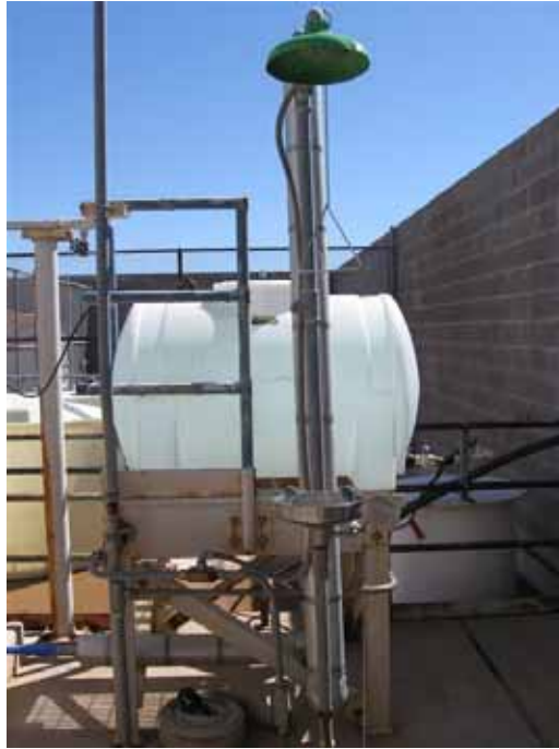
Photo 28. PGAS Site Visit. Subunit A treatment compound eyewash station.
