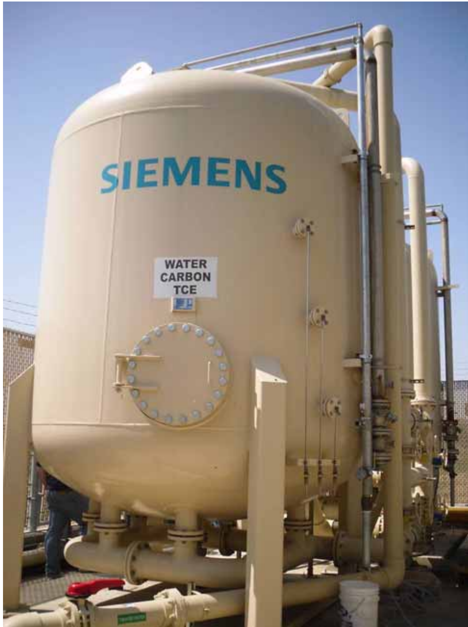
Photo 2. PGAN Site Visit. Liquid phase carbon vessel at EA-05.
