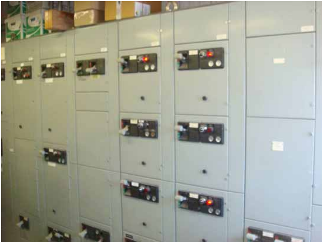
Photo 6. PGAS Site Visit. Motor Control Center for Southern Subunit A.
