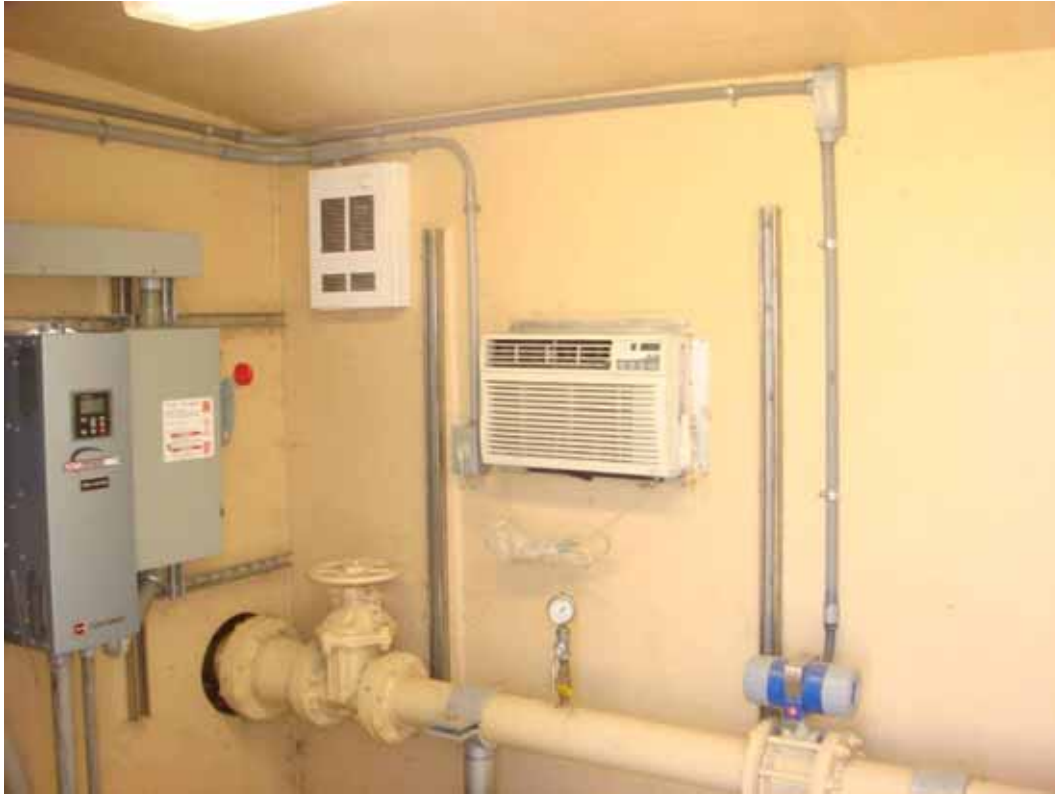
Photo 39. PGAS Site Visit. Extraction and treatment control building at Subunit C showing VFD, shutoff valve, and flow totalizer.
