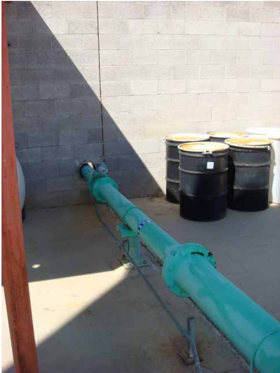
Photo 9. PGAS Site Visit. Piping from Subunit A airstripper to injection wells penetrating compound wall.
