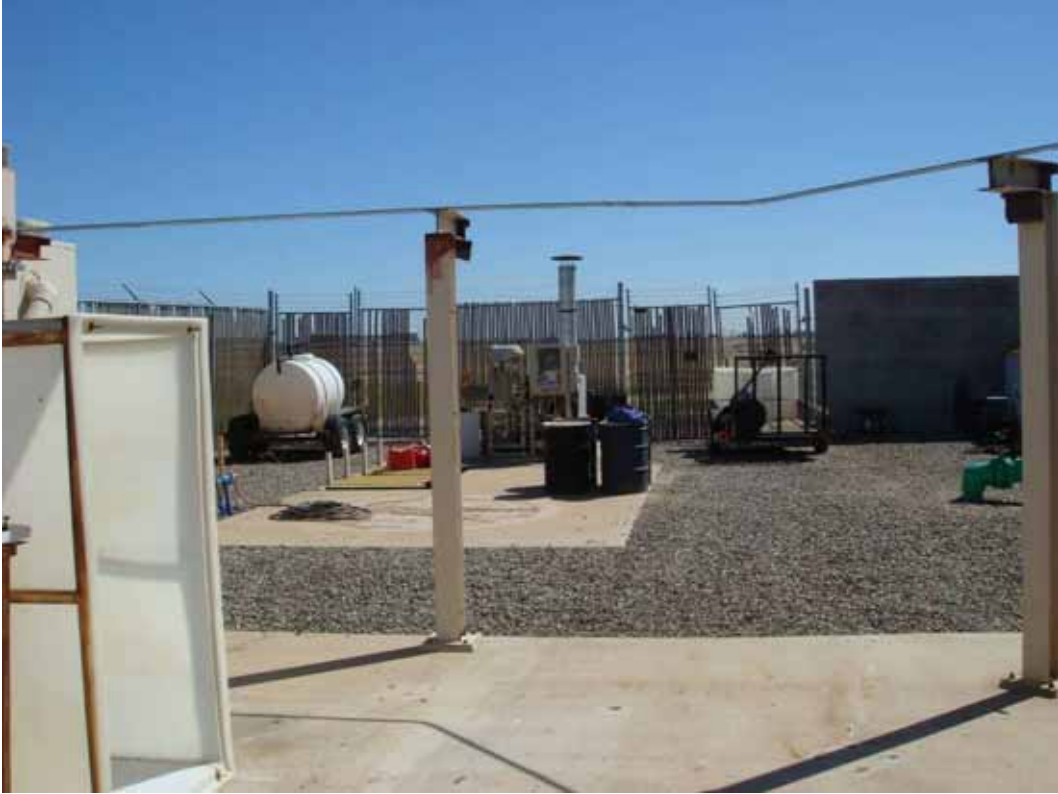
Photo 12. PGAS Site Visit. Subunit A treatment compound.
