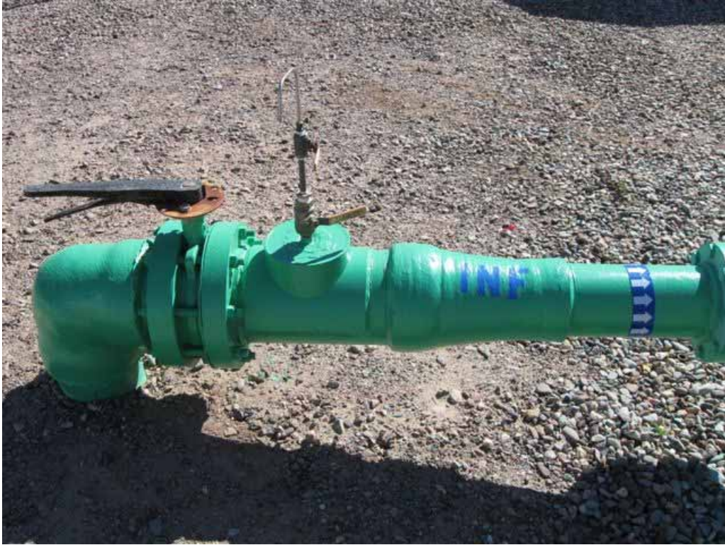
Photo 1. PGAS Site Visit. Subunit A influent piping showing manual shutoff valve and sample port.
