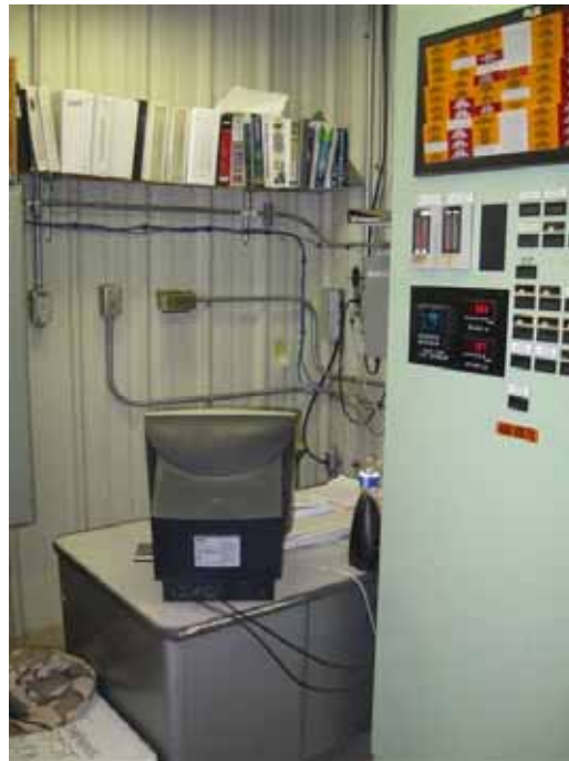
Photo 21. PGAS Site Visit. Subunit A control room.
