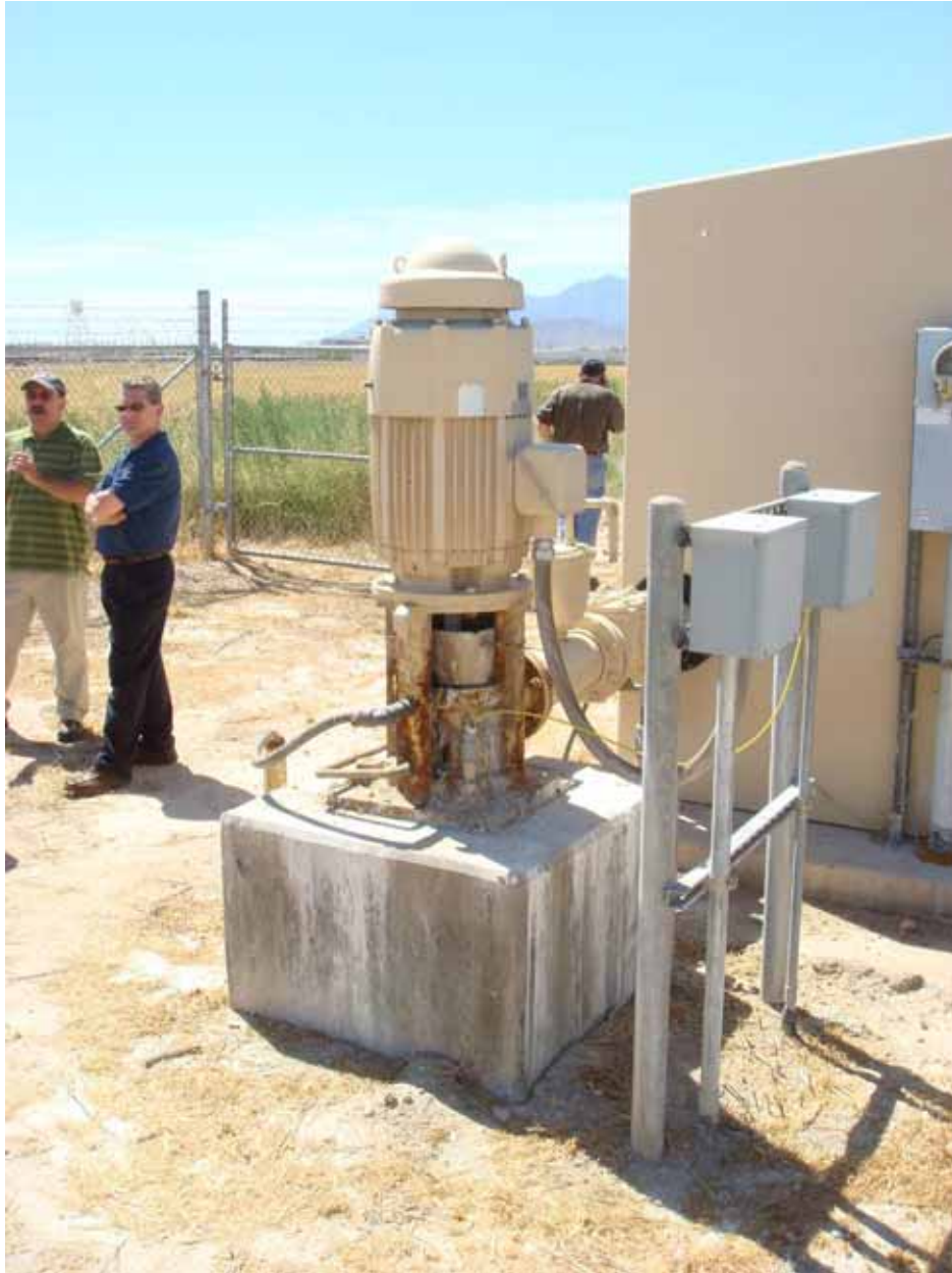
Photo 44. PGAS Site Visit. Extraction pump for well E-102.
