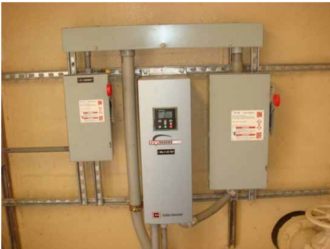
Photo 40. PGAS Site Visit. Variable Frequency Drive for extraction well E-102.
