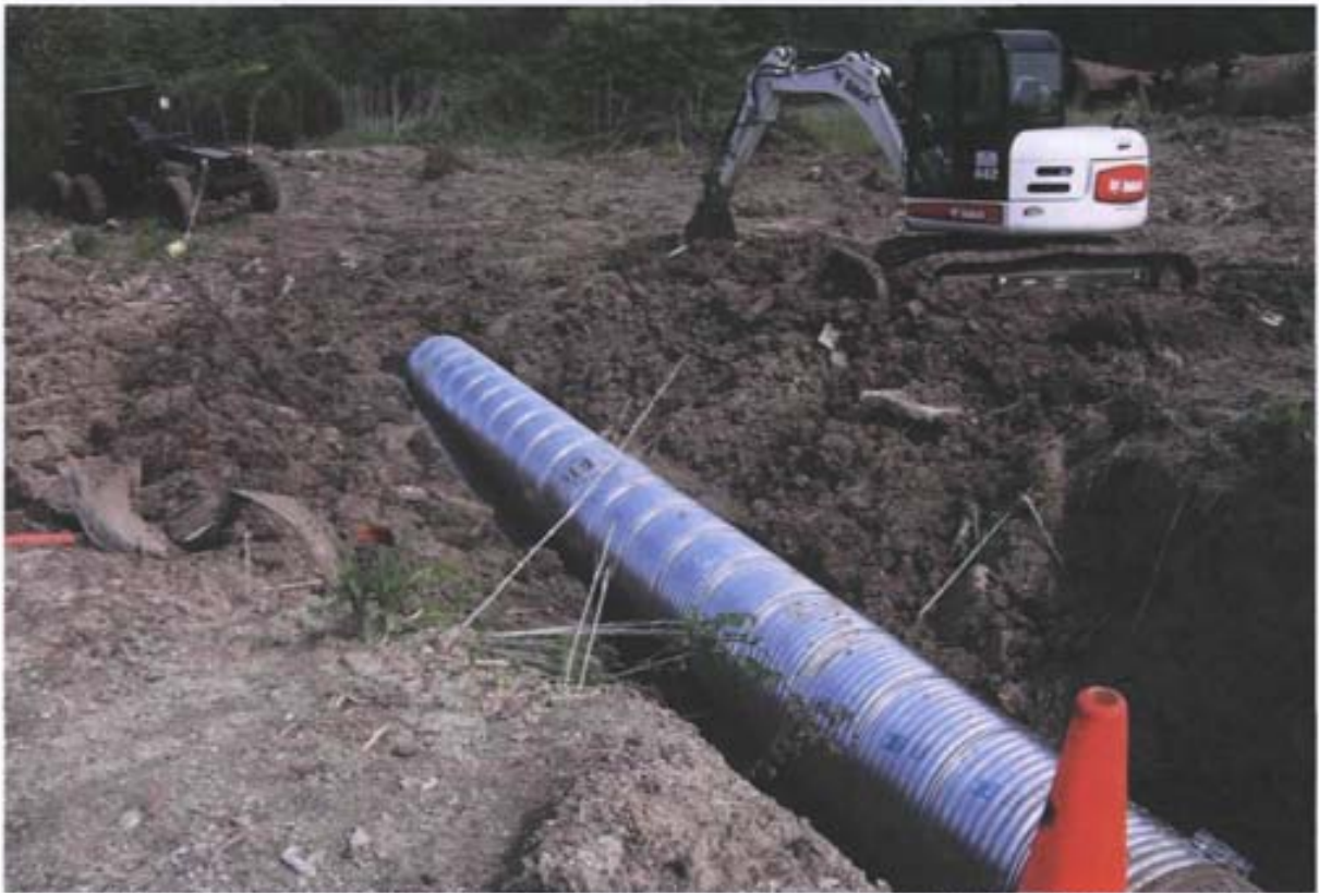
Photo 52: Northwest view of 20 by 80 by 10-foot disturbed area during culvert replacement at Site LF-42.
