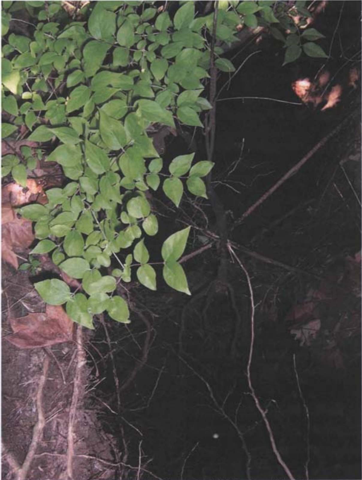
Photo 40: Close-up of 20 by 4-foot erosion feature near north IC boundary at Site LF-34.
