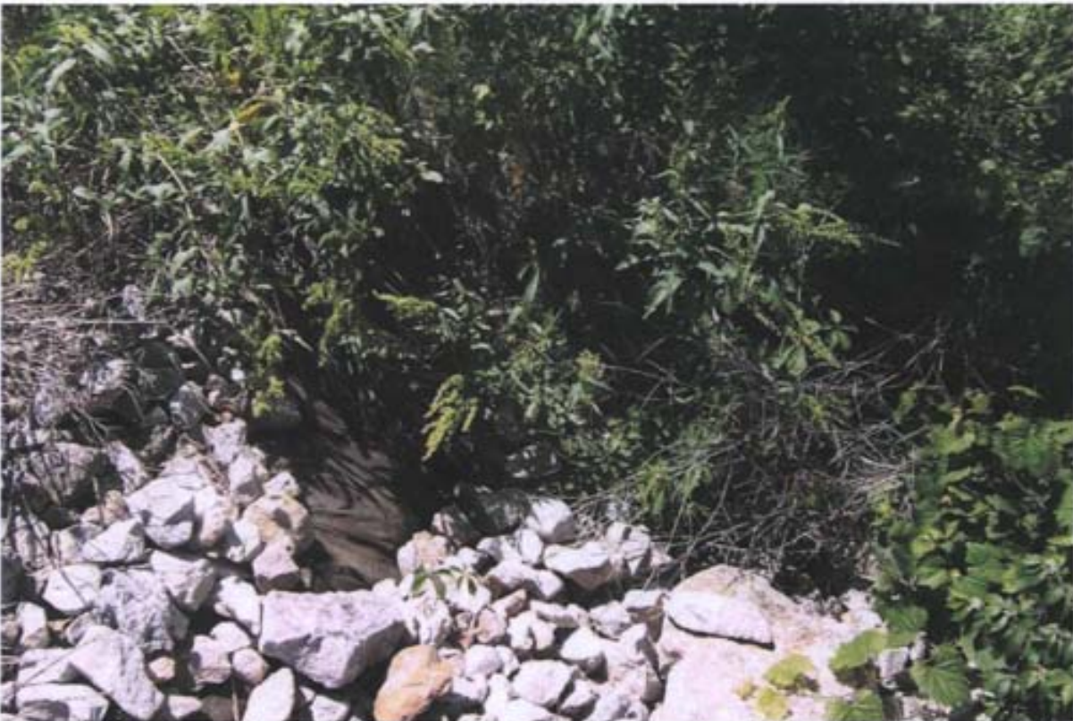
Photo 12: Close-up of 7 by 15 by 3-foot erosion feature along southern bank of Lower Branch Creek at Sites LF-03/SS-41.
