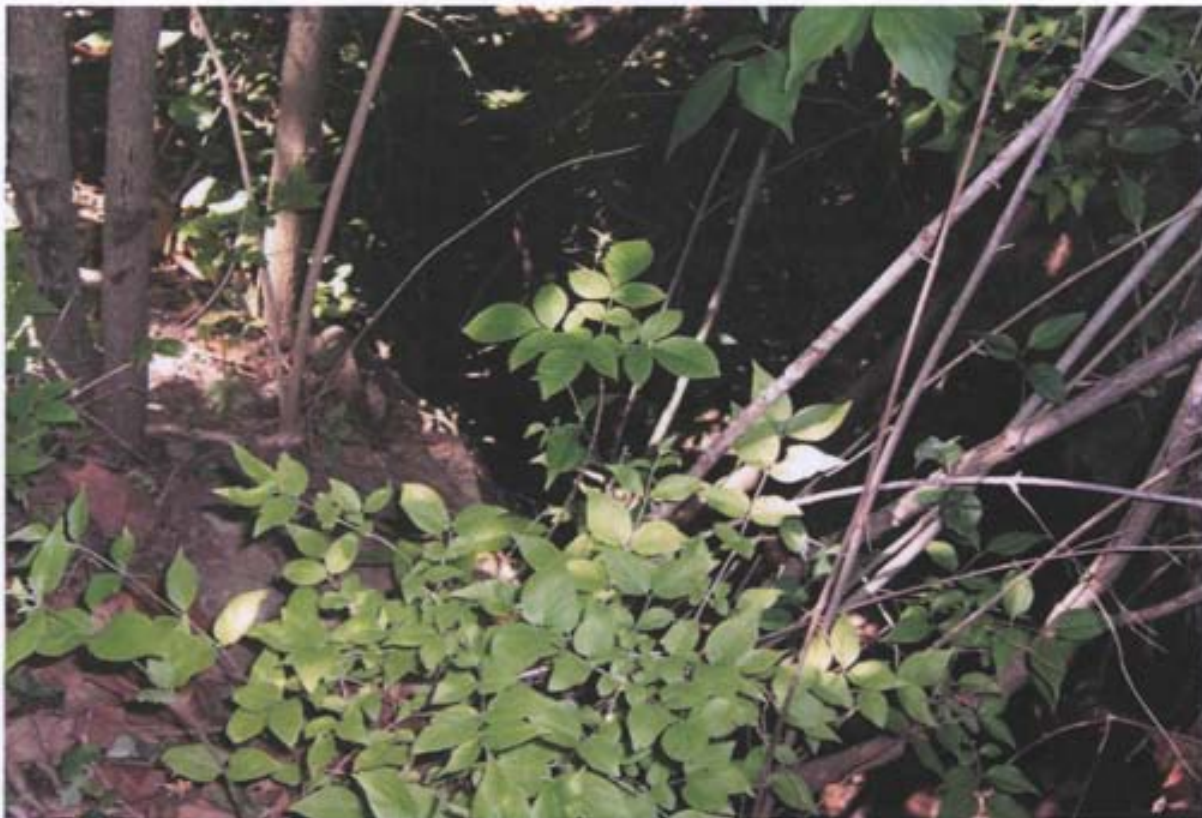
Photo 43: Close-up of 20 by 4-foot erosion feature near north IC boundary at Site LF-34.
