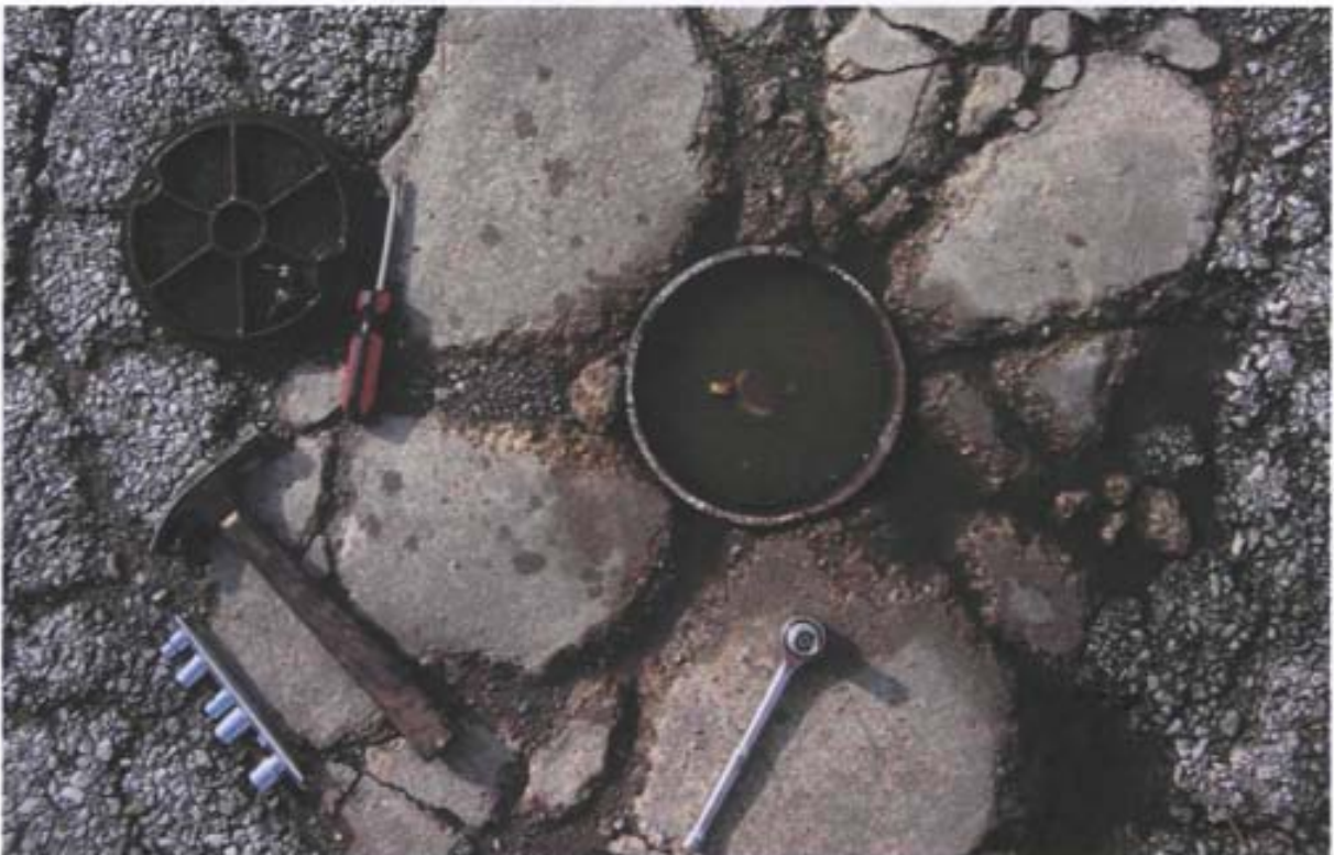
Photo 31: Close-up of submerged well protector at monitoring well SS30-MW-16 at Site SS-30.
