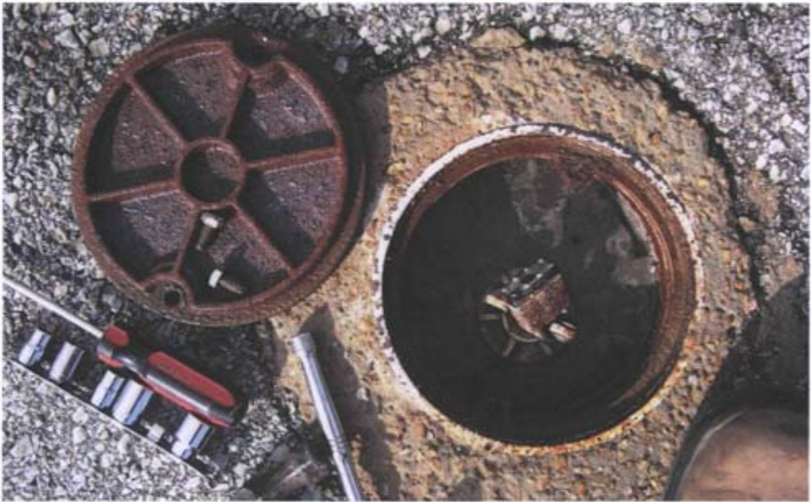
Photo 30: Closeup of partially submerged well protector at SS30-MW-18.
