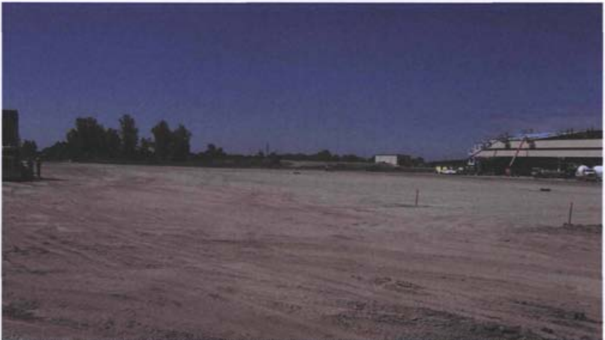
Photo 2: Southwest view of parking area and apron under construction at Sites FT-02, LF-12, and SS-44.
