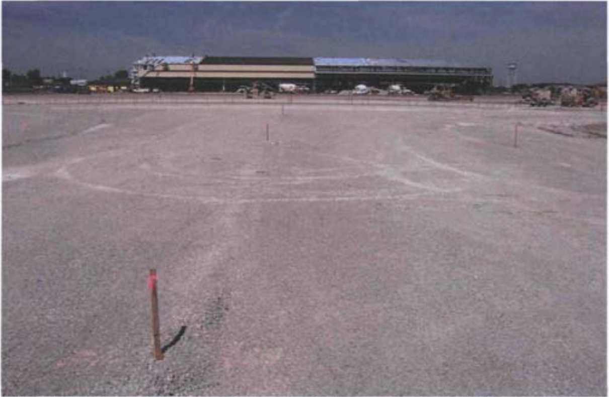
Photo 5: West view of parking area, apron, and facility under construction at Sites FT-02, LF-12, and SS-44.
