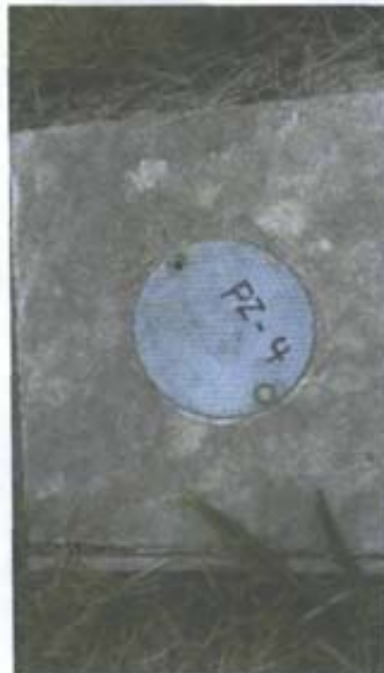
Photograph No. 22 Description: PZ-4; note one bolt not attached. Date: June 15, 2010
