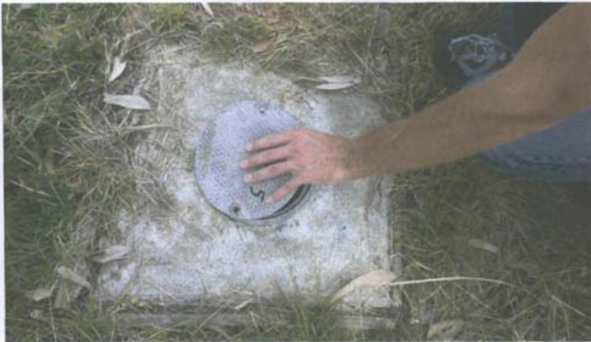
Photograph No. 21 Description: PZ-5 cap detail. Date: June 15, 2010
