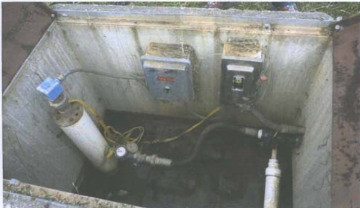
Photograph No. 12 Description: Alternate view inside the vault at RW-1. Date: June 15, 2010
