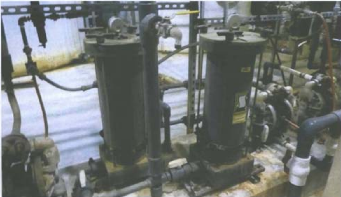
Photograph No. 92 Description: Serfilco 50-micron filters. Date: June 15, 2010
