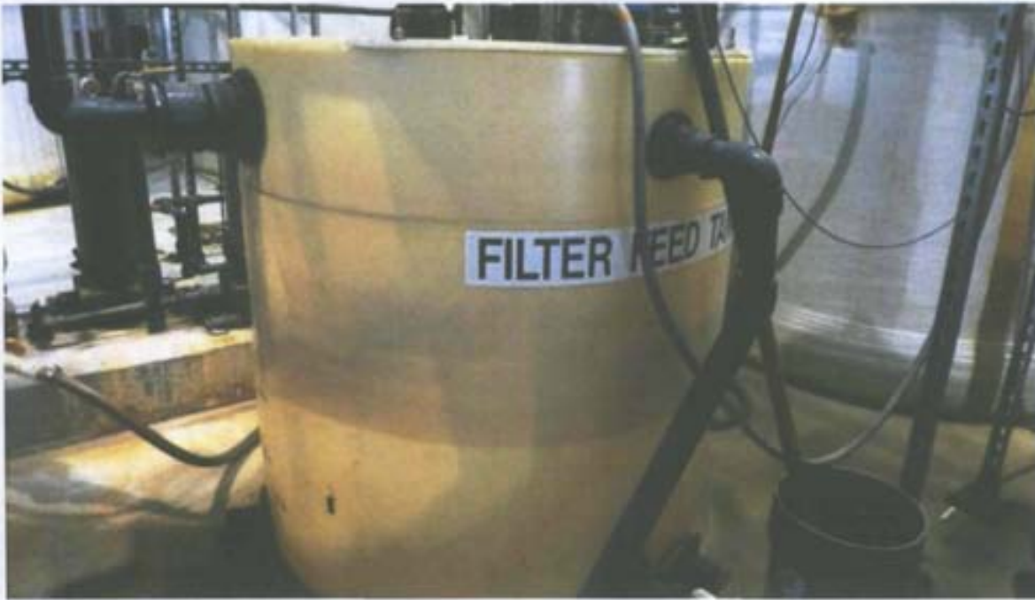
Photograph No. 91 Description: Connection from the clarifier to the filter feed tank. Date: June 15, 2010
