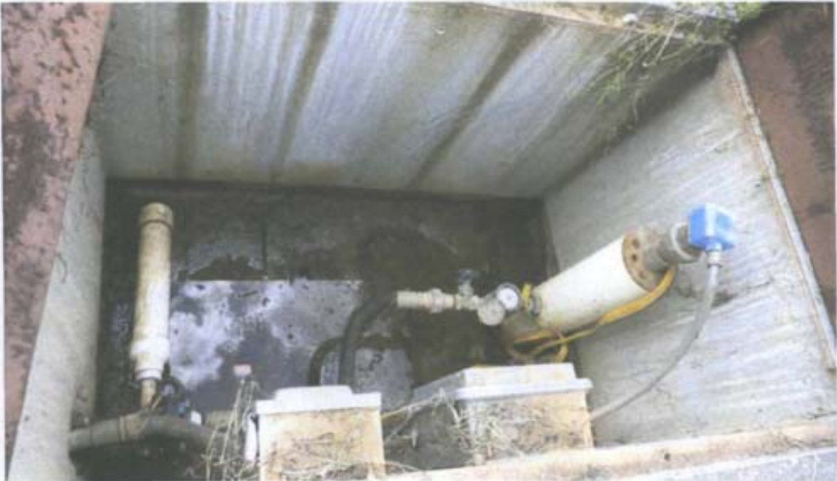
Photograph No. 11 Description: View inside the vault at RW-1; note ponded water. Date: June 15, 2010
