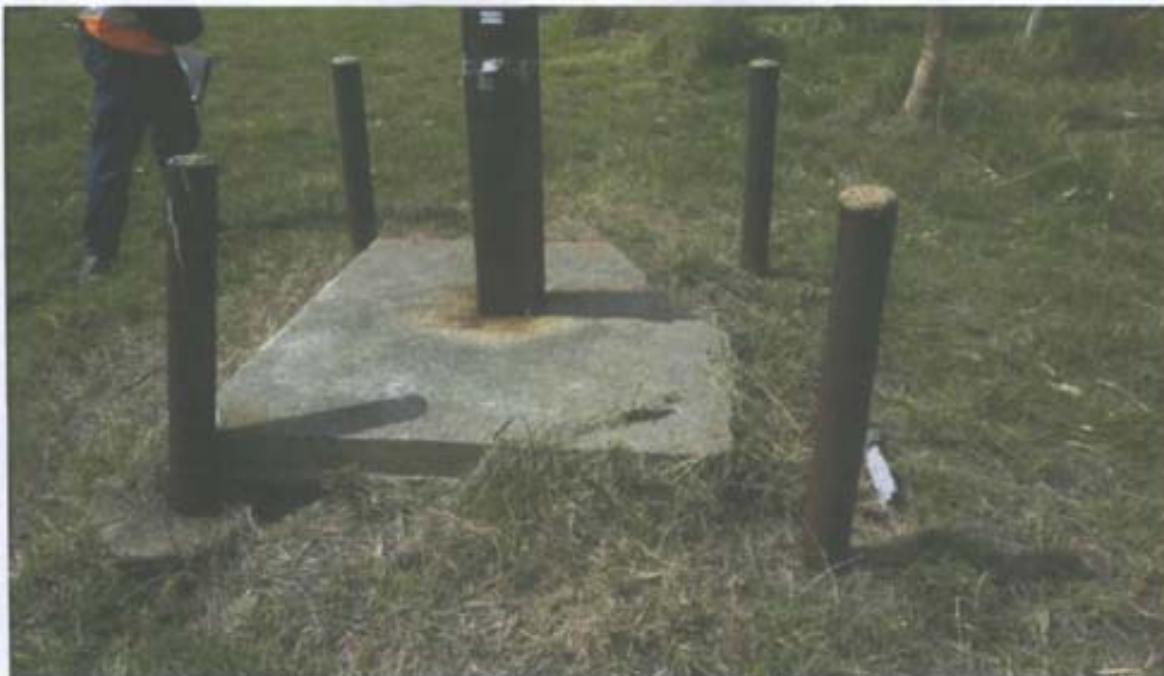
Photograph No. 7 Description: Monitoring well MW-31A; note damaged pad and eroded soil. Date: June 15, 2010
