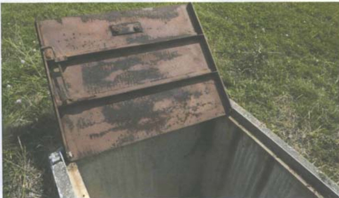
Photograph No. 16 Description: Detail of vault cover at RW-1; note broken hinge in upper right side corner. Date: June 15, 2010
