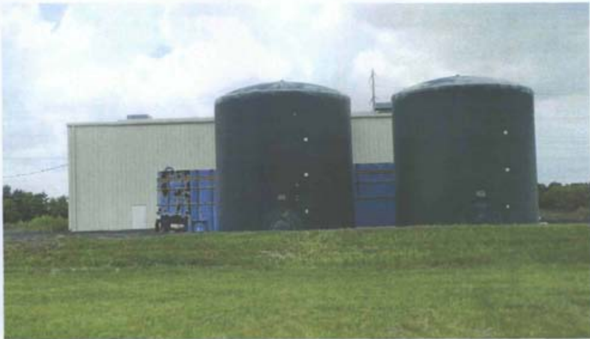
Photograph No. 55 Description: Storage tanks (each green tank is 20,000-gallon usable capacity). Date: June 15, 2010
