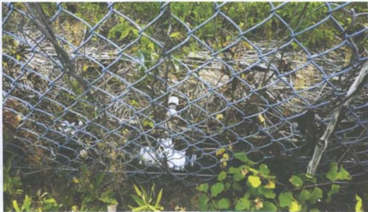
Photograph No. 38 Description: Irrigation outlet for the monofill used during the establishment of the vegetative cover. Date: June 15, 2010
