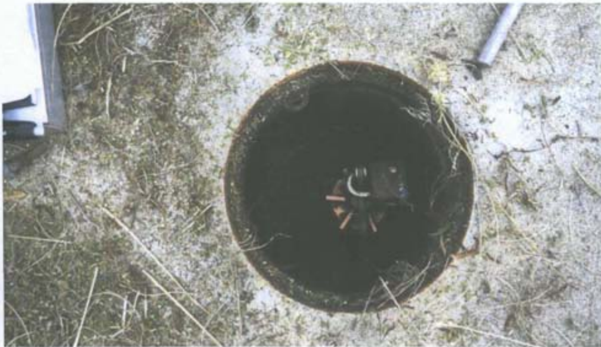
Photograph No. 42 Description: Monitoring well SW-2 detail – lock is rusted and cannot be opened. Date: June 15, 2010
