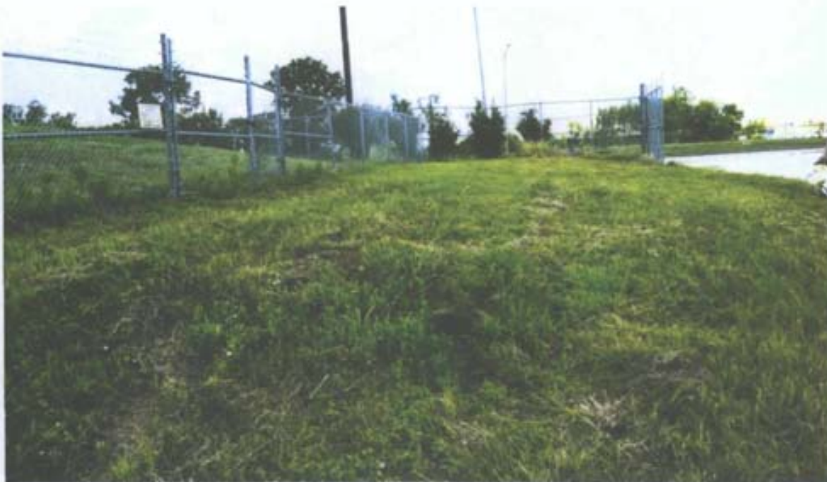
Photograph No. 44 Description: Storm drainage along the exterior side of the monofill eastern fence. Date: June 15, 2010
