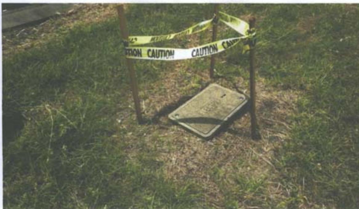
Photograph No. 84 Description: PRS electrical box. Date: June 15, 2010
