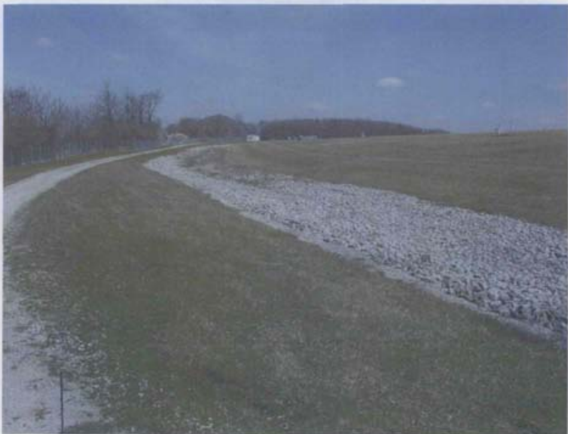
Western landfill rip-rap drainage ditch and perimeter road facing north from southwest corner of landfill
