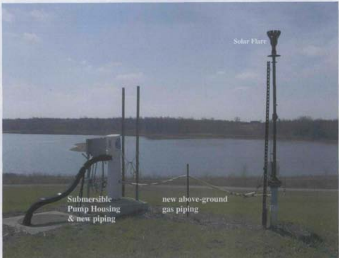
Close-up of LRW-19 and solar flare showing retrofitting with submersible pump and new piping, facing south toward Fairfield manufacturing's old stone quarry
