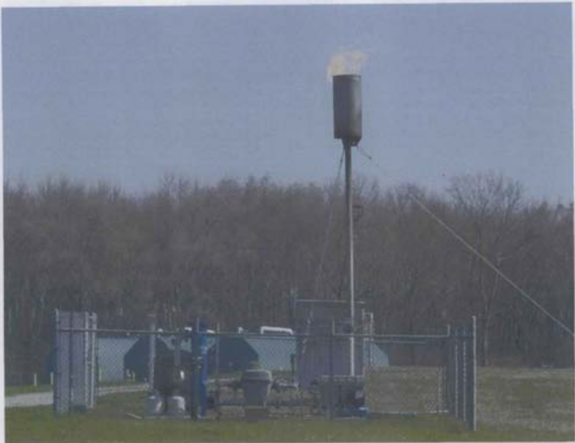
Candlestick flare with leachate storage tanks in background
