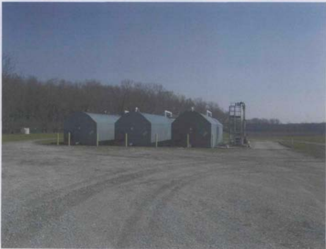
Leachate storage tanks and tanker truck loading area
