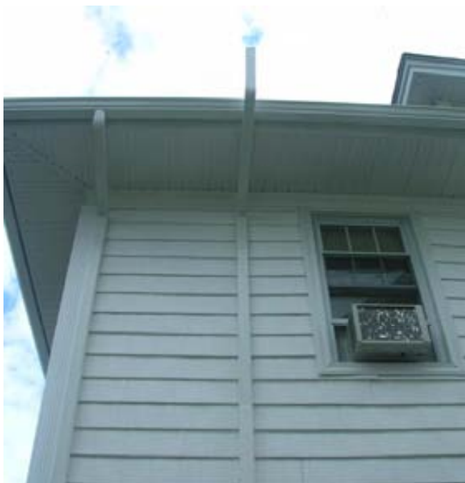
Photograph 6) House #19 – 79 Homestead Avenue: Vent Cap
