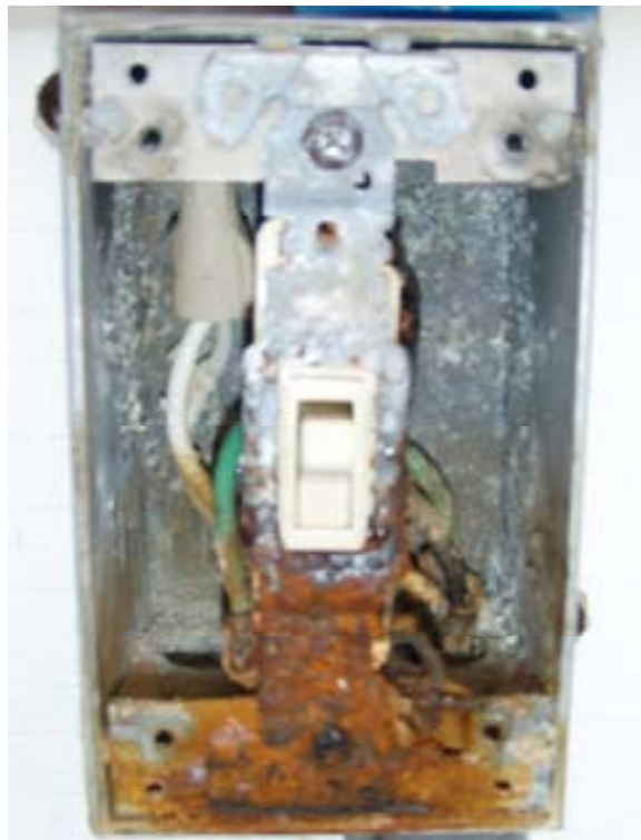
Photograph 1) House #3 – 29 Burr Place: Electric Box
