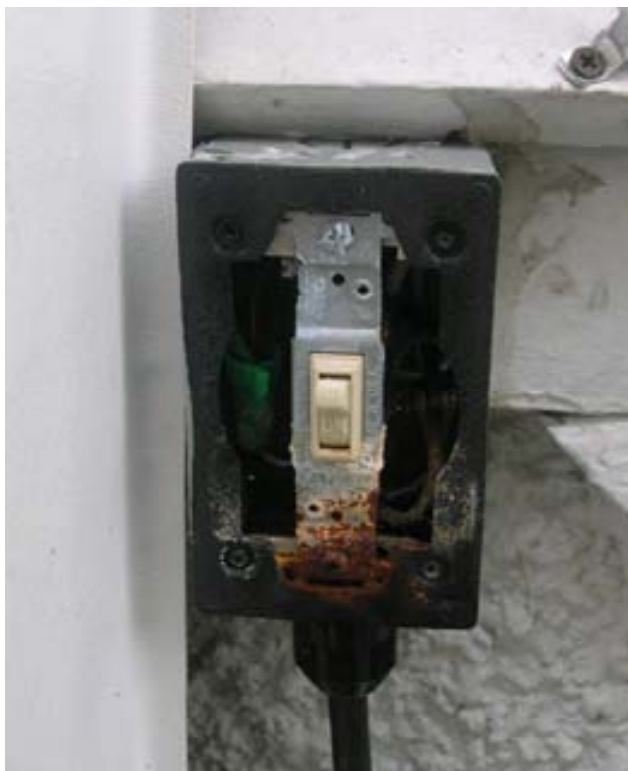
Photograph 7) House #19 – 79 Homestead Avenue: Electric Box
