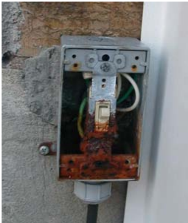
Photograph 3) House #8 – 470 Ferry Boulevard: Electric Box
