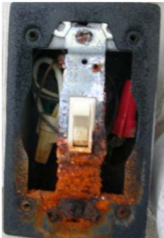
Photograph 19) House #86 – 135 Riverview: Electric Box
