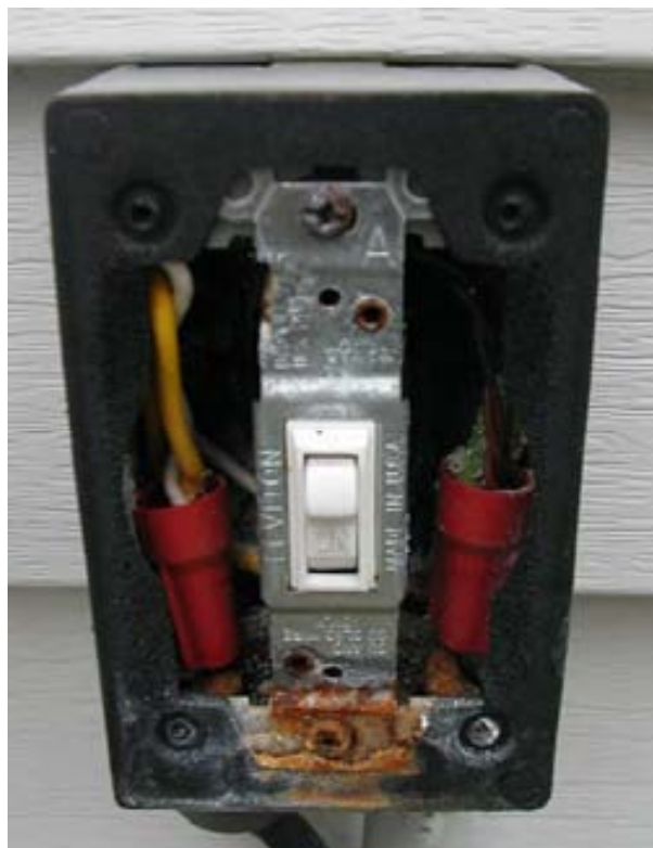
Photograph 21) House #93 – 73 Willow Avenue: Electric Box
