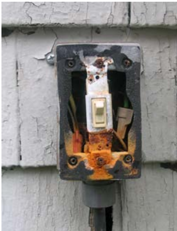
Photograph 4) House #13 – 36 Homestead Avenue: Electric Box
