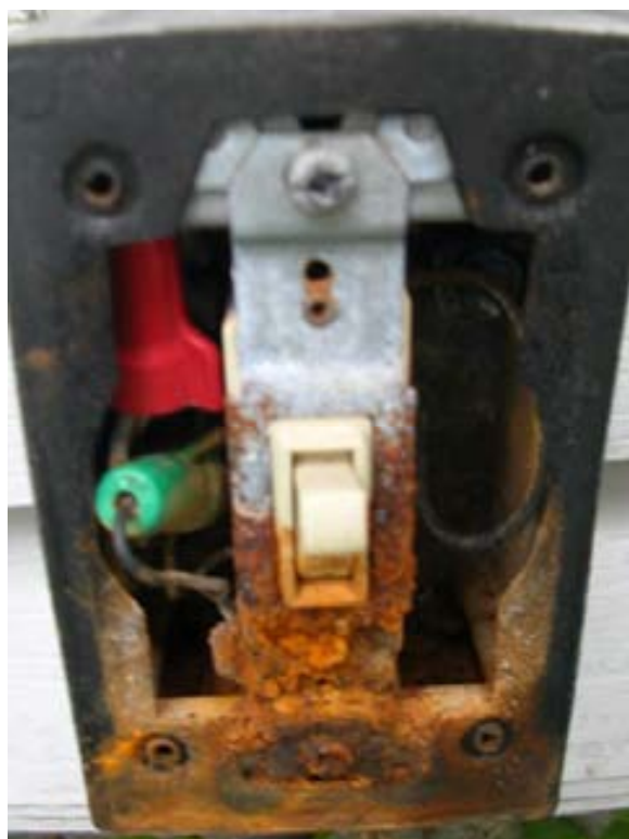
Photograph 24) House #100 – 116 Willow Avenue: Electric Box
