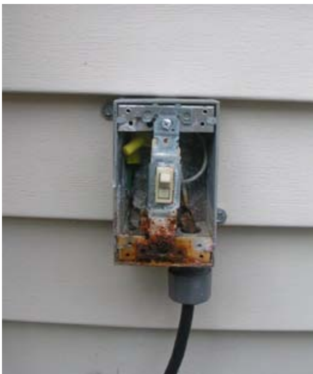
Photograph 8) House #20 – 85 Homestead Avenue: Electric Box
