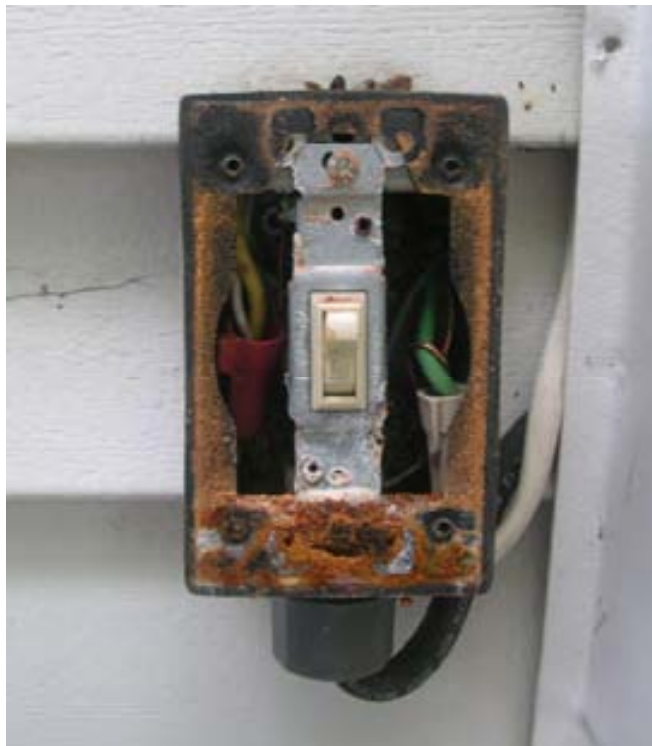
Photograph 9) House #24 – 109 Homestead Avenue: Electric Box
