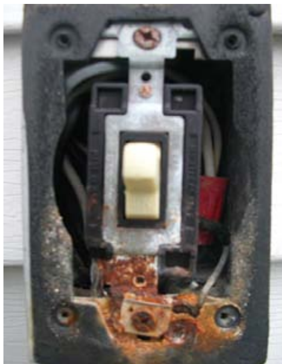
Photograph 20) House #89 – 24 Willow Avenue: Electric Box
