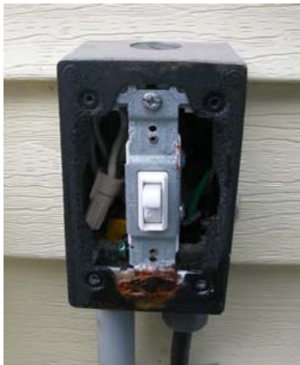
Photograph 23) House #95 – 93 Willow Avenue: Electric Box
