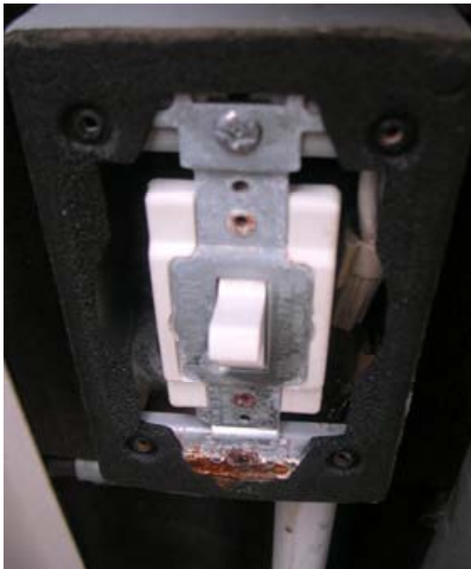
Photograph 5) House #15 – 63 Homestead Avenue: Electric Box
