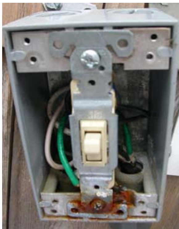
Photograph 22) House #94 – 86 Willow Avenue: Electric Box
