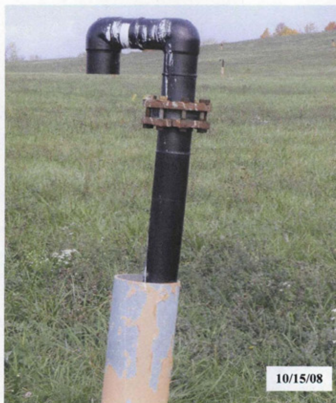
Sample port of landfill passive gas vent, on cap
