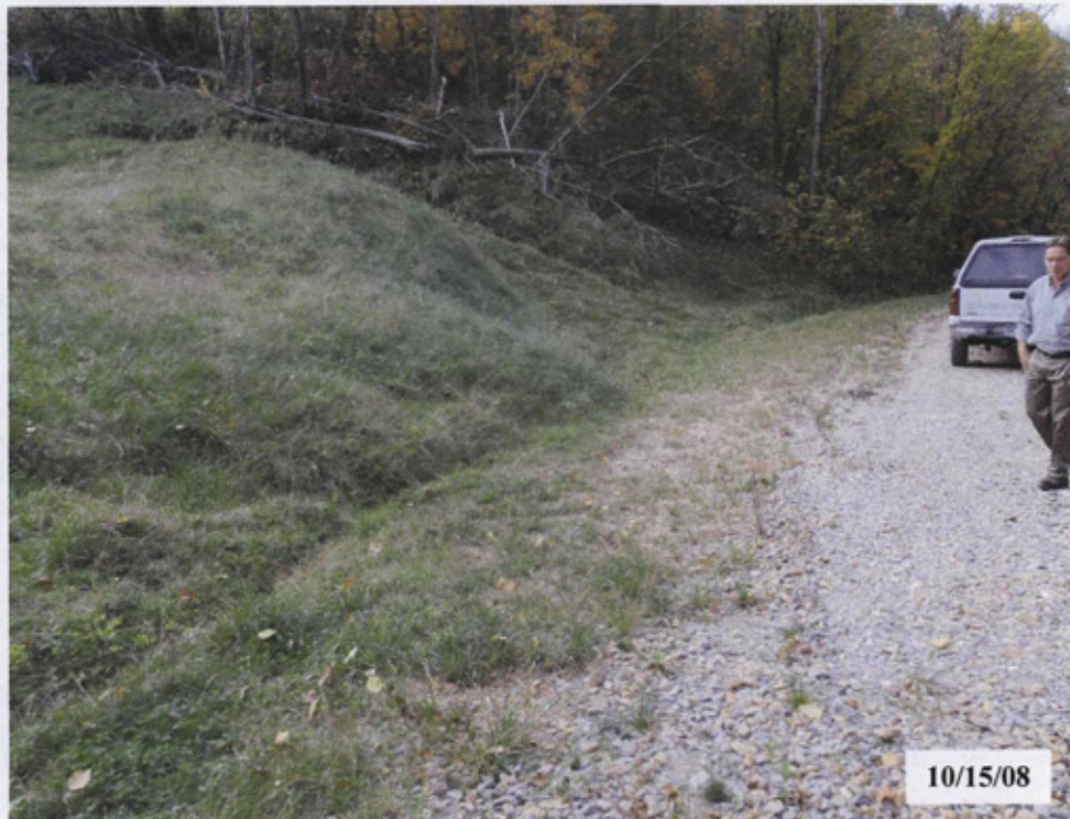
Access road outside fence, location of reoccurring erosion repair
