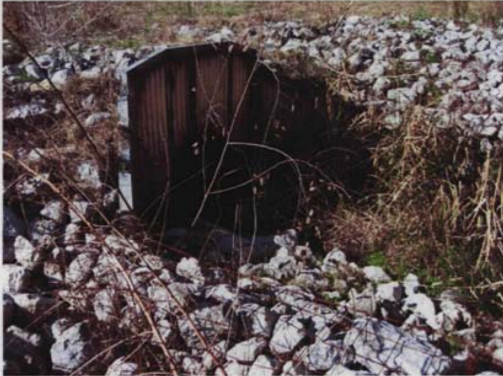
Culvert used to drain water from the nearby railroad under the Site.
