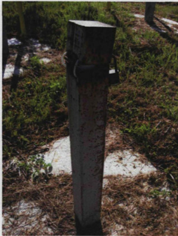
Cables used to fix monitoring wells where the hinges have broken.
