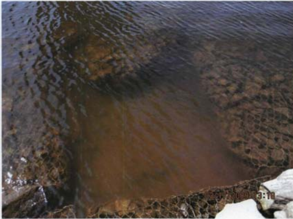
DISLODGED GABION BASKET
