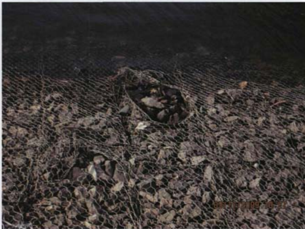
HOLE IN GABION MESH
