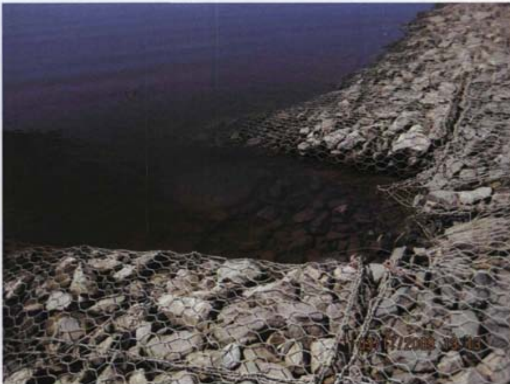
DISPLACED GABION BASKET
