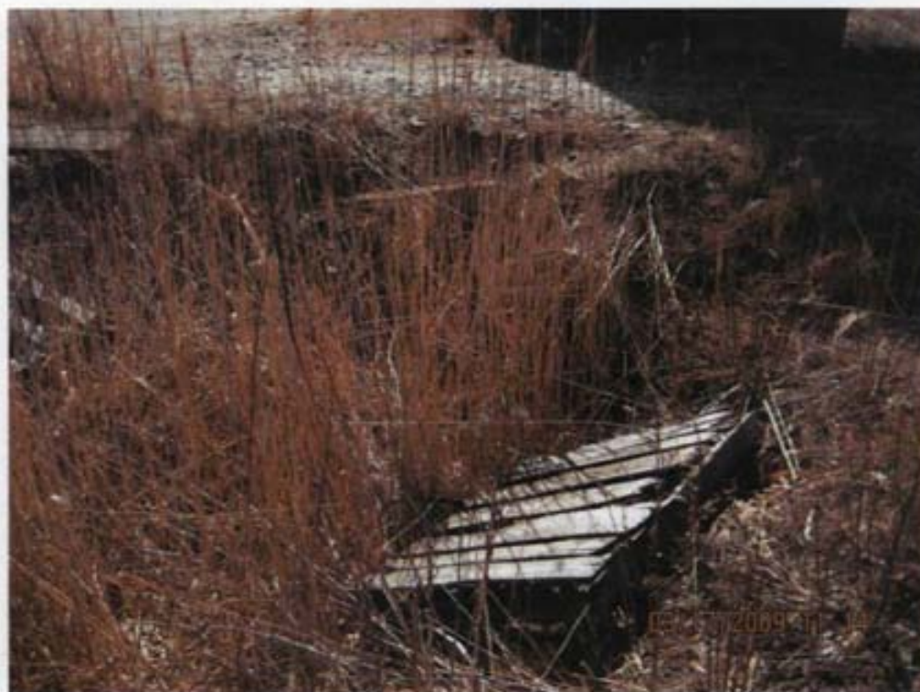
DEBRIS IN AREA A
