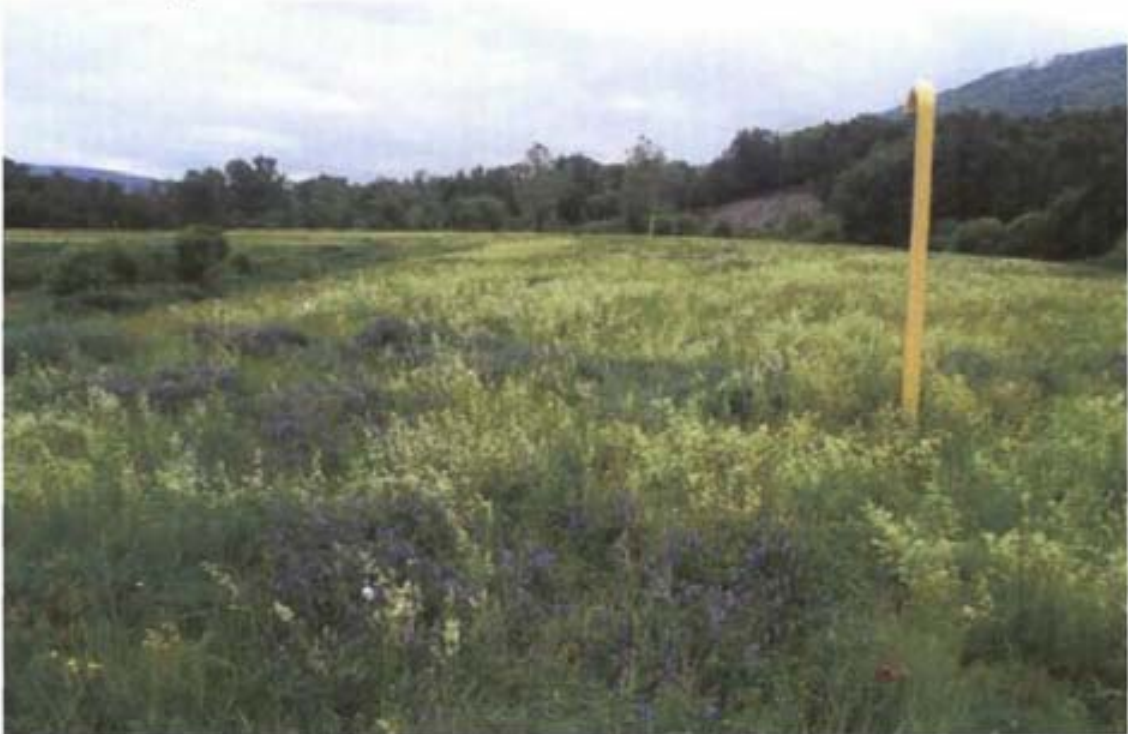
Photo 2 No signs of settlement or localized depressions. Landfill crest needs mowing. Gas vents remain undamaged and functional.
