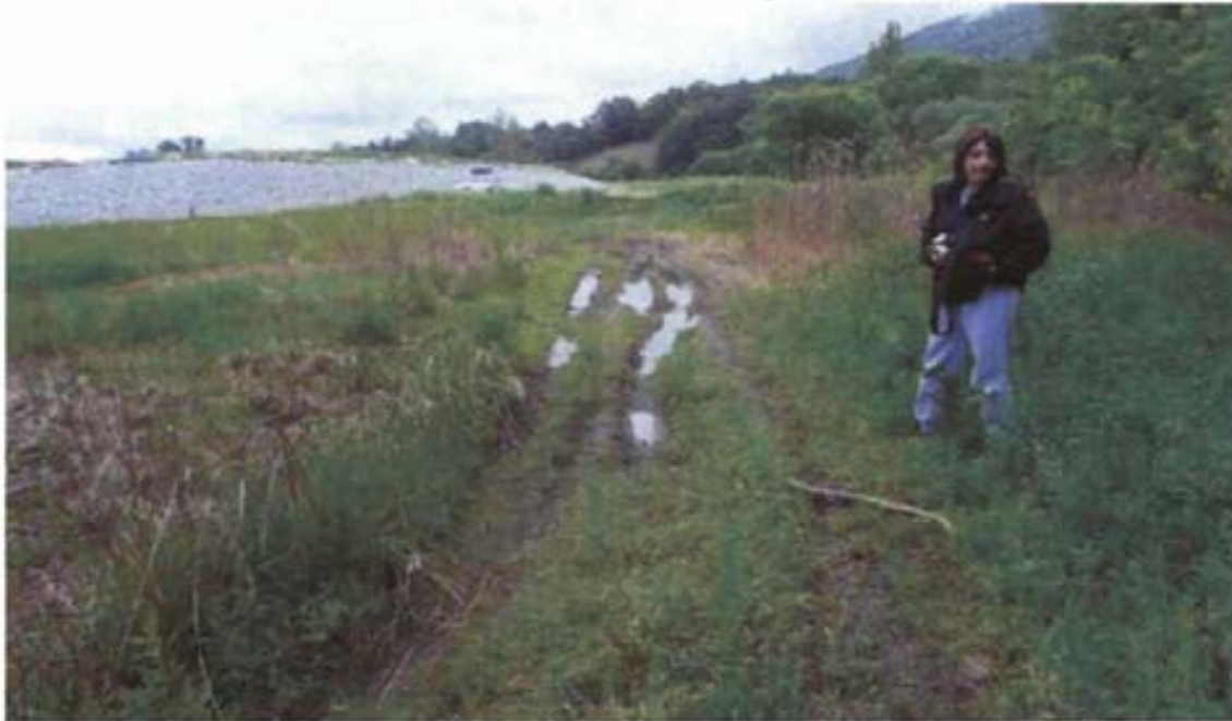
Photo 11 Ruttled access road to stabilized outlet structure requires maintenance.
