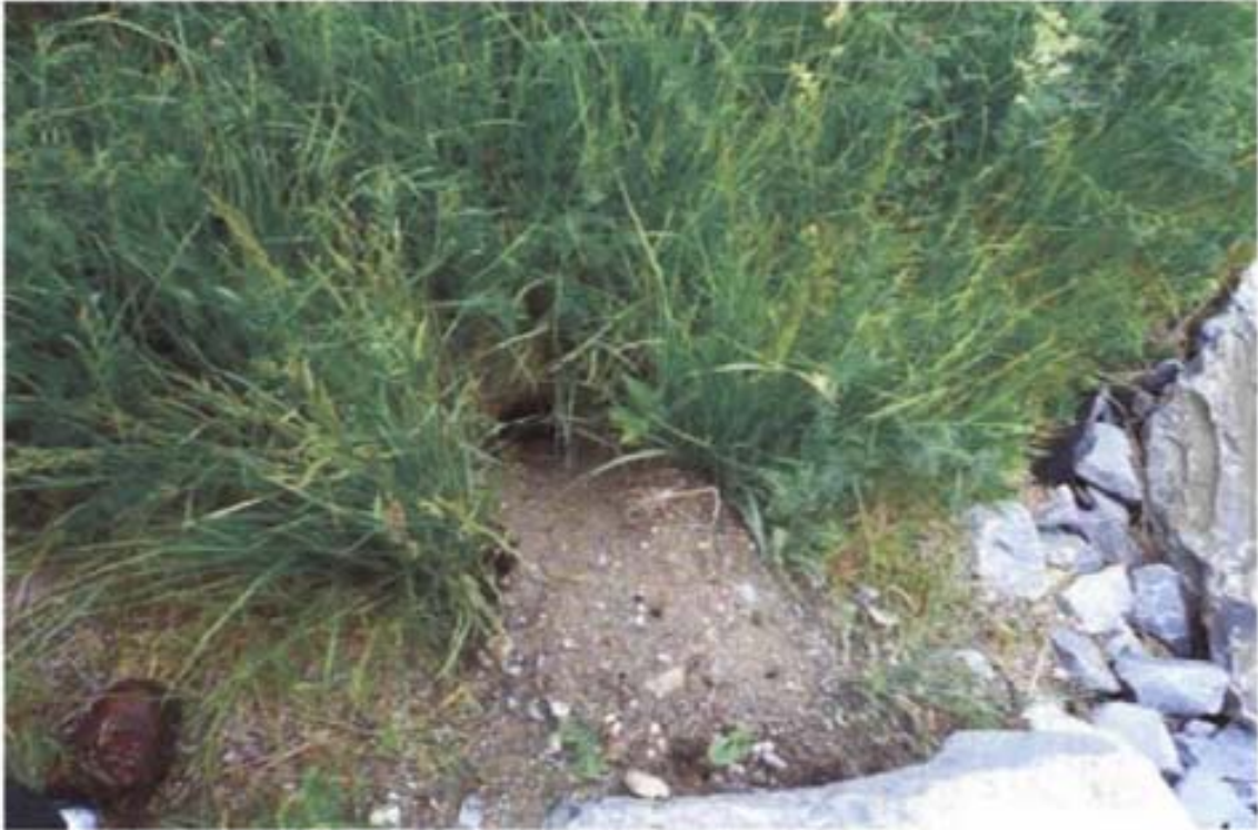
Photo 7 Animal burrow at edge of riprap above Culvert No. 2
