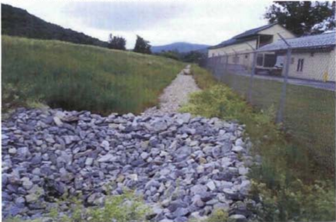
Photo 5 Lateral ditches are clear except for vegetation. Perimeter fence is in good condition.
