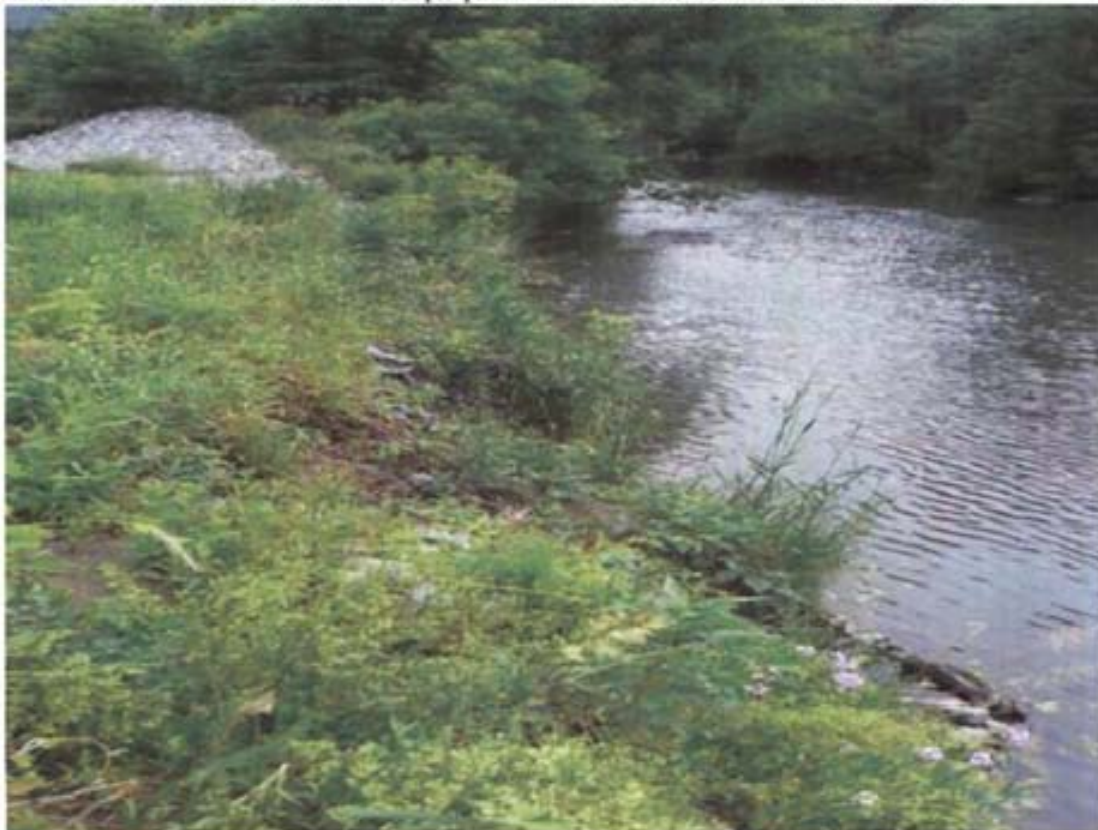
Photo 12 Bank erosion and loss of riprap has occurred at stabilized outlet structure.
