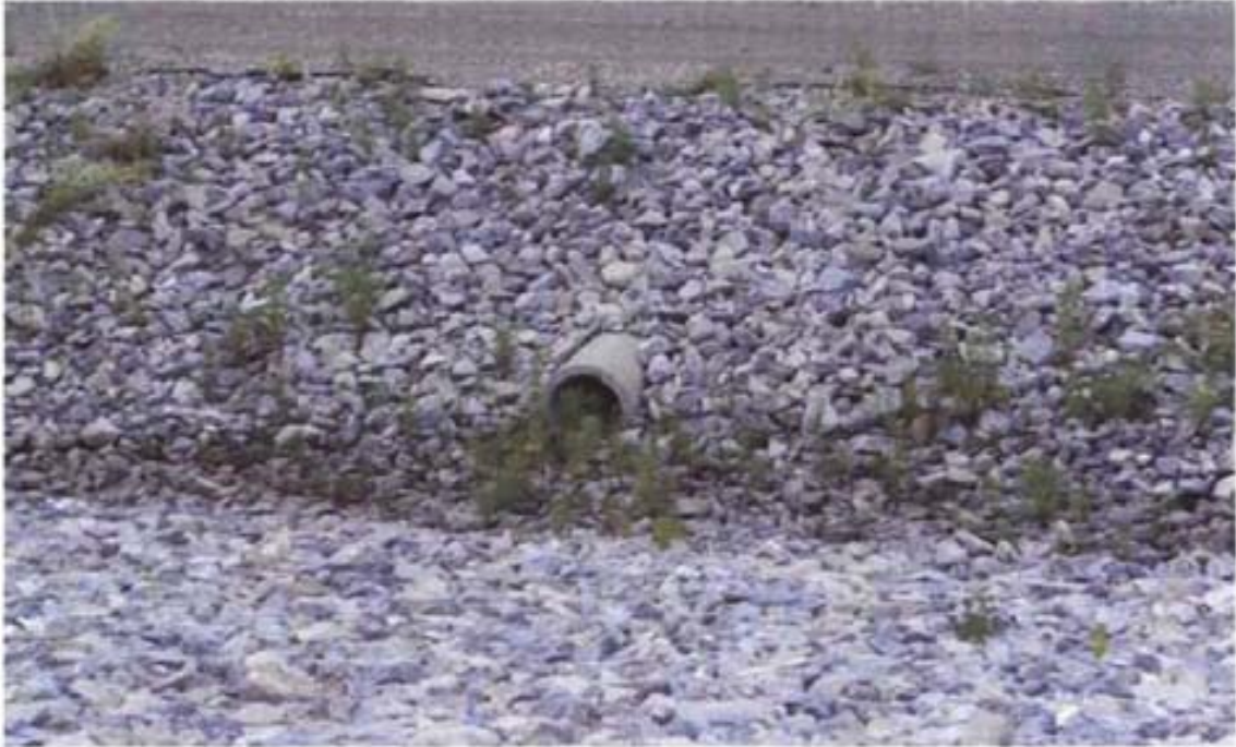
Photo 3 Vegetation growing on riprap should be removed. Culverts are unobstructed.
