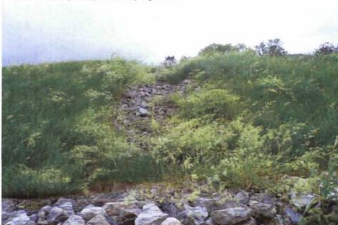
Photo 17 Swale is partially blocked by vegetation.
