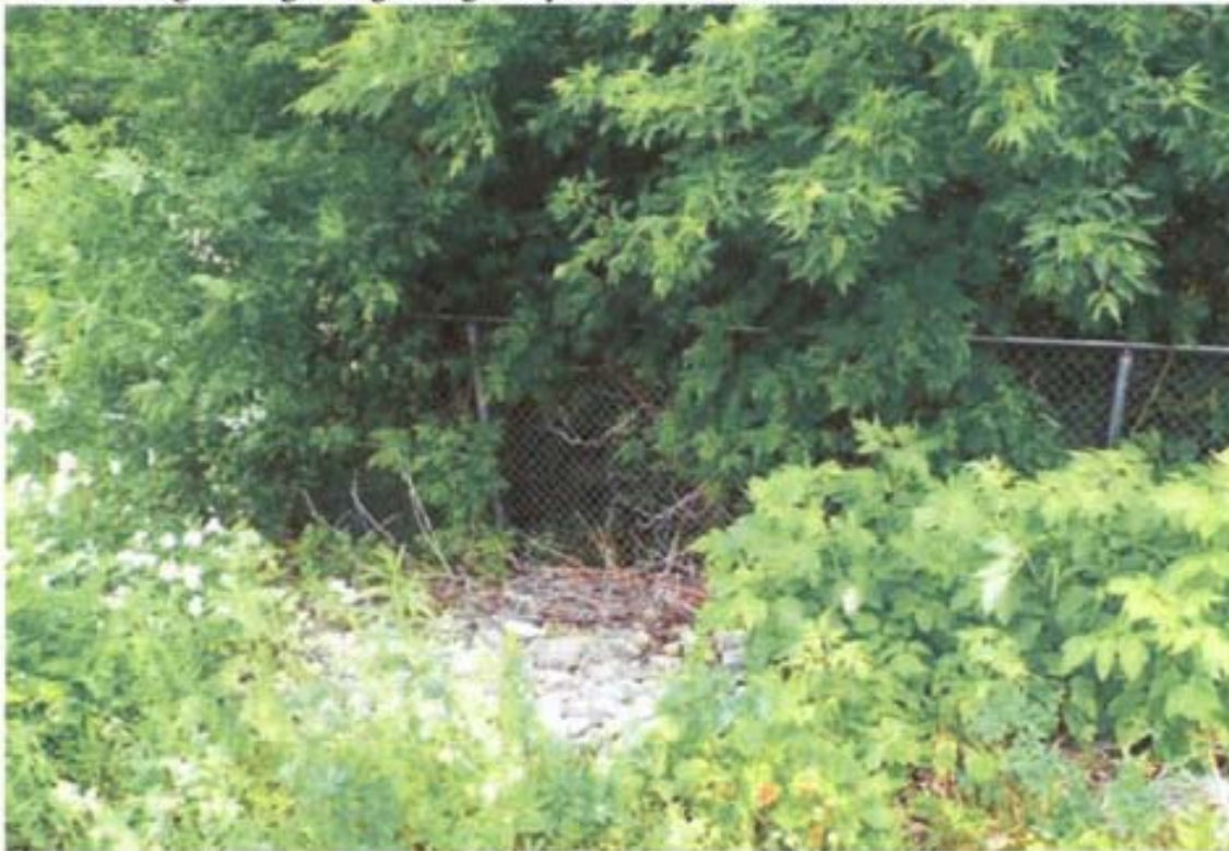
Photo 19 Vegetation growing through the perimeter fence should be cleared.
