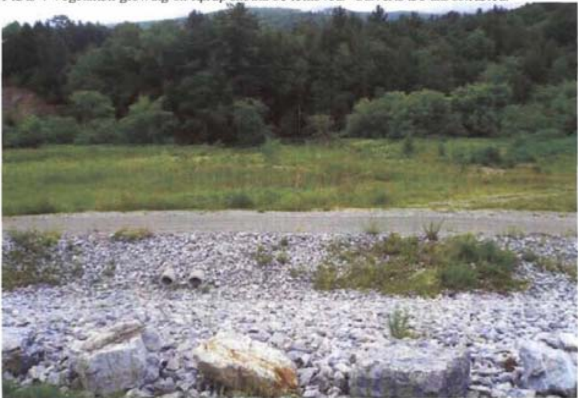
Photo 4 Vegetation growing on riprap should be removed. Culverts are unobstructed.
