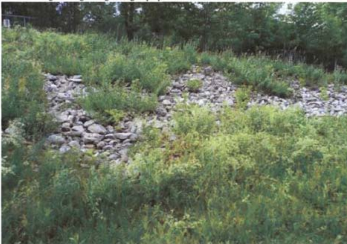
Photo 18 Vegetation growing through riprap should be removed.
