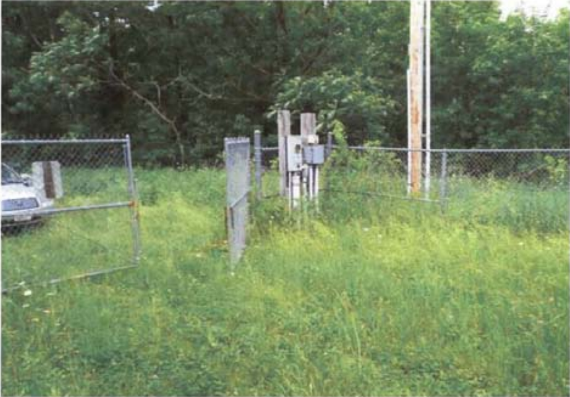
Photo 14 Locked gate and electrical panel are in good condition. Landfill vegetation is too tall.
