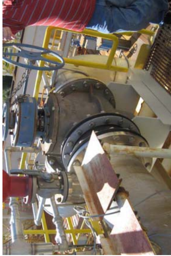
MFTP manual 3-way valve for AMD influent.
