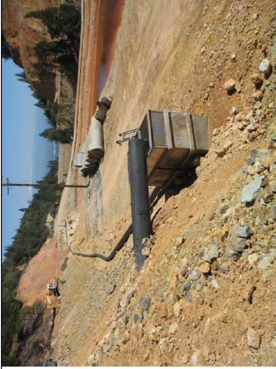
Old No. 8 gravity drain pipeline installed in March 2008. PW-3 was not being pumped at the time of the inspection.
