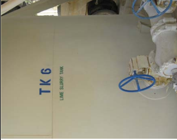
MFTP lime slurry tanks. The treatment plant has two lime slurry tanks for redundancy.
