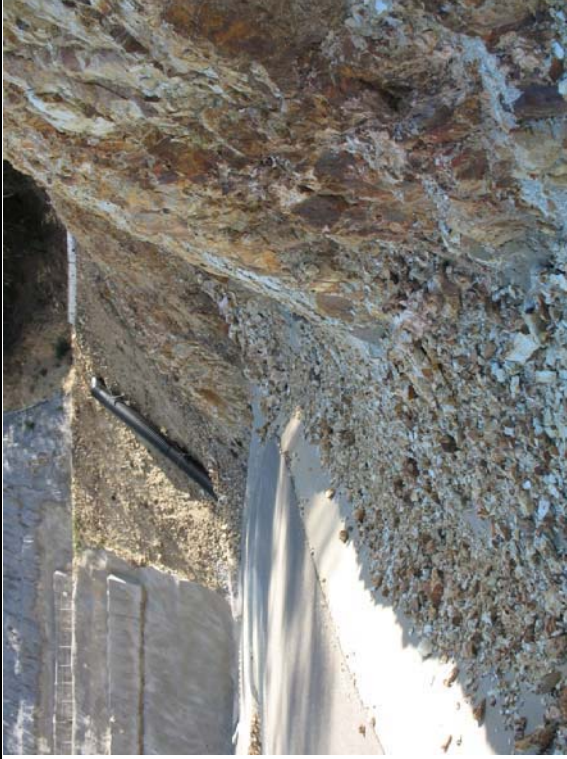
SCRR storm water channel. Rocks have accumulated in channel and need to be removed more frequently.
