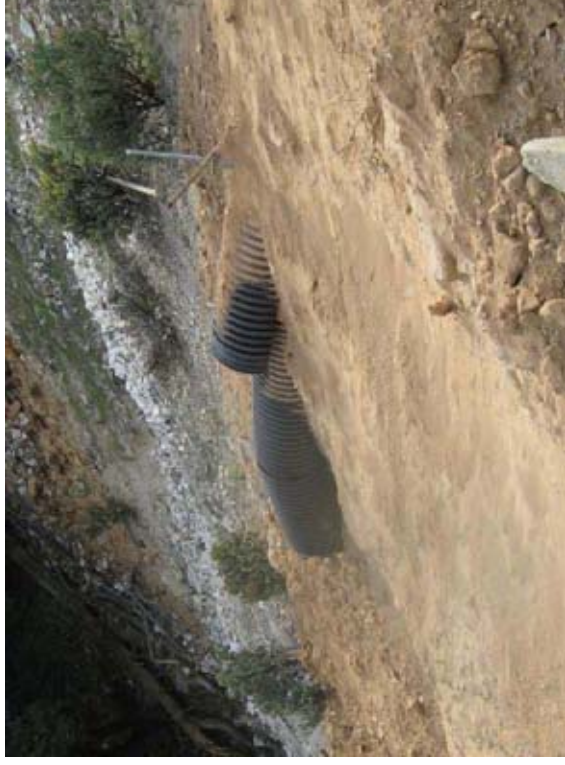
Four down comers from culverts along the Jeep Road have broken and need to be replaced. This pipeline is near mile marker 2 1/2.
