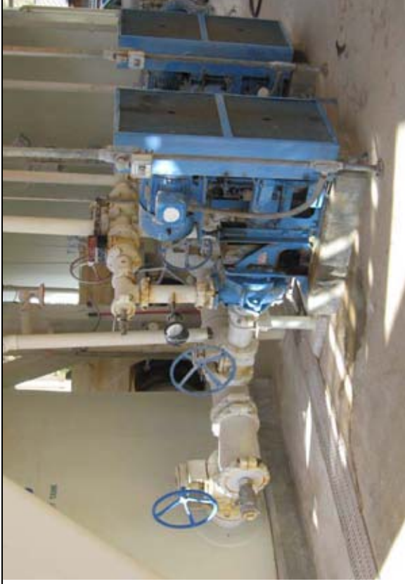
MFTP lime slurry pumps. All pumps and tanks, except the thickener, have redundancy.
