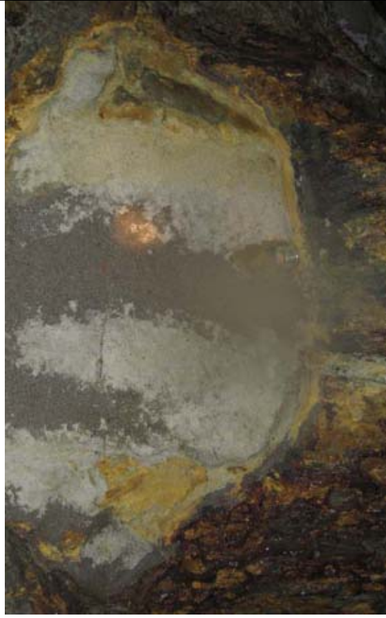
Richmond Mine. Shotcrete form has fallen off a portion of the plug. The pipe drain shown in the photo is blocked, and seepage is occurring around the edge of the chute plug.
