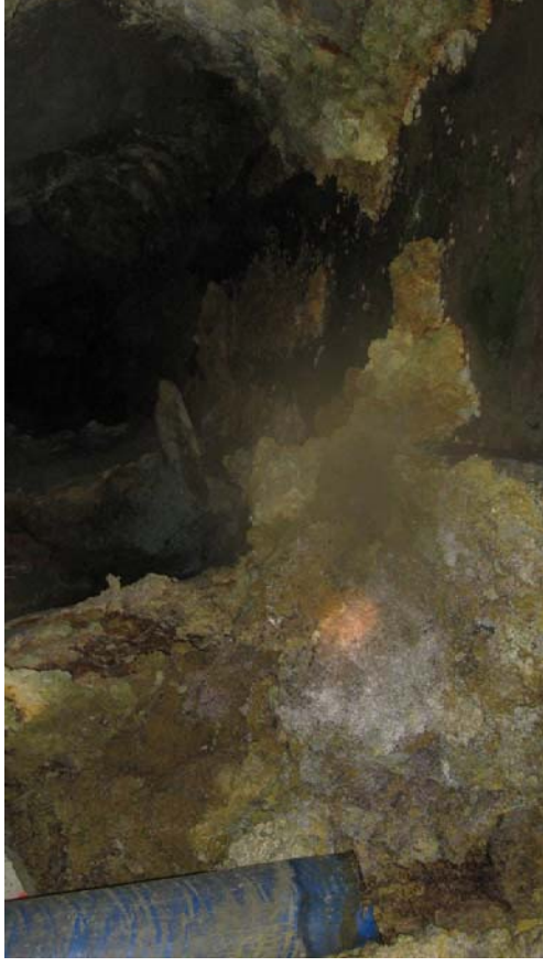
Richmond Mine. Wes Franks commented this was a pile of the shotcrete form that had fallen from the wall (the "back").
