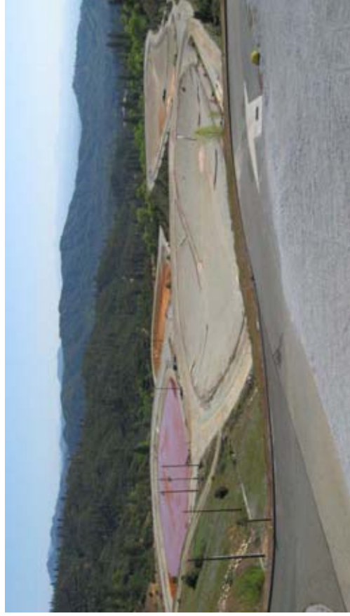
MFTP sludge drying beds. Pond # 4 was almost full and Pond # 3 was one third full, for a total sludge volume of about 20,000 yd 3 .
