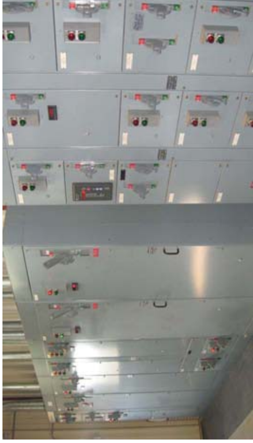
Minnesota Flats Treatment Plant (MFTP) Control Center.
