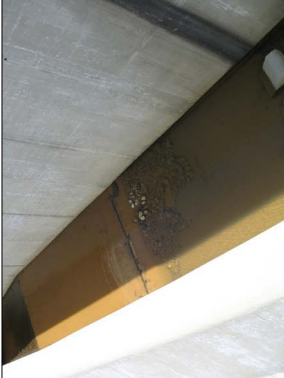
SCRR Spillway. Rocks and gravel have entered the spillway from the storm water channel.
