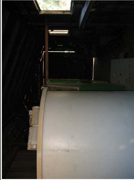
Tanks maintained by Ted Arman and located within the metal shed. Photo was taken from window on north side of shed.
