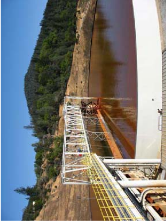
MFTP thickener. The thickener tank launder was recoated in 2007.
