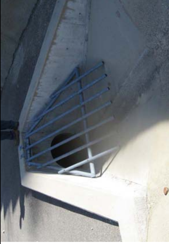
SCRR storm water channel. Gap between channel bottom and metal grate has allowed some rocks to enter spillway. Bars should be extended.
