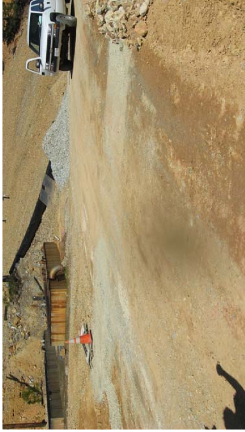
Old No. 8 PW-3 Grit Chamber shown in background. New gravity drain pipeline alignment evident in foreground, adjacent to orange cone.
