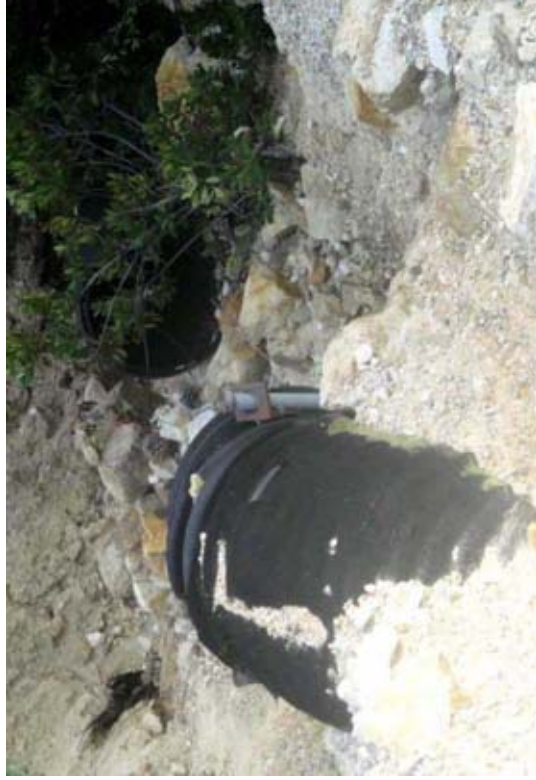
Four down comers from culverts along the Jeep Road have broken and need to be replaced. This pipeline is near mile marker 2 1/2.
