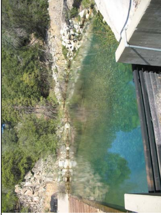
Upper Spring Creek Diversion Inlet Structure. Sand and gravel in sedimentation basin needs to be removed.
