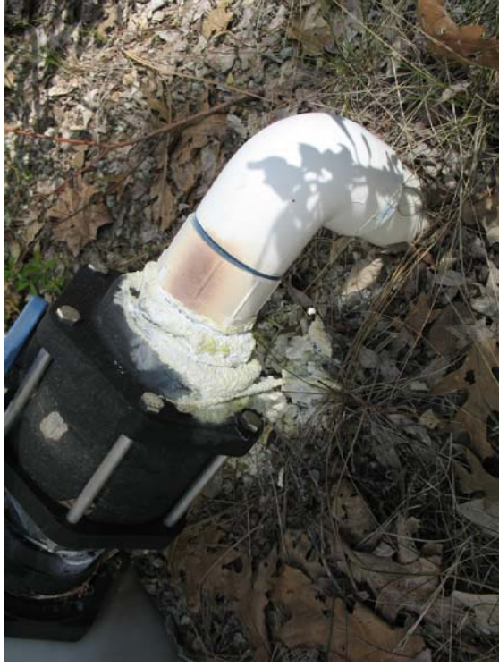
Precipitates on the pipe connection for the middle poly tank, located east of the shed, indicates a leak. There is no secondary containment.
