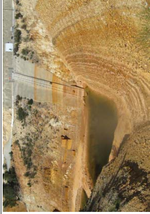
SCRR intake structure and dam. The water level this wet season came up to the second gate.
