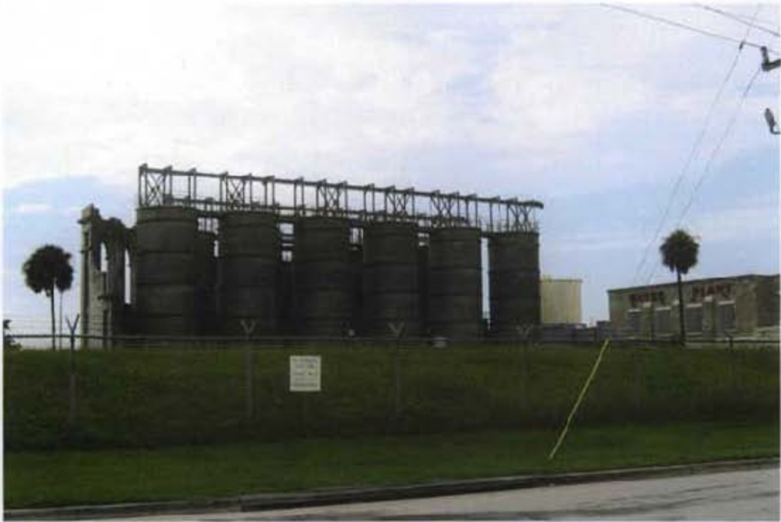
Air stripping towers at the Hialeah WTP
