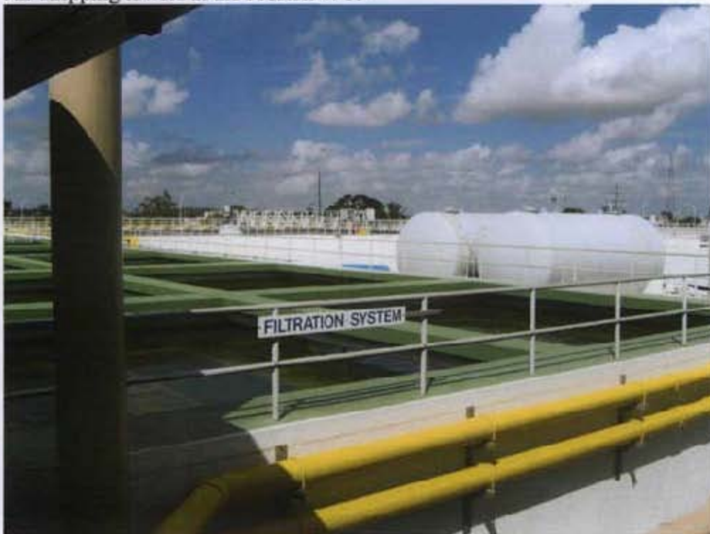
Filtration system at Preston WTP
