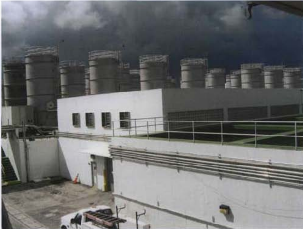
Air stripping towers at the Preston WTP
