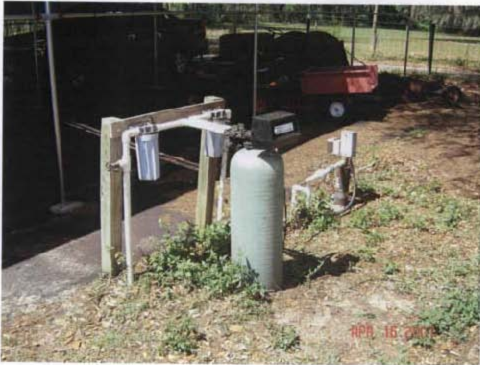
Carbon filter installed on drinking water well at Carbon Filter Location #1.
