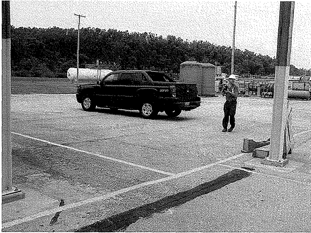
Spill Area Asphalt Cap – truck parked on cap – delineated by yellow lines
