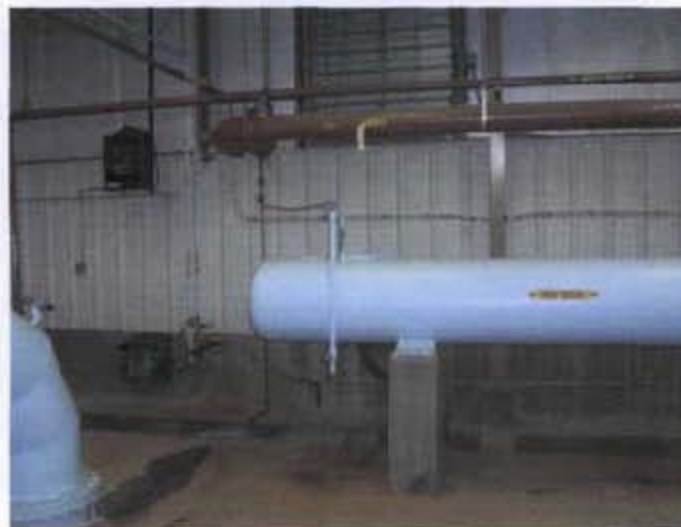
Photo 4: Water Out-take from the Air Strippers
