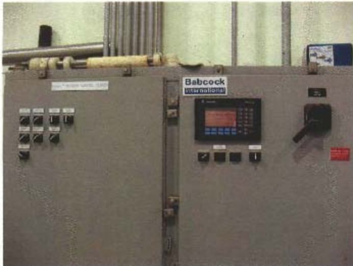
Photo 31- Package Sequencing Batch Reactor (SBR) Control
