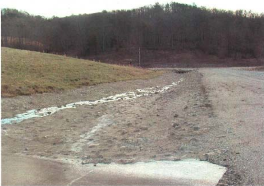
Photo 11- OU2 Surface Drainage Feature
