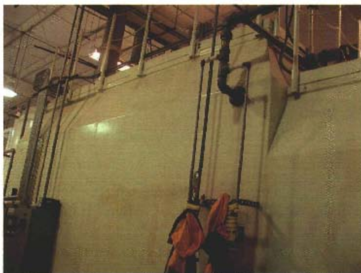
Photo 30- Package Sequencing Batch Reactor (SBR)
