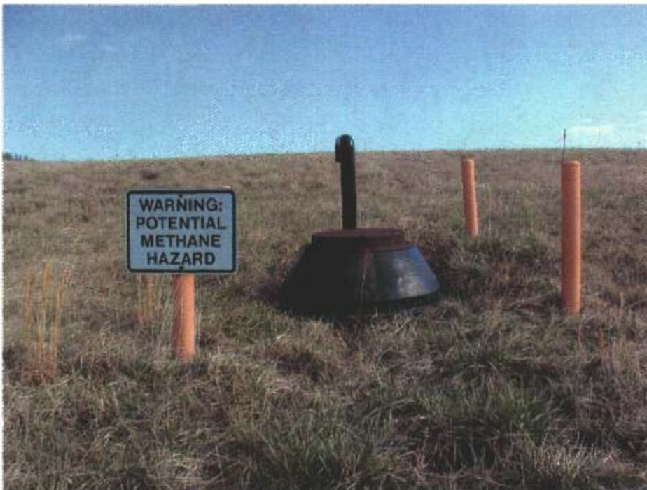
Photo 12- OU2 Typical Extraction Well, and Gas Vent
