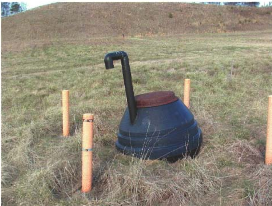
Photo 14- OU2 Typical Extraction Well, and Gas Vent: Some erosion and rodent burrowing evident at base
