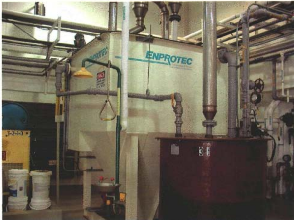
Photo 33- Package Metals Removal Unit (MRU)
