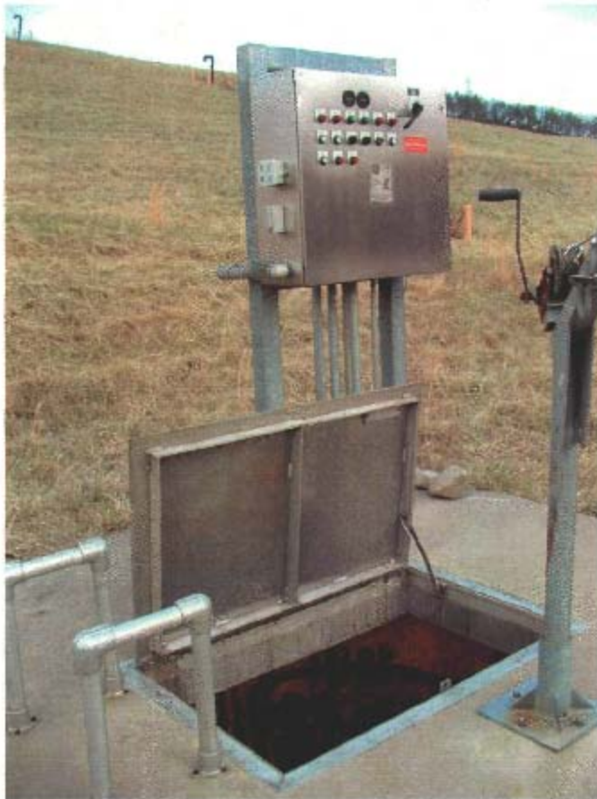
Photo 6- Leachate Collection Lift Station
