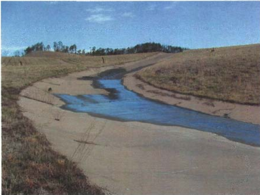
Photo 10- OU2 Surface Drainage Feature
