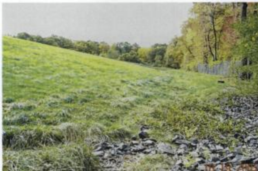
Photograph 2 – Sudbury Landfill looking west from toe of slope. (Note unwanted vegetation growing within toe-drain)
