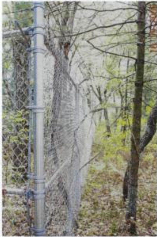
Photograph 3 – Broken limbs and small trees fallen onto perimeter fence near northeast corner.
