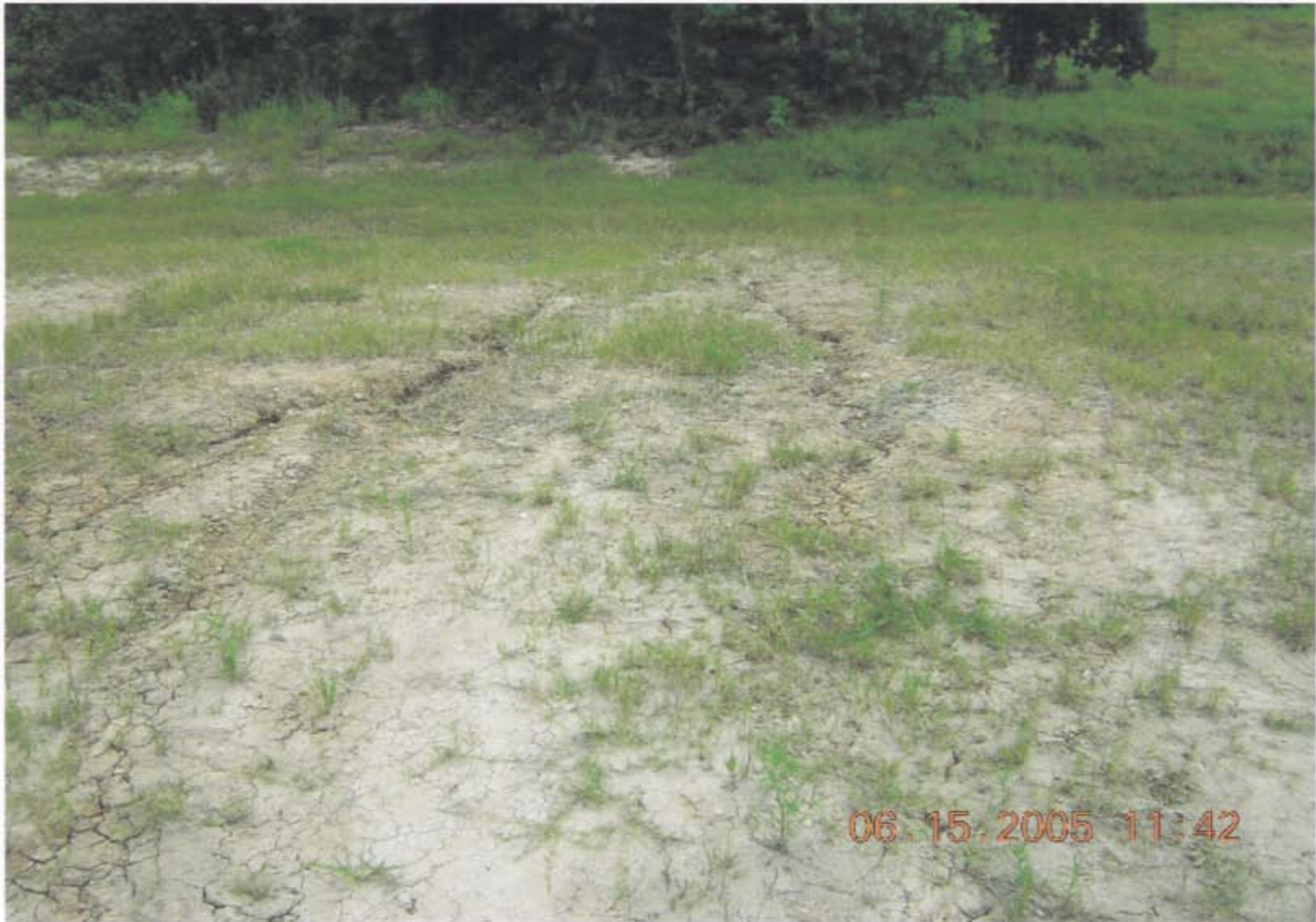
Photo 28: OU1: Erosion cuts in the north east slope of the Consolidation Cell (Pond 2).
