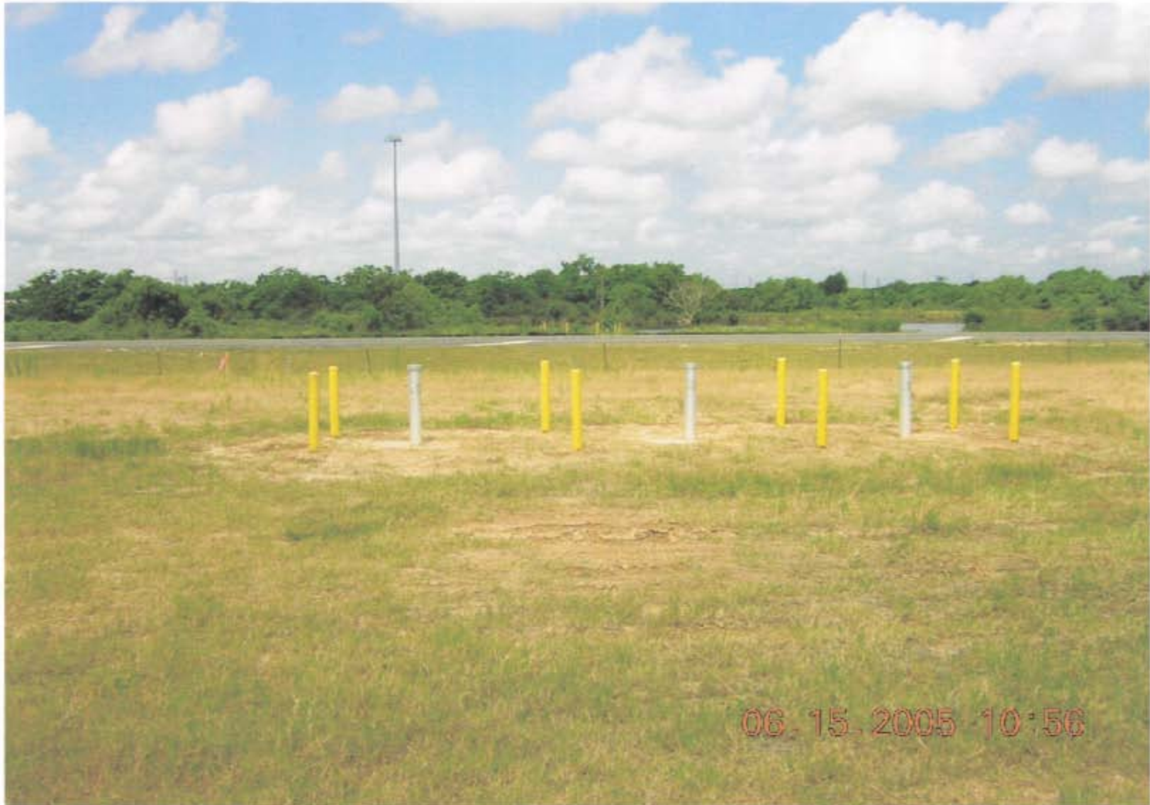
Photo 9: OU1: Site groundwater monitoring wells. ID tags and locks are in place.
