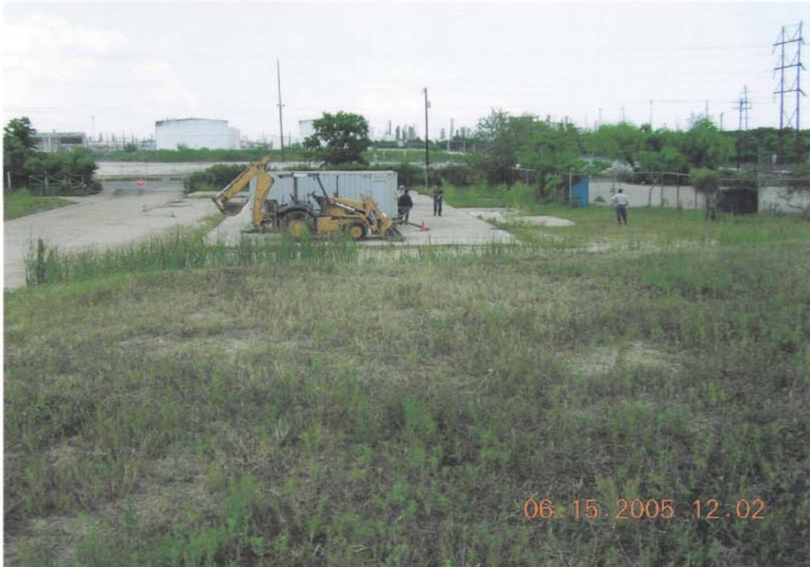
Photo 33: OU1: Equipment staging northwest of Pond 7 on former smelter concrete pads. [filename: TXT_DSCN0730.jpg]
