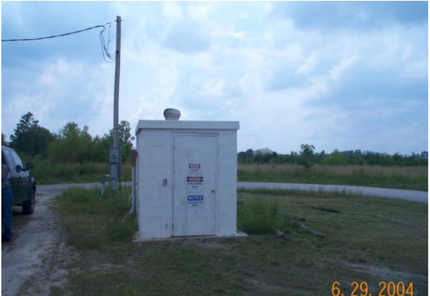
Photo 3: View of the Picher #5 MW. The City of Picher has erected a well house over the well-head and connected this well to the City water supply.
