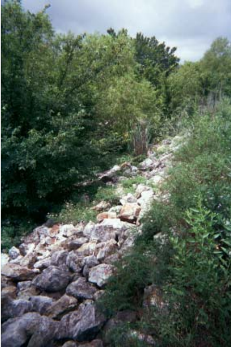
Photo 65: View of diversion dike at the Big John Mine site, located in Kansas. The subsidence feature is located to the right of this view. Large rocks were put in place to protect against erosion.
