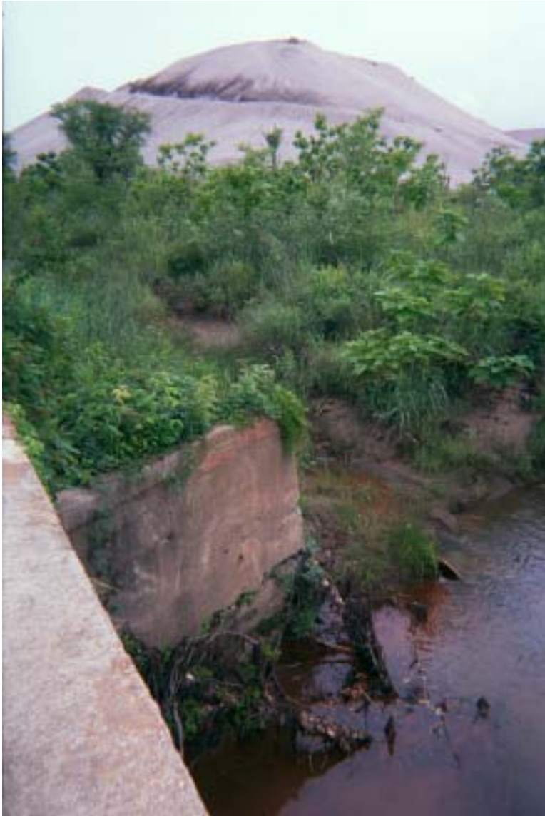
Photo 74: View of Tar Creek at the Douthat Bridge. This picture was taken of the upstream side of the creek. Note the red tint to the water from iron oxide precipitation. This location is where acid mine water starts to enter Tar Creek.
