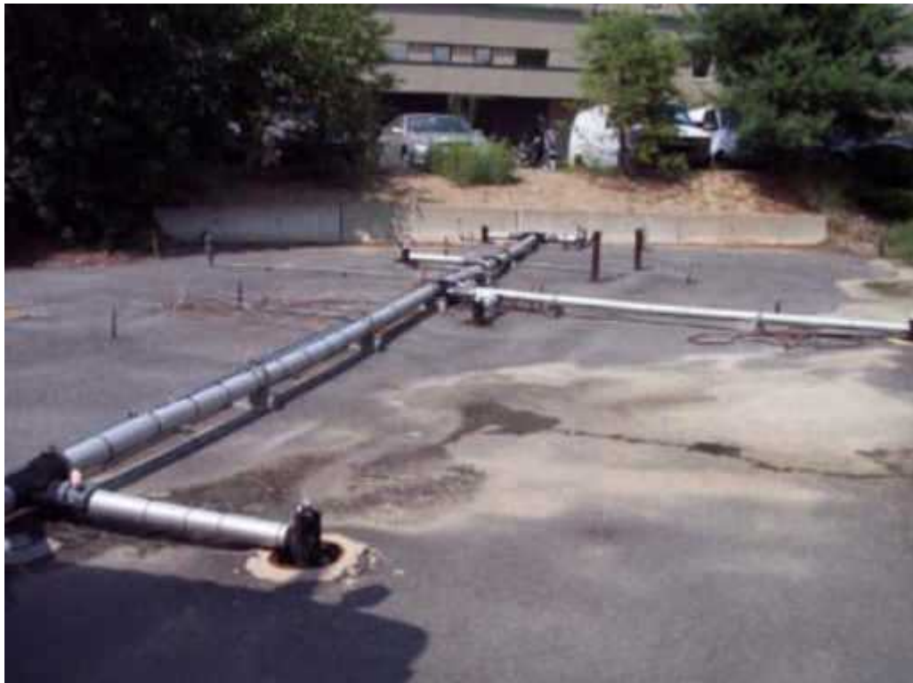
NEP Photo 2: Air Sparge System Wells 101 A&B
