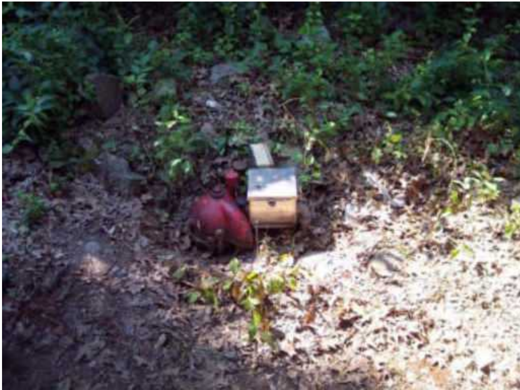
UniFirst Photo 13: Pumping Well UC22
