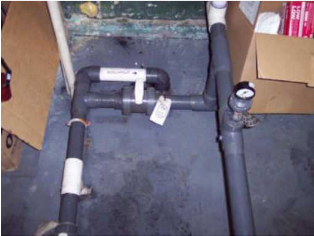
UniFirst Photo 11: Discharge Clean Water to Storm Sewer
