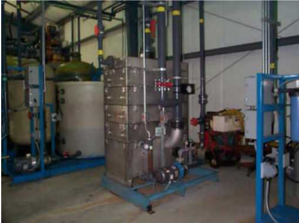
Wildwood Photo 5: Air Scrubber
