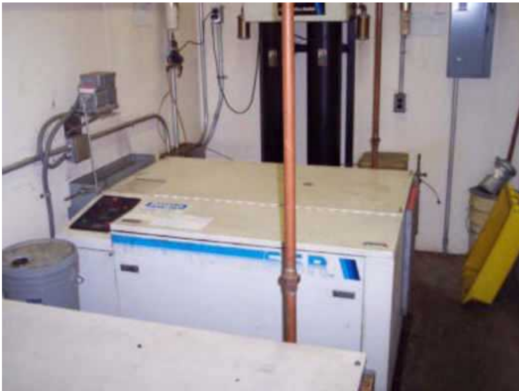
Grace Photo 10: Air Compressors
