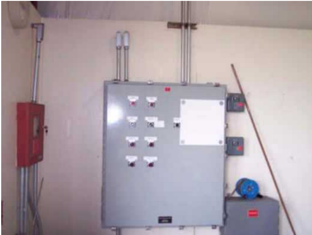
Grace Photo 9: Alarm Panel
