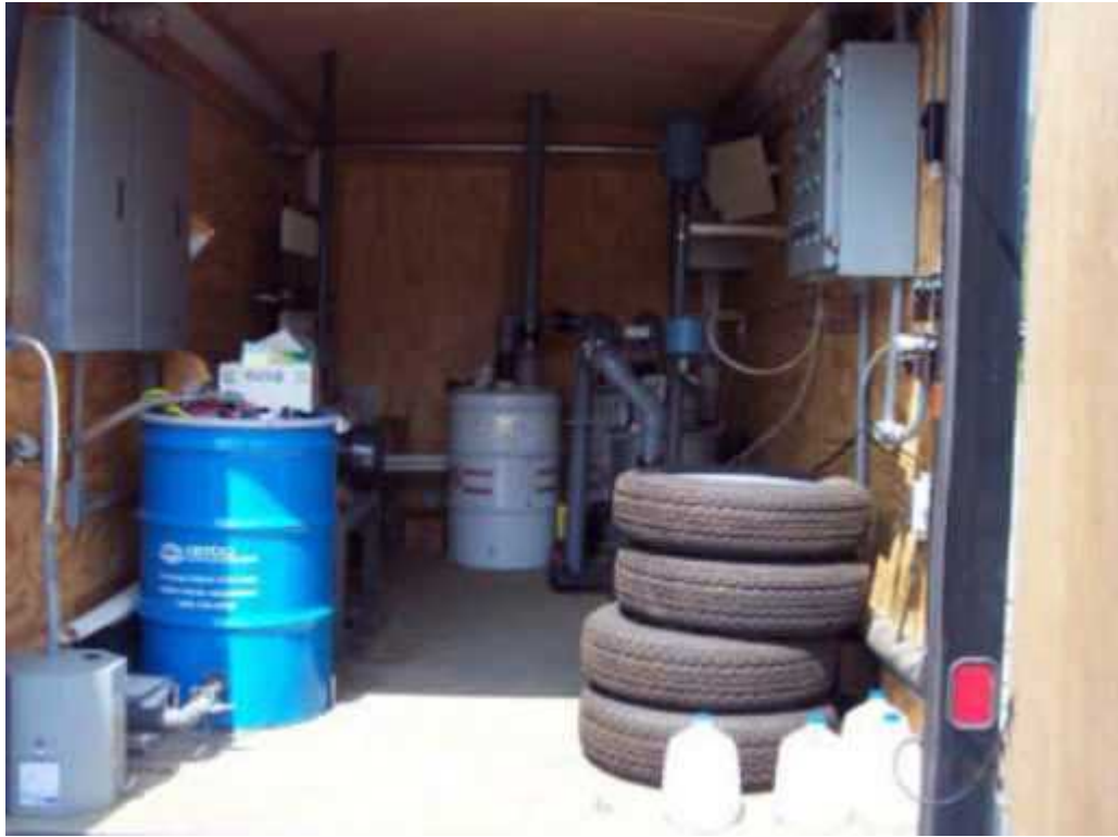
NEP Photo 3: Treatment System
