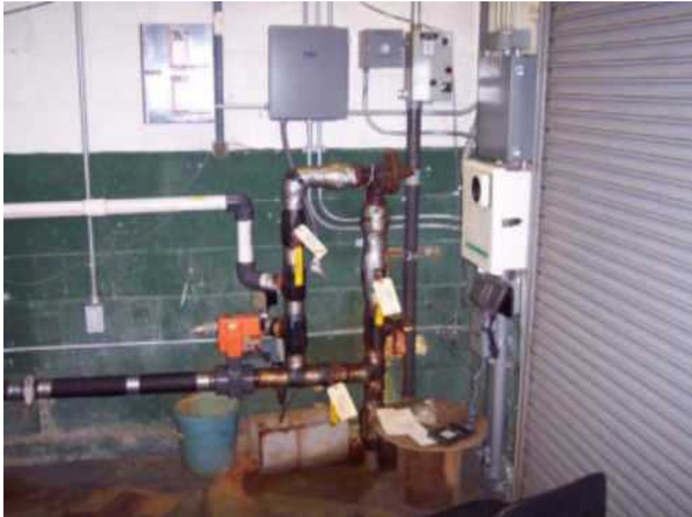
UniFirst Photo 1: Influent Piping/Gauging
