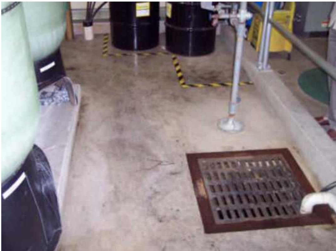
Grace Photo 6: Floor Sump Area, note excess water on floor
