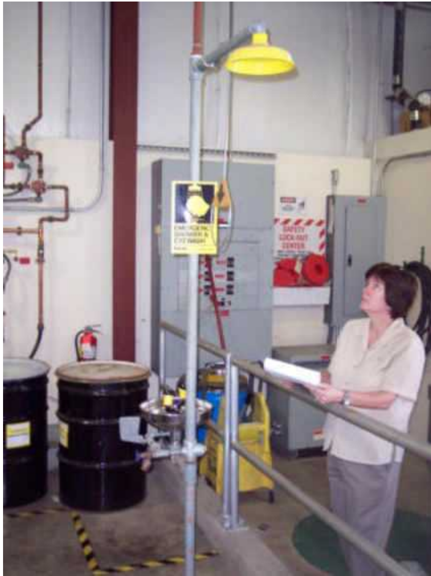
Grace Photo 7: Emergency Shower
