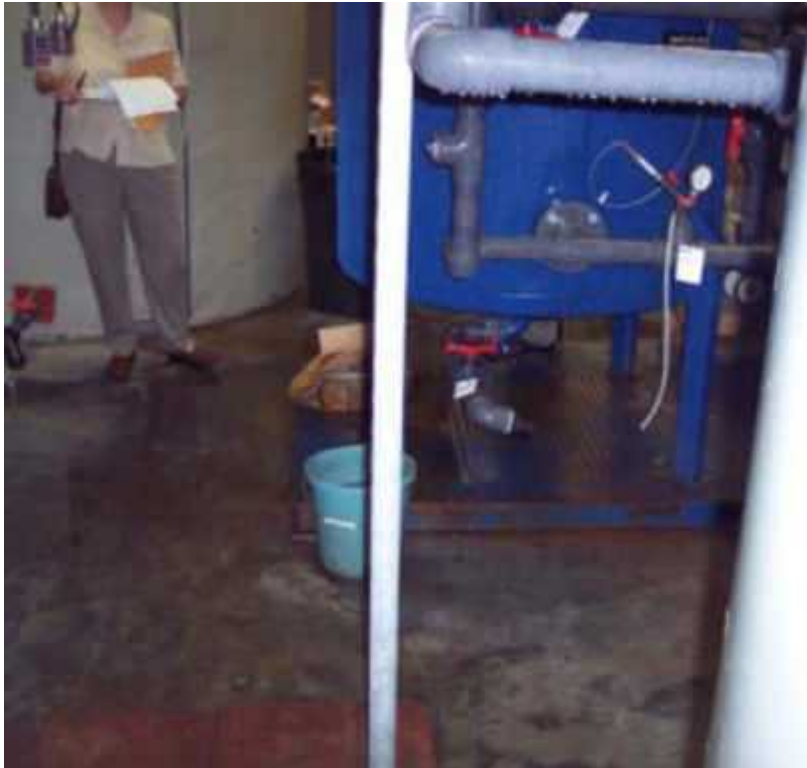
UniFirst Photo 12: Floor Area, note excess water on floor
