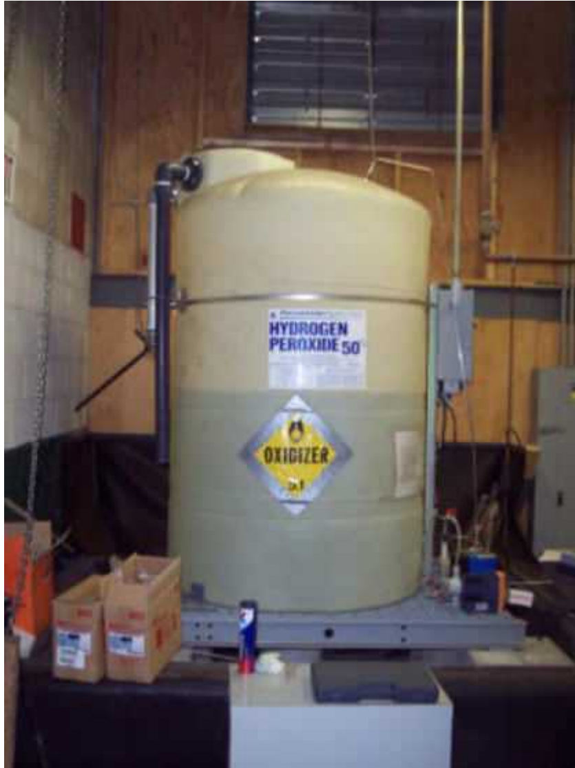
UniFirst Photo 4: No Longer Operational H 2 O 2 Tank
