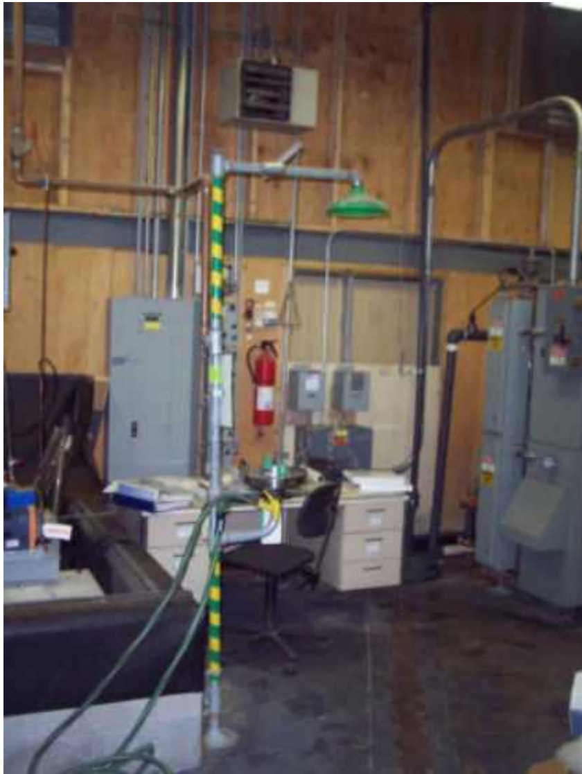
UniFirst Photo 5: Safety Showers - Boxes
