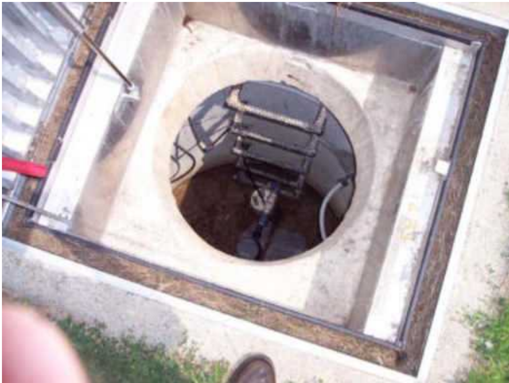
Grace Photo 15: Pumping Well RW 21, with Slight Sheen in Access Manhole
