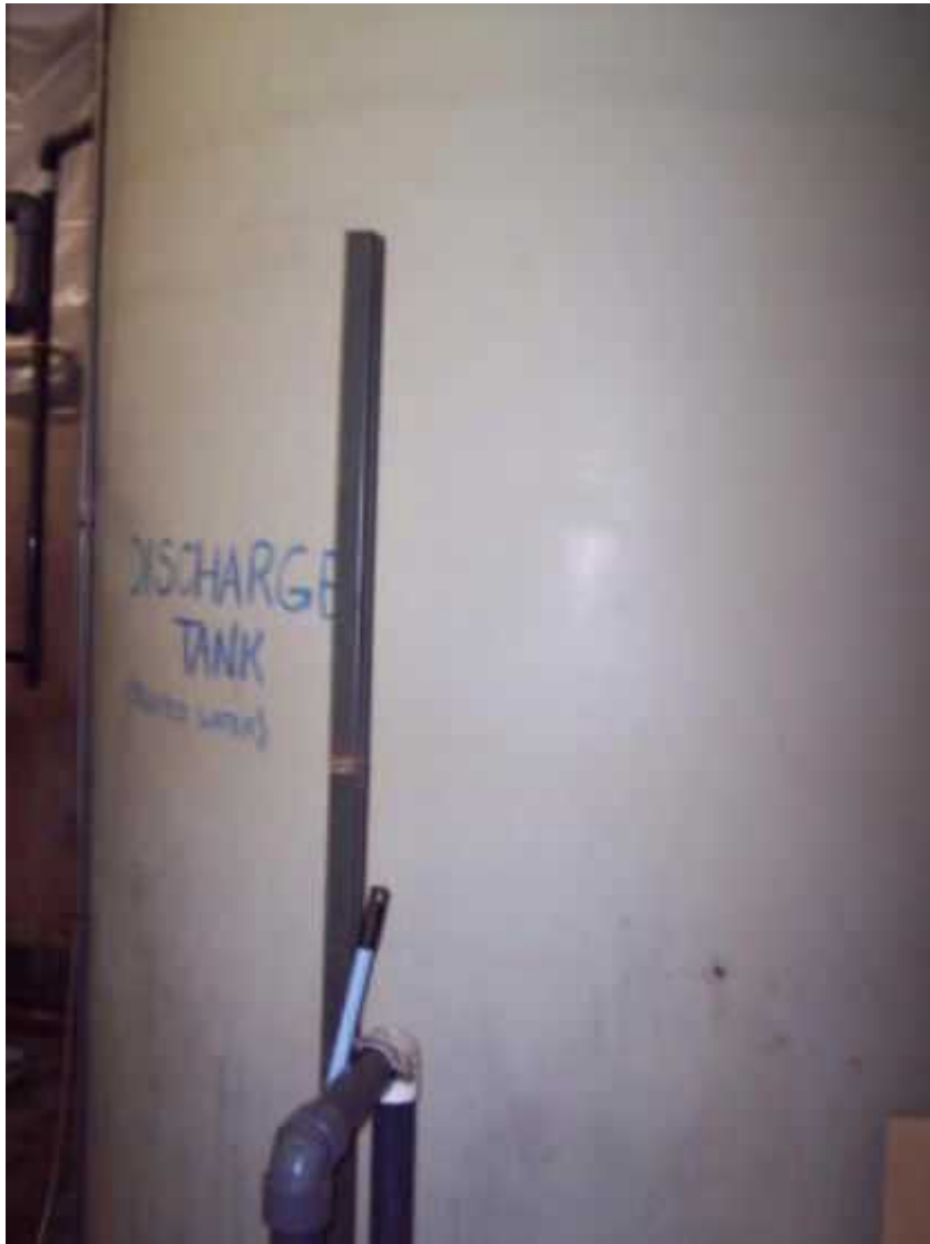
UniFirst Photo 9: Discharge Tank
