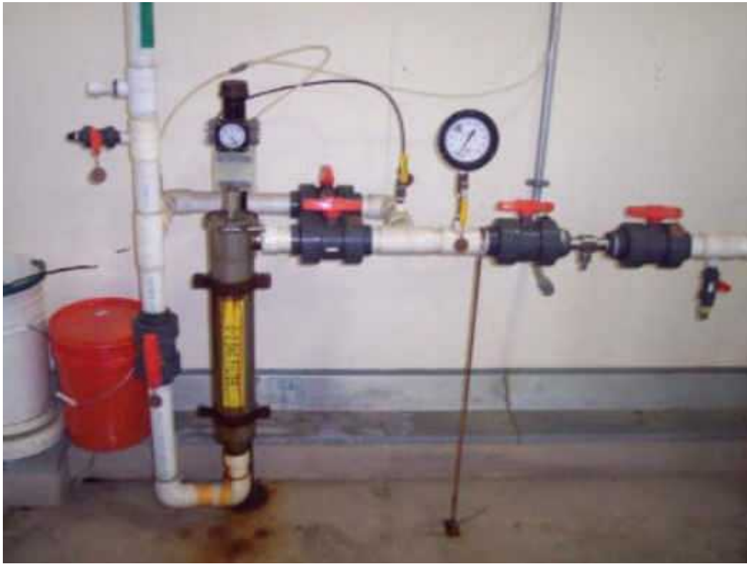
Grace Photo 3: Bag Filters and Pressure Gauges
