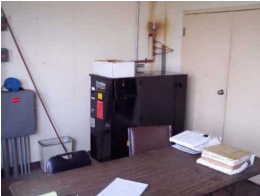
Grace Photo 12: Air Stream Oil/Water Separator
