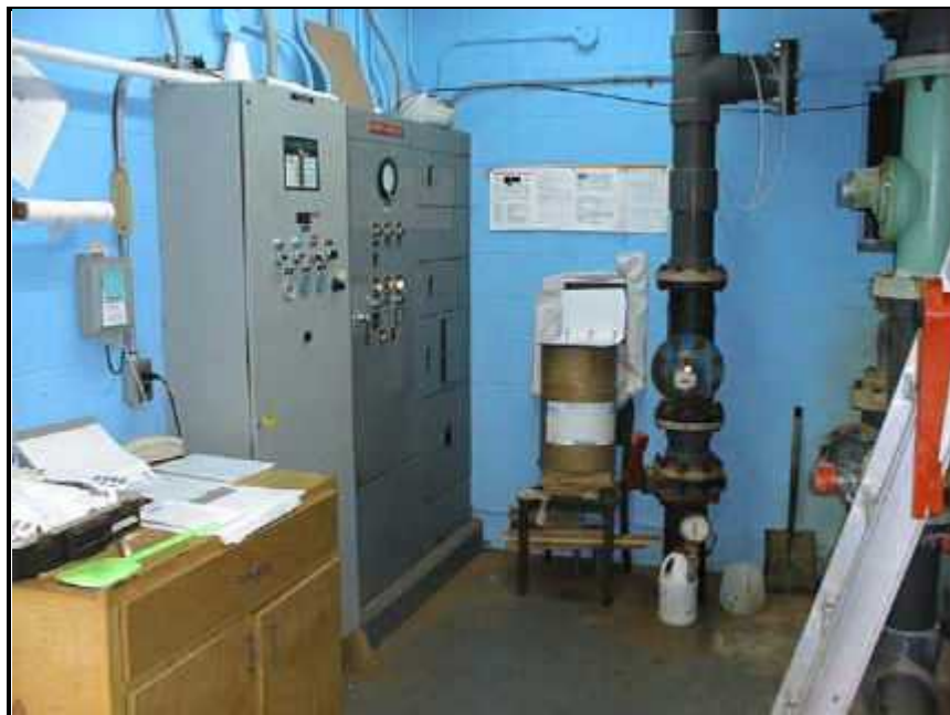
Photo 4: Inside Wyndmere Water Treatment Plant
