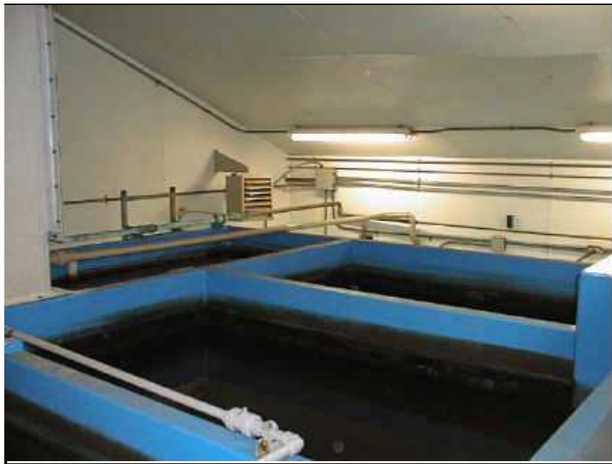
Photo 18: Lidgerwood Water Treatment Plant Filters
