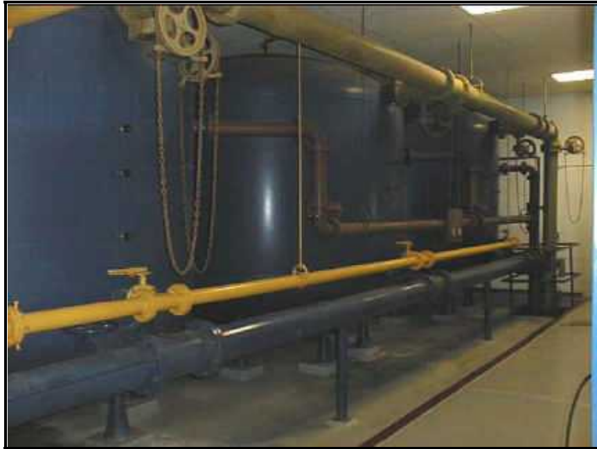
Photo 13: Water Treatment Plant Green Sand Filters, Southeast Water Rural Water System
