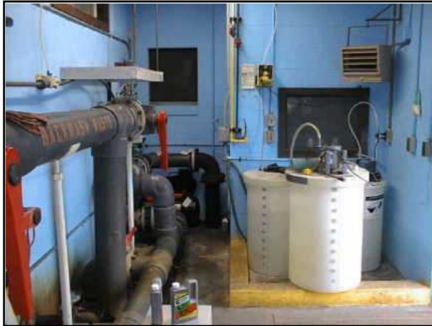
Photo 3: Inside Wyndmere Water Treatment Plant
