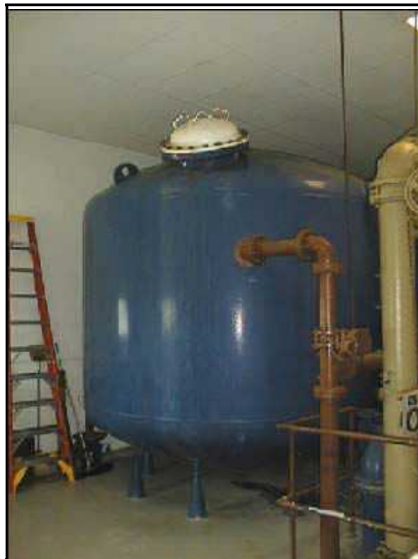
Photo 10: Water Treatment Plant Green Sands Filters, Southeast Water Rural Water System
