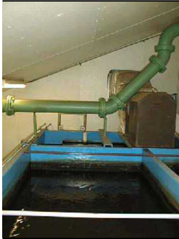
Photo 17: Lidgerwood Water Treatment Plant Filters
