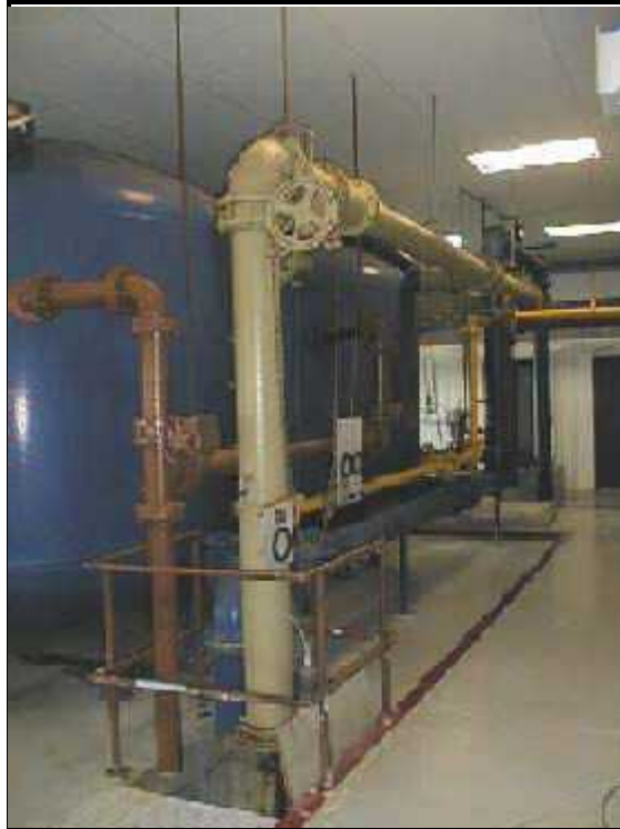
Photo 11: Water Treatment Plant Green Sand Filters, Southeast Water Rural Water System
