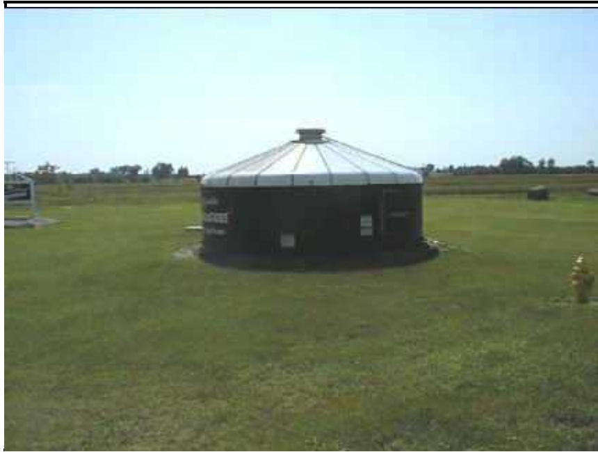
Photo 24: Lidgerwood Water Treatment Plant, Sludge Storage Tank
