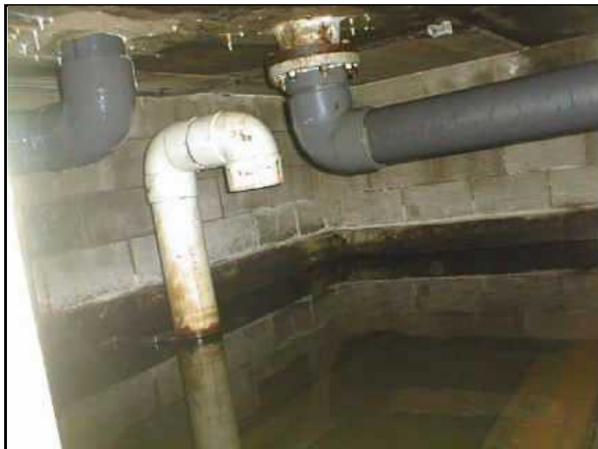
Photo 6: Wyndmere Water Treatment Plant-Filters
