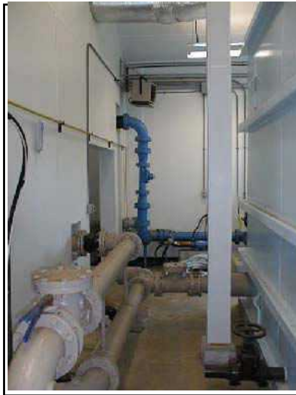
Photo 20: Lidgerwood Water Treatment Plant Contact Basins
