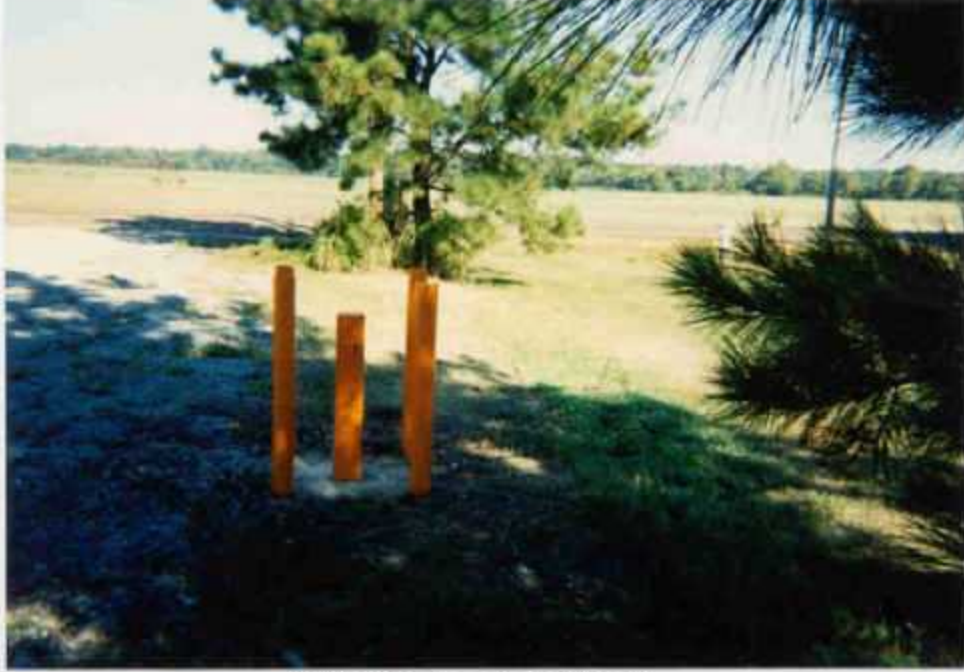
5) Monitoring Well OW-2A
