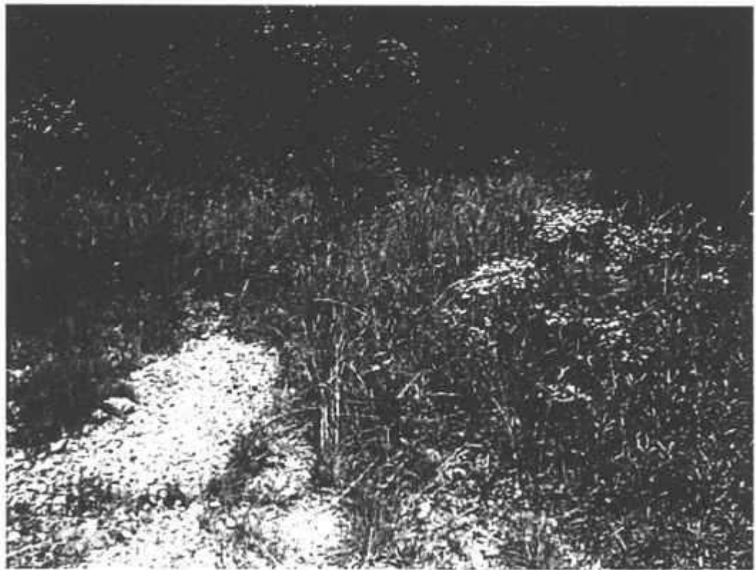
Photograph: Small area of surface erosion on eastern slope Project Name: Cedartown Municipal Landfill Superfund Site
