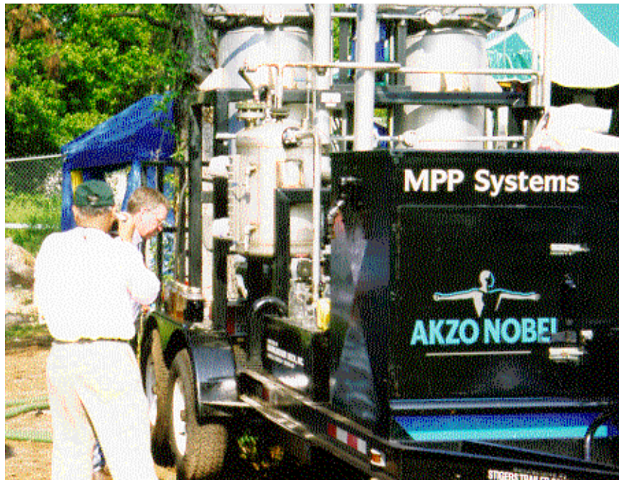
Trailer-mounted MPP system
