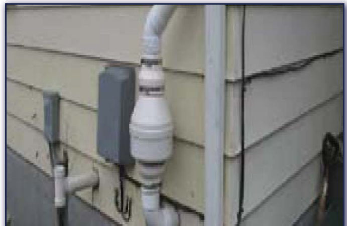
Fan Venting Soil Gas from Under Building to Outside Air
