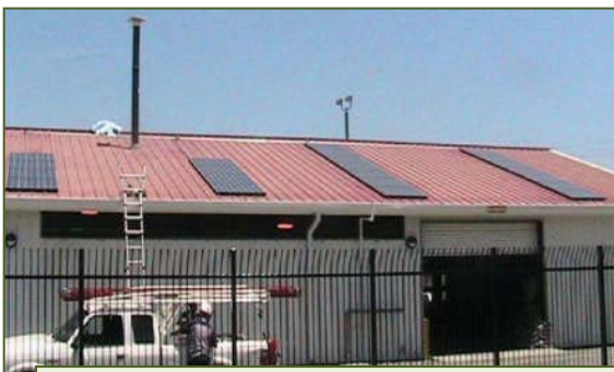
A photovoltaic system added to P&T operations at the Pemaco Superfund Site in Maywood, CA, contributes 5,900 kWh of electricity each year to high-vacuum dual-phase extraction of groundwater.
