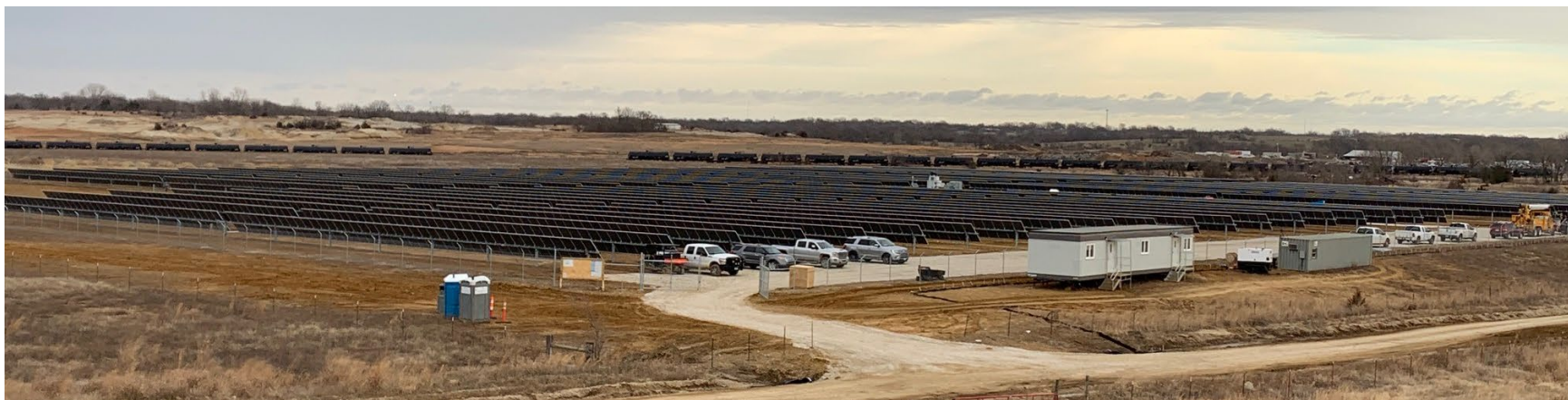
A solar farm at the Oronogo-Duenweg Mining Belt site in Missouri.
