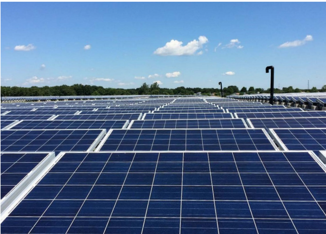
Figure 1: A solar farm at the Brick Township Landfill site (New Jersey).
