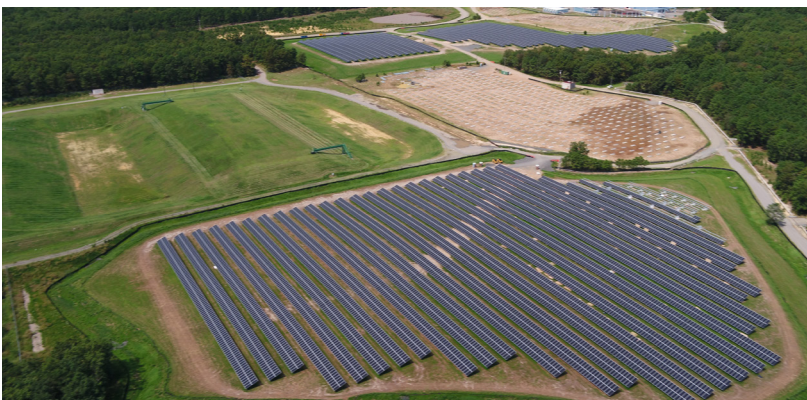
Figure 24. Aerial view of the solar array at the Ciba-Geigy site (New Jersey).
