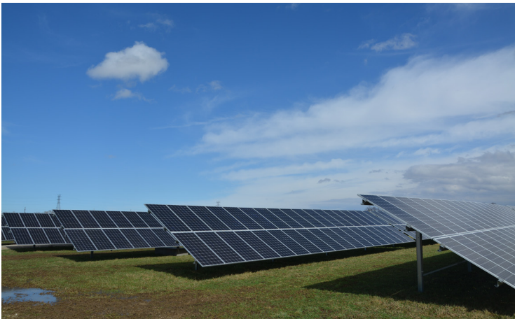
Figure 17. Maywood Solar Farm at the Reilly Tar & Chemical Corp. (Indianapolis Plant) Superfund site (Indiana, Region 5).
