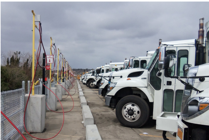
Figure 14. A compressed natural gas fueling station that fuels municipal sanitation trucks at the Syosset Landfill Superfund site (New York, Region 2).
