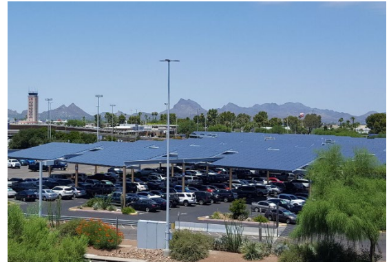
Fig. 10 Solar parking canopy. Source: Skeo Solutions.
