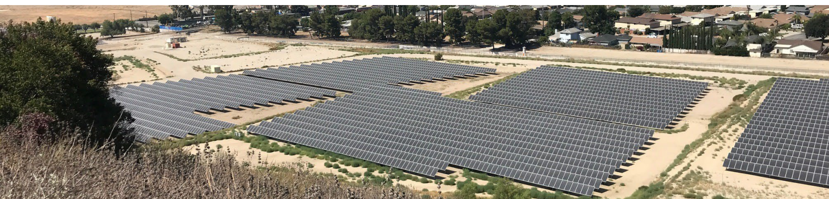
The 11,000-panel solar array at the Pacific Coast Pipeline Superfund site.
