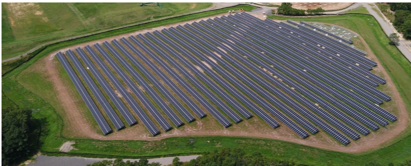
Solar panels at the capped Ciba-Geigy Corp. site.
