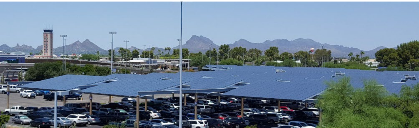
The solar canopies over the parking lot at Tucson International Airport.
