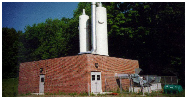
Figure 36. The groundwater treatment facility at the South Municipal Water Supply Well site.
