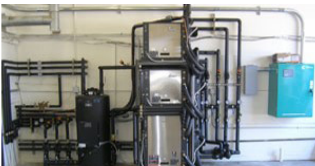
Figure 80. The geothermal heating and cooling system at the Arsenic Trioxide site.
